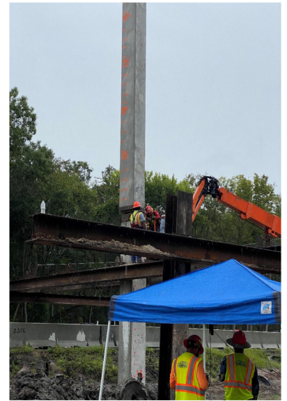
As part of a recent FDOT project, University of Central Florida researchers studied the impacts of pile-driving ground vibrations in various soils.
