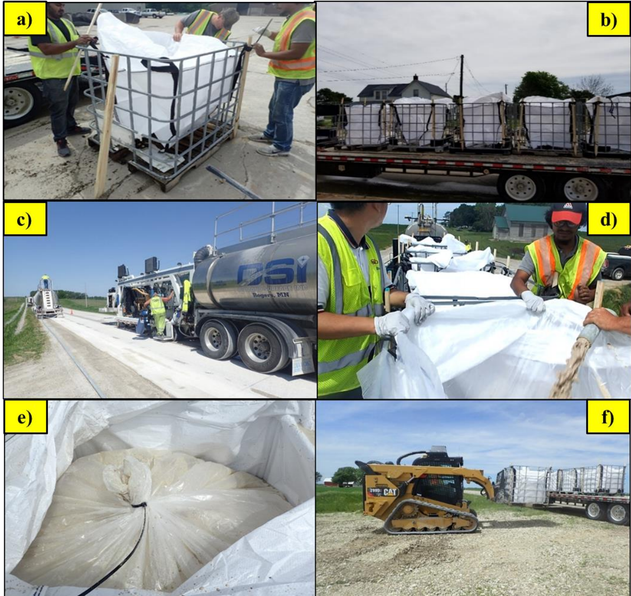
Figure 50. CGR collection at diamond grinding project site in Washington County: (a) preparing the super bags with containment, (b) transporting the super bags to the diamond grinding site, (c) diamond grinding operations, (d) filling the super bags with CGR, (e) securing the bags, and (f) transporting the bags to the construction site
