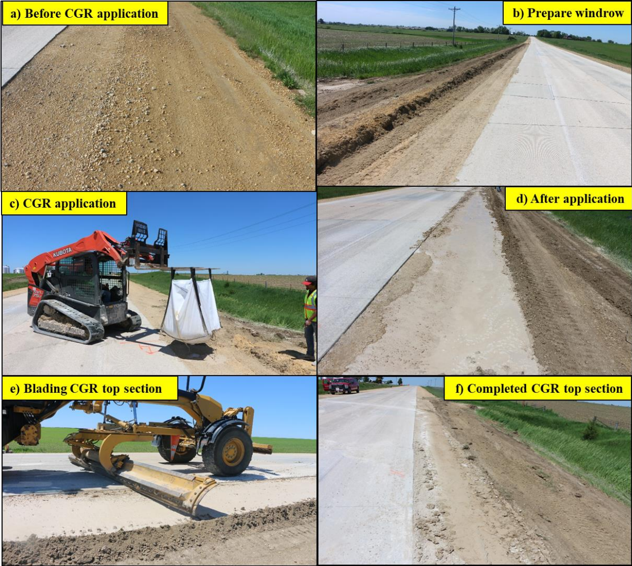
Figure 61. Construction of CGR Top section in Clinton County: (a) section appearance before CGR application, (b) creating windrow, (c) dumping CGR, (d) section appearance after CGR application, (e) blading CGR Top section, and (d) completed CGR Top section
