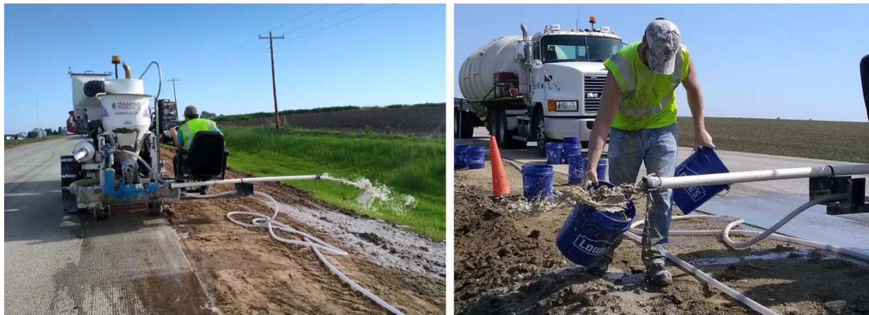
Figure 2. Direct discharge CGR collection (site CGR-3)
