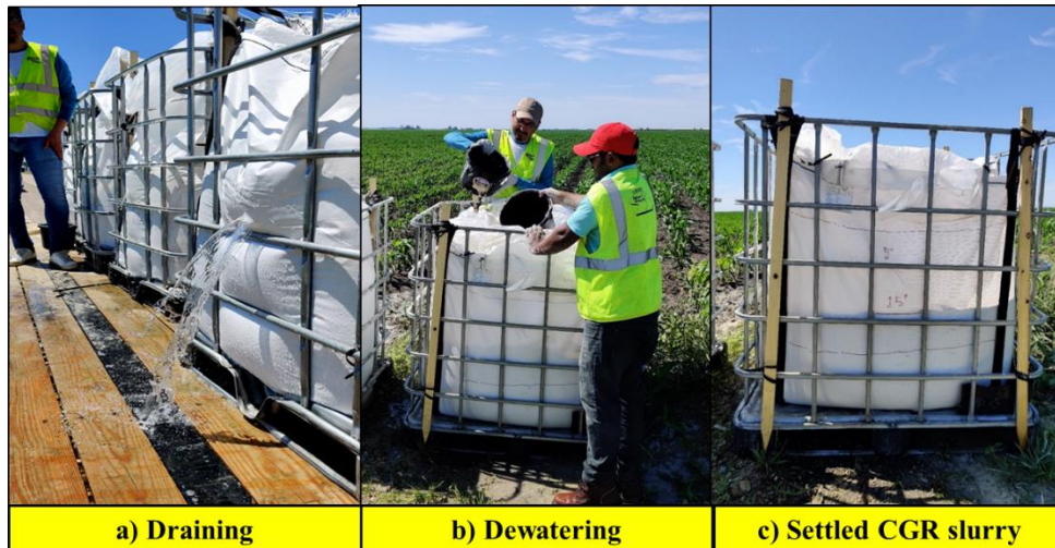
Figure 51. Dewatering process for CGR slurry at the demonstration site in Washington County: (a) draining water from bags, (b) manual dewatering, and (c) settled CGR slurry
