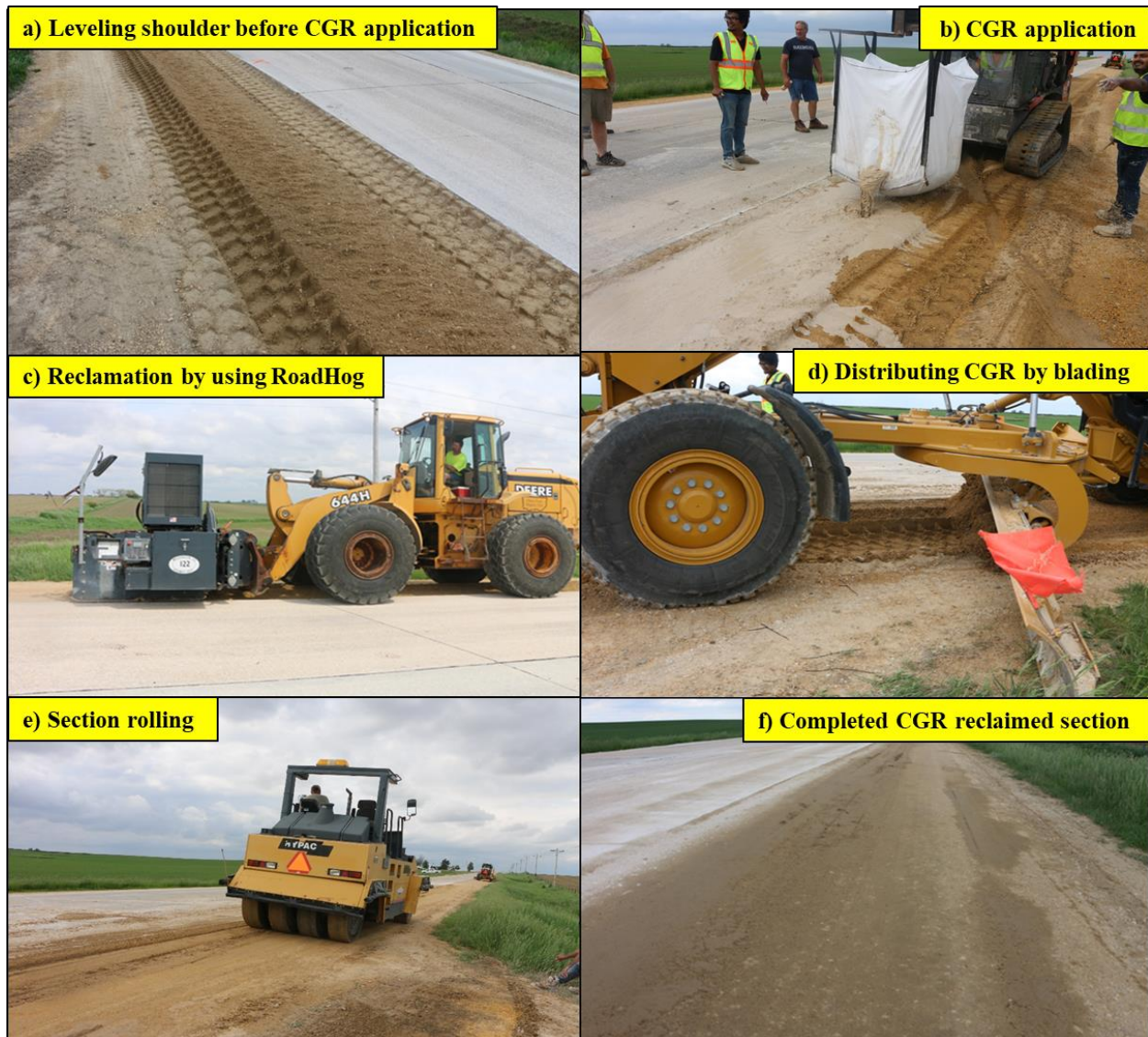
Figure 60. Construction of CGR Reclaimed section in Clinton County: (a) leveling site before CGR application, (b) dumping CGR, (c) reclaiming soil with CGR using a RoadHog, (d) distributing CGR by blading, (e) rolling compaction, and (f) completed CGR Reclaimed section
