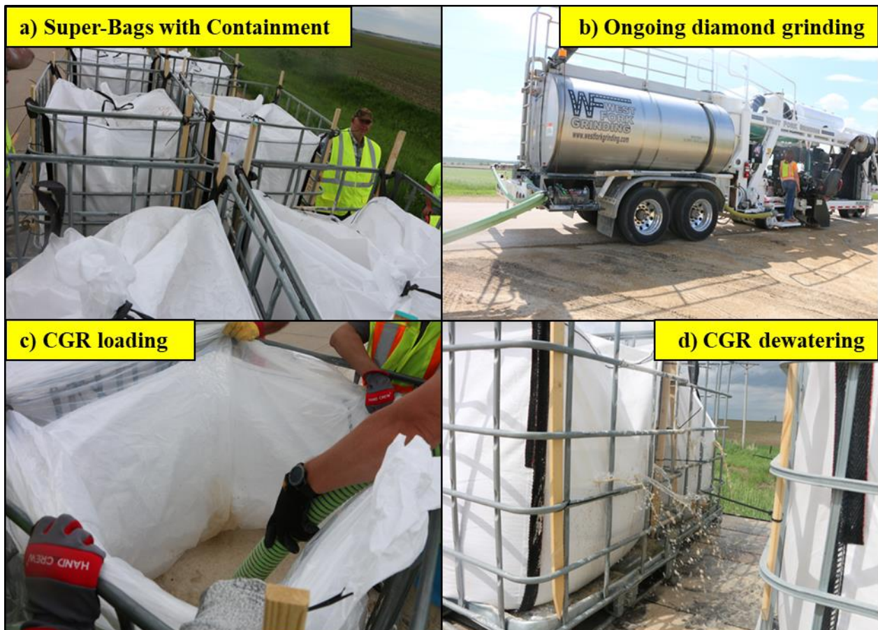
Figure 59. CGR collection at diamond grinding project site in Clinton County: (a) preparing the super bags with containment, (b) diamond grinding operations, (c) filling the super bags with CGR, and (d) dewatering the CGR bags
