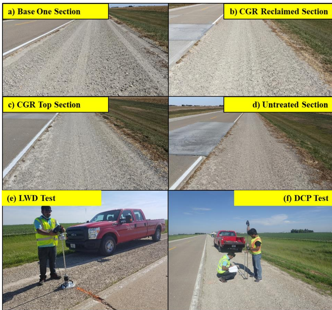
Figure 54. Washington County site appearance after two years: (a) Base One-treated section, (b) CGR Reclaimed section, (c) CGR Top section, (d) untreated section, (e) LWD testing, and (f) DCP testing
