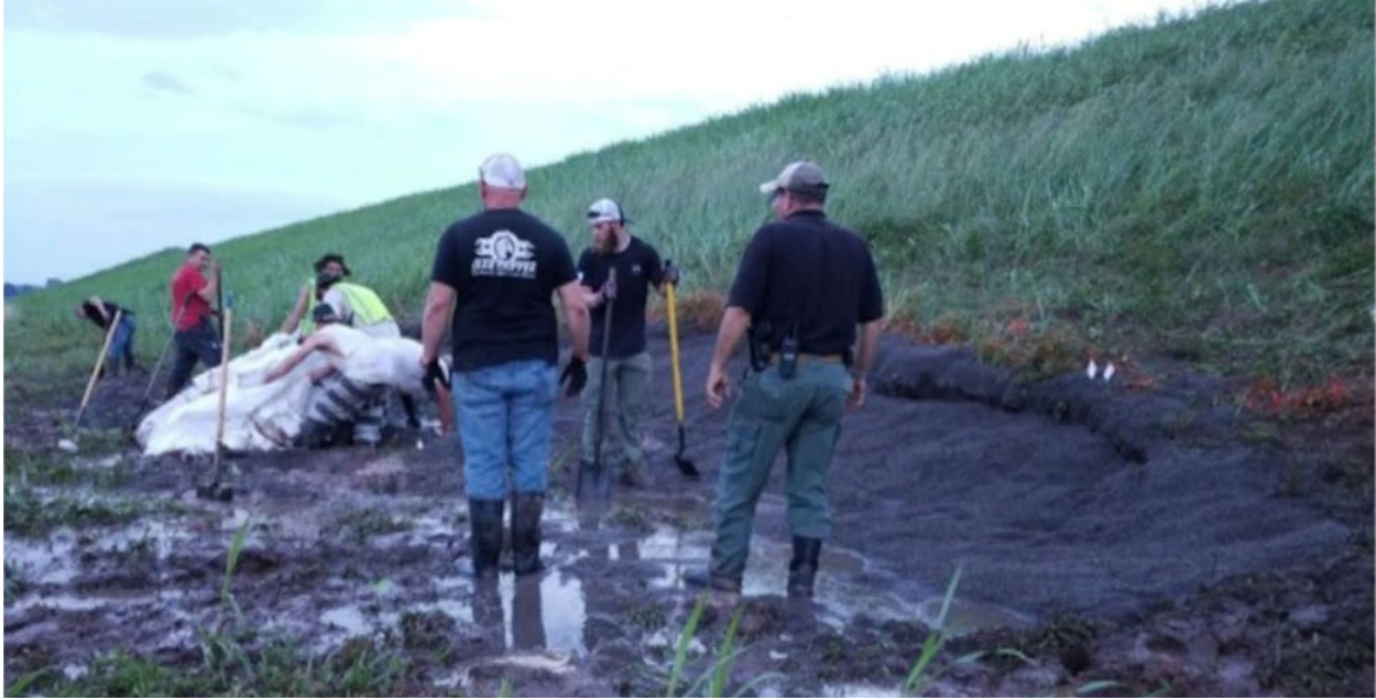
Figure 14 Placement of gravel at the base of the 2019 slide on June 25, 2019 (USACE, 2019)
