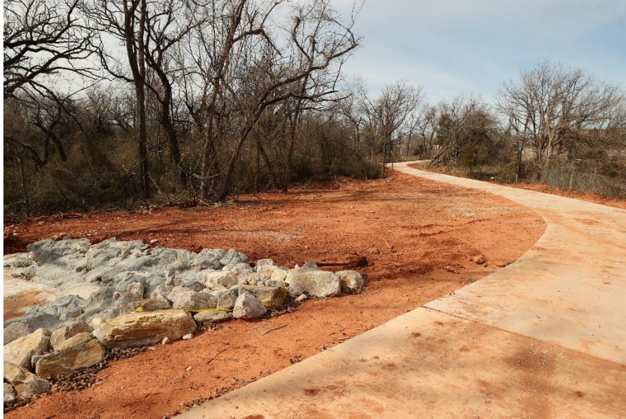
Figure 7: Oklahoma City is expanding active transport and access to park space with the construction of the Deep Fork Trail. (Source: Oklahoma City Planning Department)
