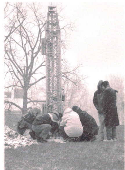
An FHWA team begins installing the new weather station. Once the station is up and running, it will gather data to support FHWA research on road weather management.
