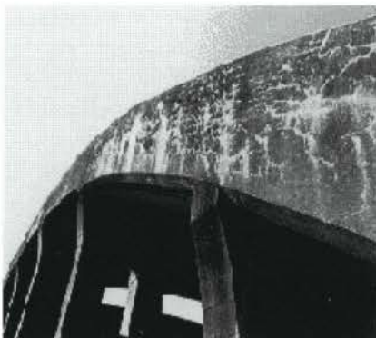
Damage from ASR gels limits the durability and performance of concrete structures such as that shown above.
