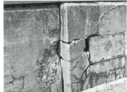
When alkalis and silica in concrete react, the result is gels that can swell and cause damaging cracks such as these.
