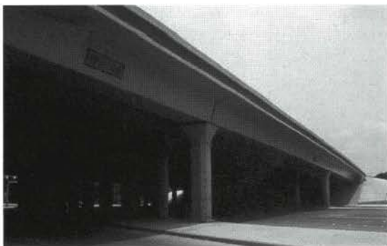
Participants at the recent annual meeting between FHWA and the National Concrete Bridge Council learned about new programs and technologies to improve concrete bridges, such as this one in Houston, TX.
