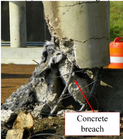
(b) Collision accident, Texas [25]
