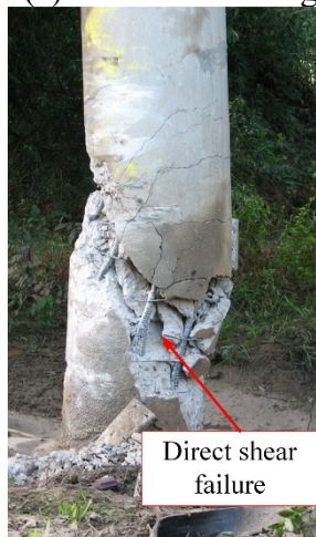
(b) Collision accident, Texas [5]
