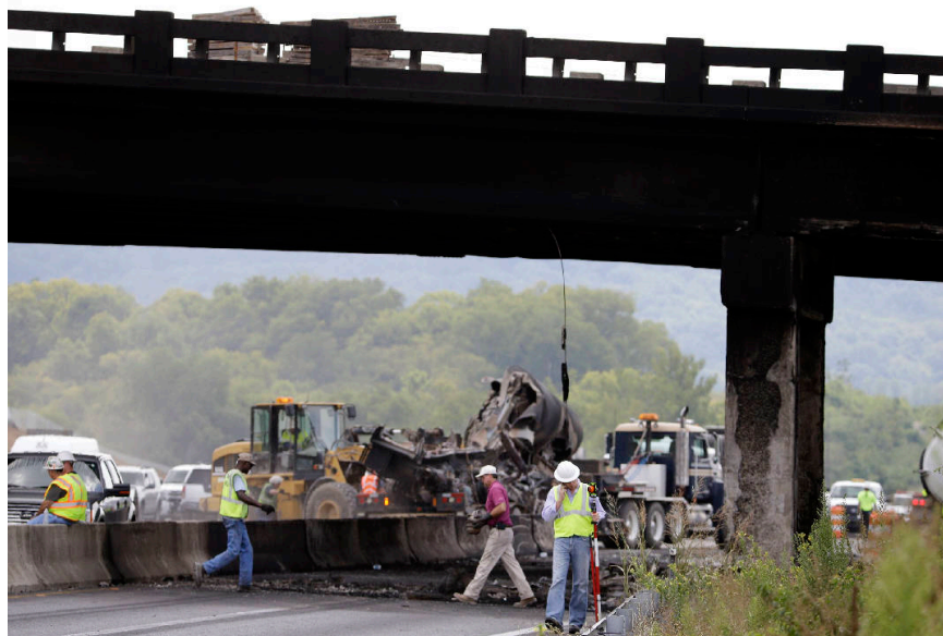
Figure 1.1 I-65 vehicle collision and explosion [1]
