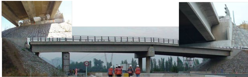
(c) Las Mercedes bridge and girder unseating at abutments, Chile
