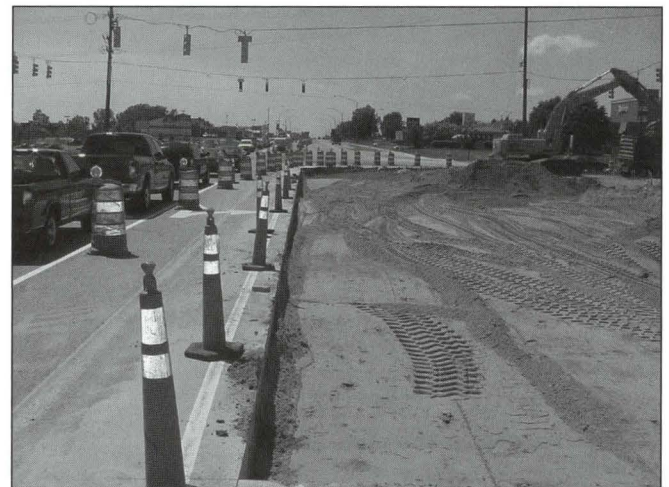
This photo shows the reconstruction of the 28th Street at Broadmoor Avenue intersection in Grand Rapids and Kentwood, Michigan.
