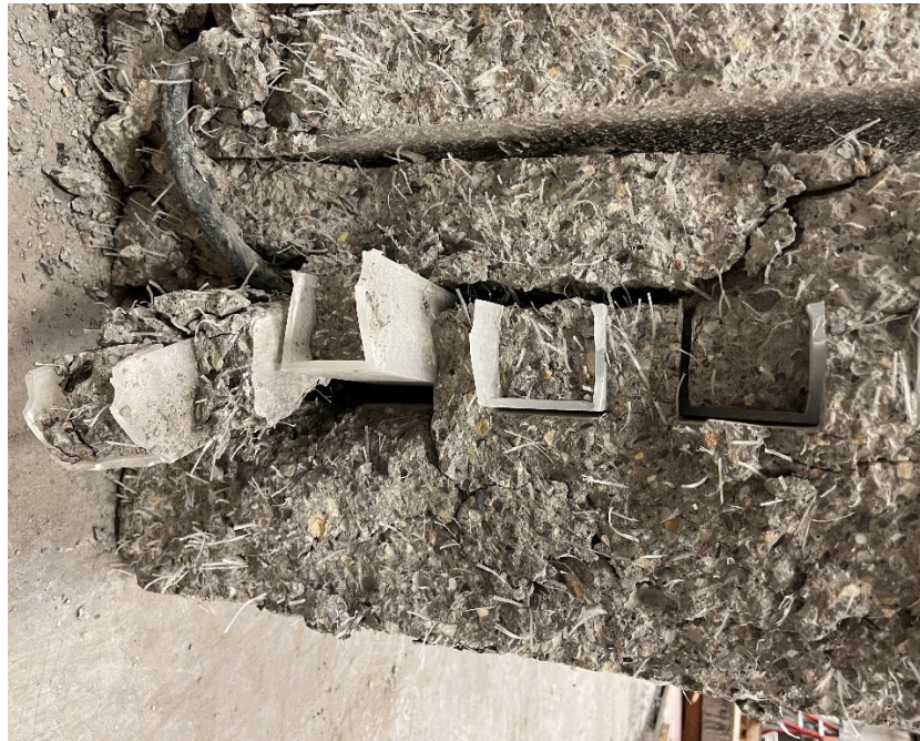
Figure 5.22 FRC Slab Exposed Failure Plane
