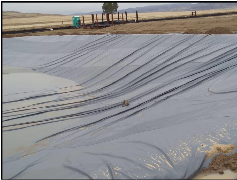
Figure 7. San Joaquin kit fox in a water containment basin on the Panoche Solar Farm construction site.
