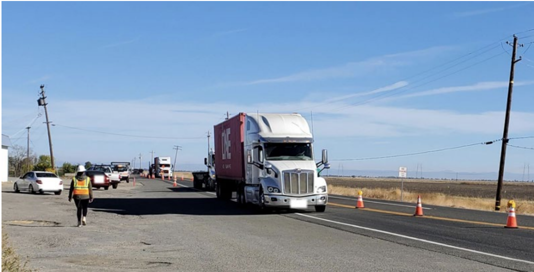
Figure 5.28 Two Heavy Vehicles Intruding into the Work Zone near Flagger Location 1
