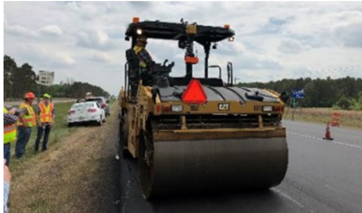
Figure 2.16 Work Zone Equipment Vehicle Used for AWARE System Testing in Minneapolis
