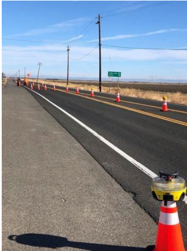
Figure 5.24 Placement of Intellicone PSA near Shoulder of the Work Zone
