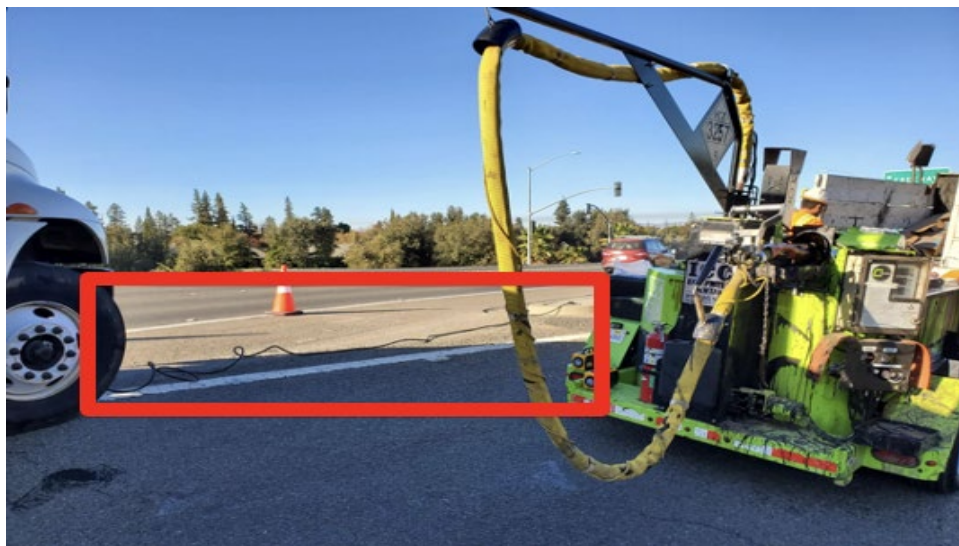
Figure 5.43 Location of Second WAS Hose Deployment
