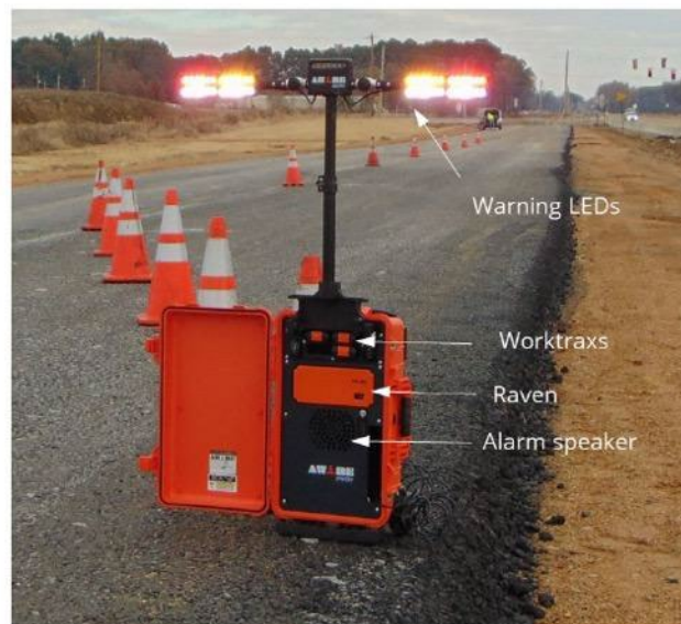
Figure 2.11 AWARE Sentry System Components (Source: CRH Inc. Video Team, 2021)
