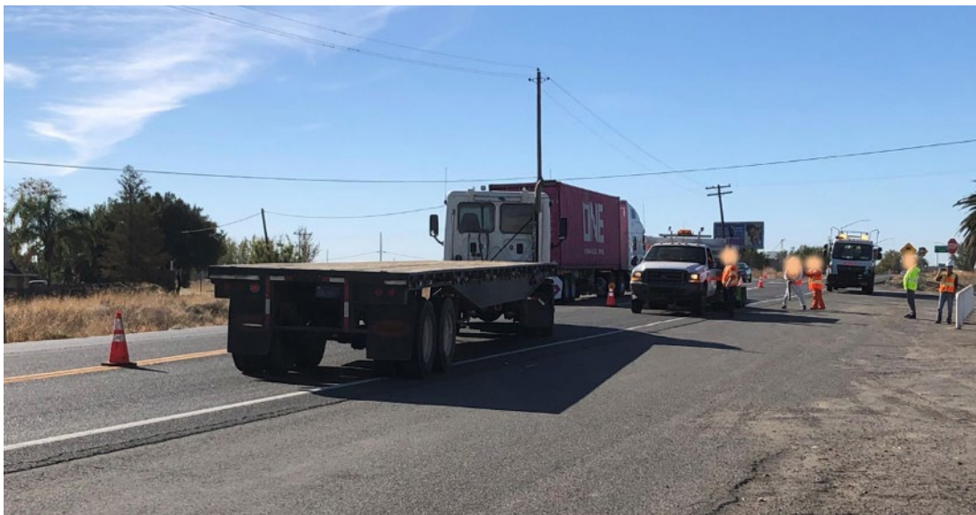
Figure 5.29 Two Heavy Vehicles Exiting the Work Zone After Intrusion
