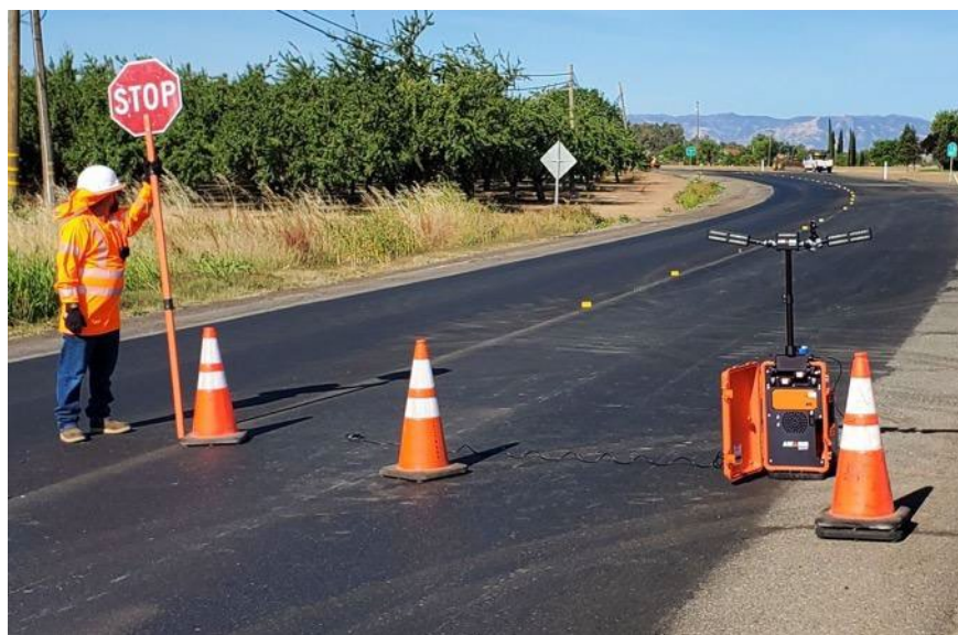
Figure 5.14 AWARE Sentry Deployment at Flagger Location on Highway 16 near Woodland, CA
