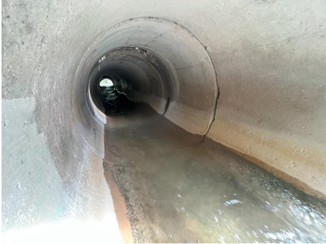
Photo of Sugarhouse Concrete pipe where the spall was measured.
