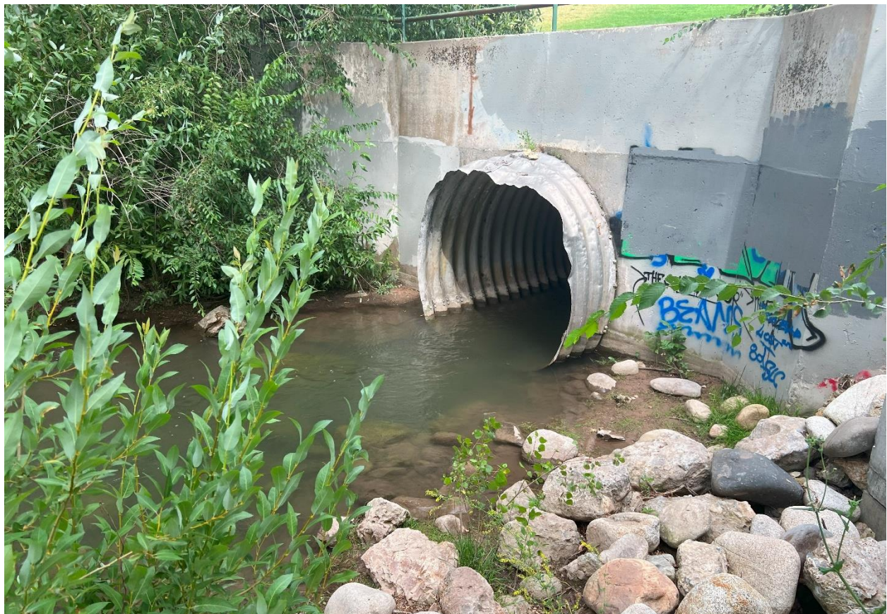
Figure 3.11.1 – Sugarhouse Park, Hidden Grove Pipe
