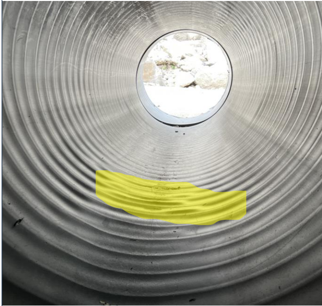
Photo with Localized Buckling Highlighted
