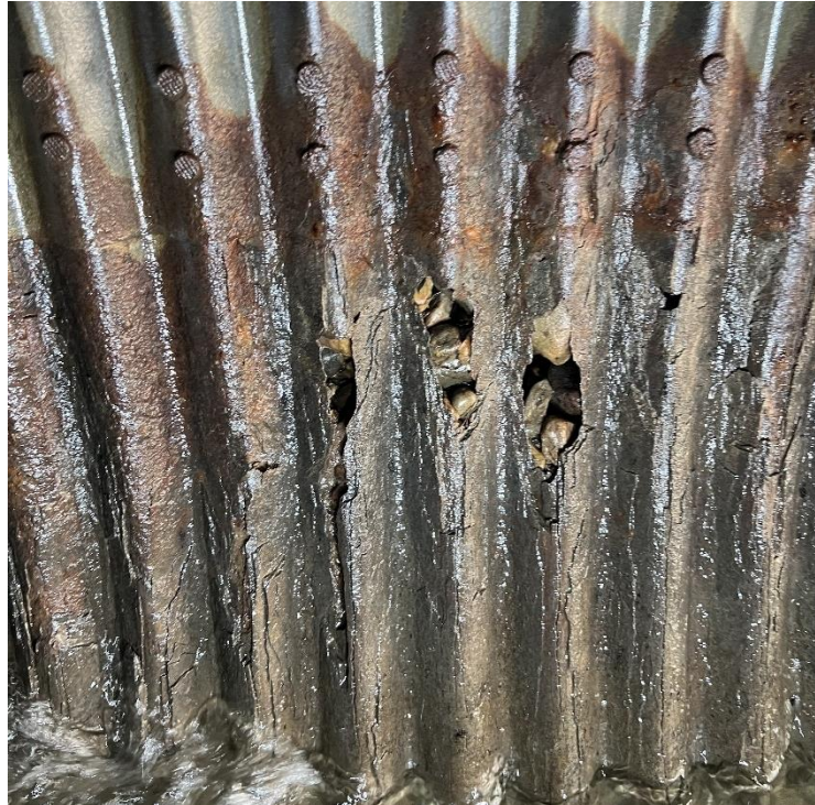
Photo of Corrosion Damage
