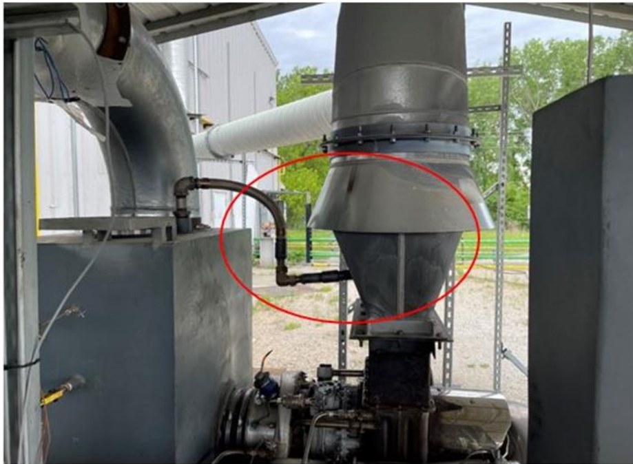
Figure K- 4. Alison 250 C28B turbine engine (exhaust shunt circled in red)
