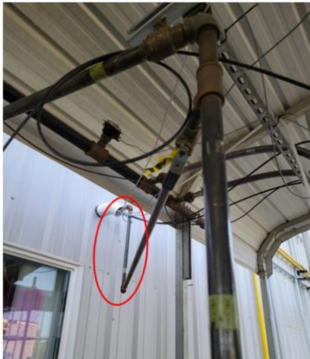
Figure 15. Bleed air sample line from engine to building
