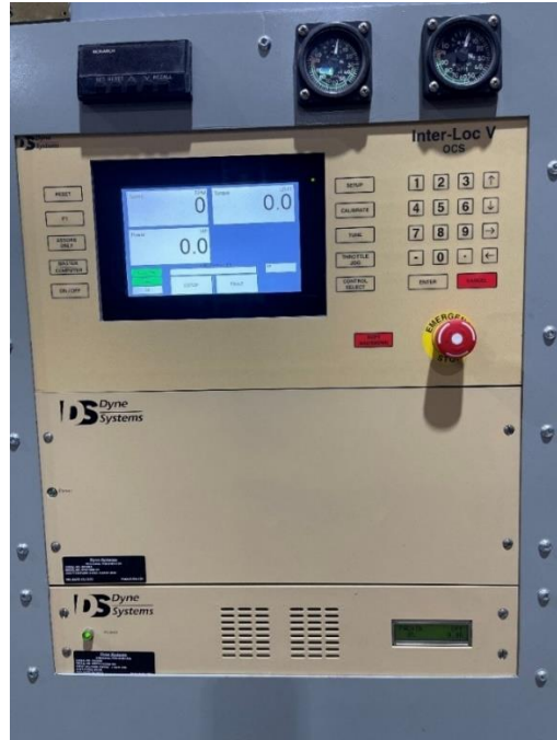
Figure 3. Engine and dynamometer control panels
