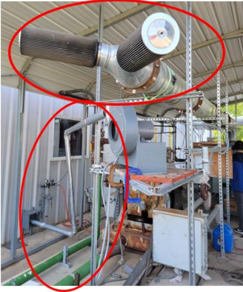
Figure 5. Dual inlet air filters (upper red circle) and inlet air sample (enclosed within lower left circle)
