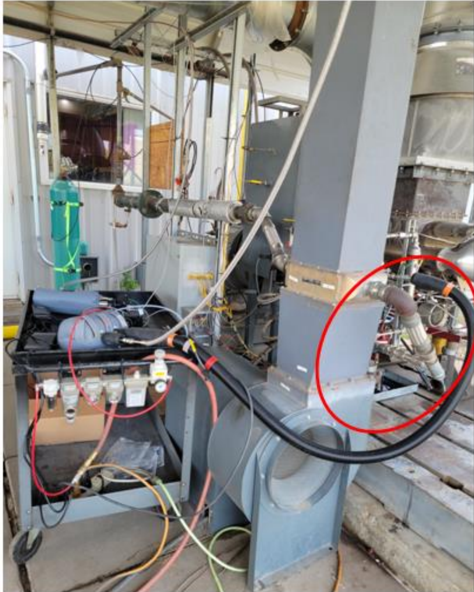
Figure 13. Flex line from engine bleed valve to heat exchanger and heat exchanger blower
