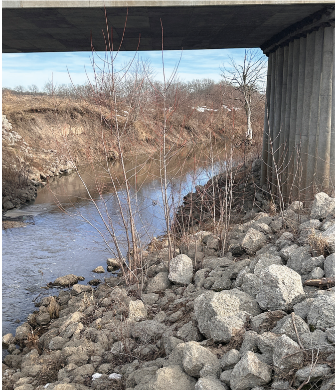
Partially grouted revetment at a Wayne County site after five years in service
