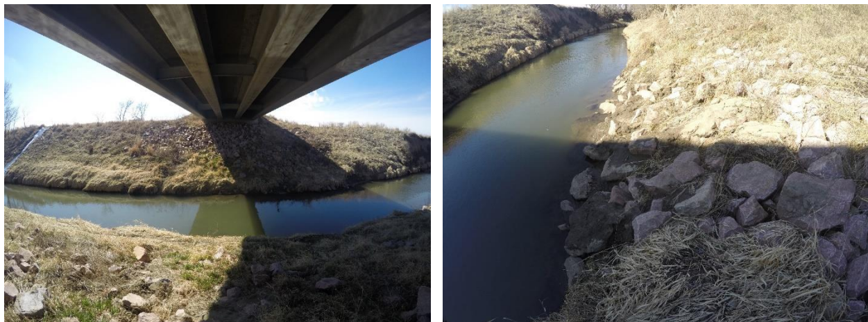
Figure 20. Undersized loose riprap in Woodbury County, Iowa
