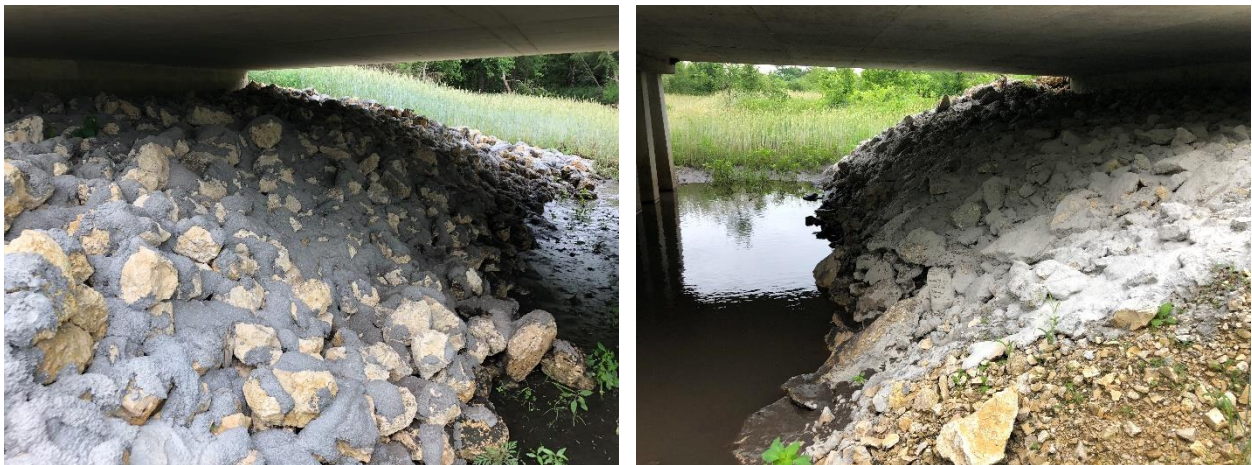
Figure 36. Condition shortly after placement for Bridge 1 (left) and Bridge 2 (right) in Buchanan County
