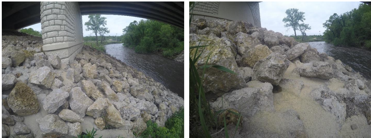
Figure 18. Minnesota Site 3: Partially grouted riprap—thin grout
