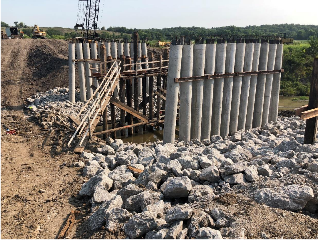
Figure 40. Wayne County pilot installation site
