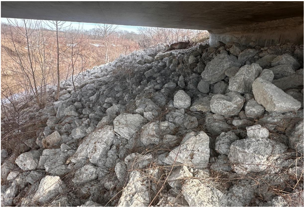
Figure 47. Wayne County Pilot installation as of February 2024
