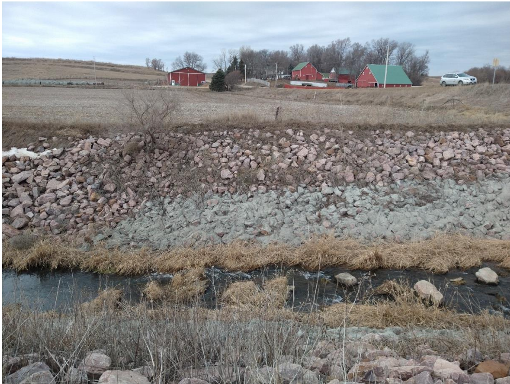
Figure 48. Woodbury County Pilot installation as of February 2024
