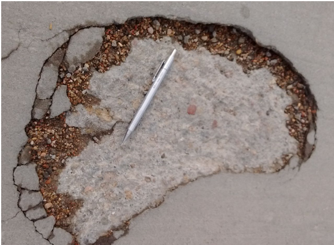
Figure 3.16: Typical Medium Spall
