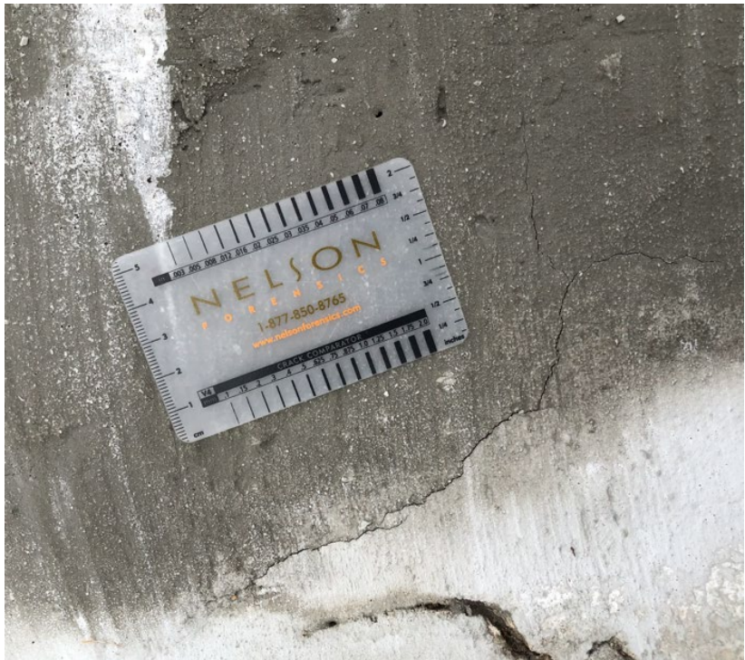
Figure 3.27: Plastic Shrinkage Crack on Surface of Layer 2
