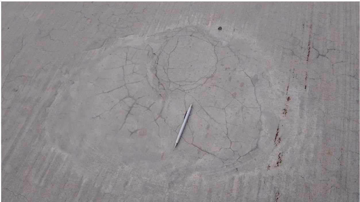
Figure 3.14: Typical Preliminary Delamination with Map Cracking
