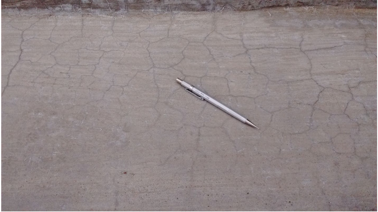
Figure 3.12: Typical Map Cracking of JMM Overlay
