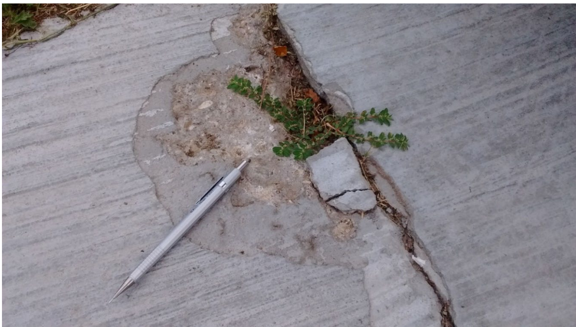
Figure 3.2: Small Isolated Spall Near Reflected Joint on Sidewalk Showing Underlying Thickness of Each Bonded Layer
