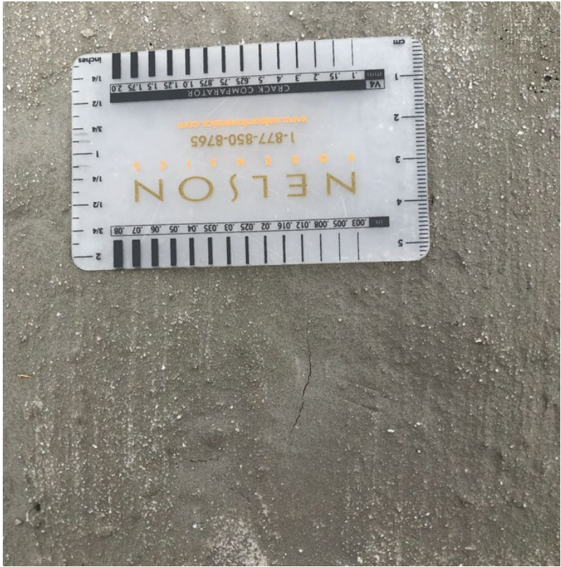
Figure 3.26: Plastic Shrinkage Crack on Surface of Layer 2
