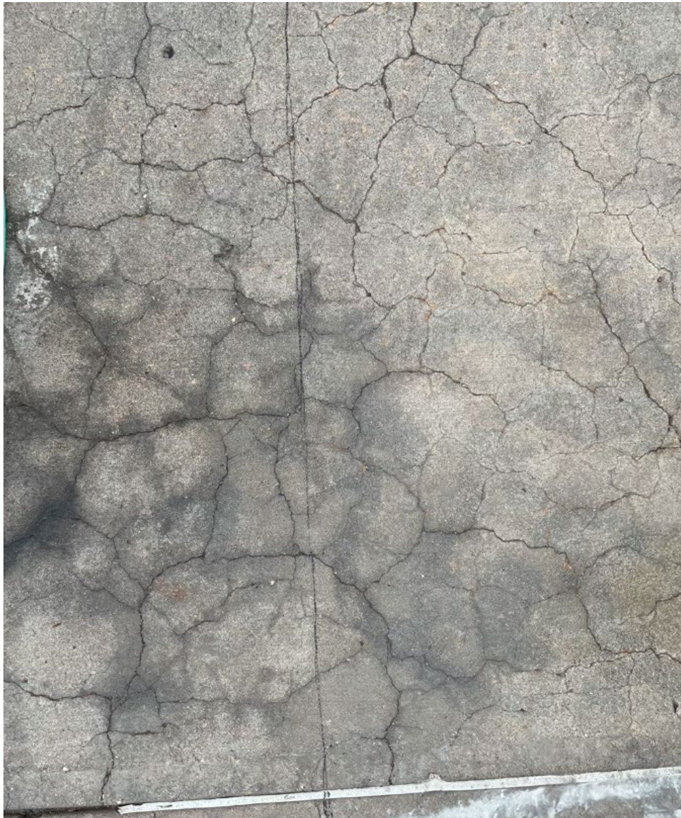
Figure 3.17: Map Cracking of Concrete Substrate Prior to Overlay Placement
