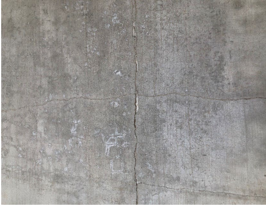
Figure 3.6: Map Cracking and Reflective Cracking Over Underlying Joints of Sidewalk
