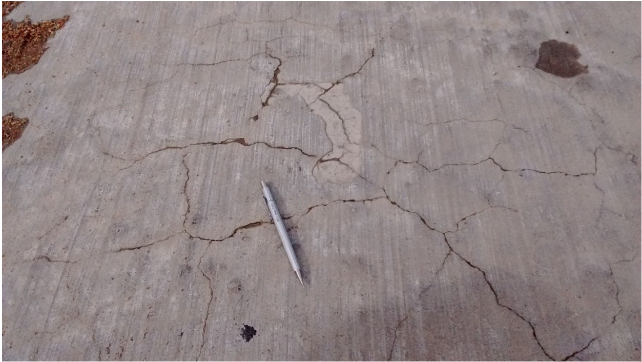
Figure 3.13: Typical Isolated Large Pattern Map Cracking
