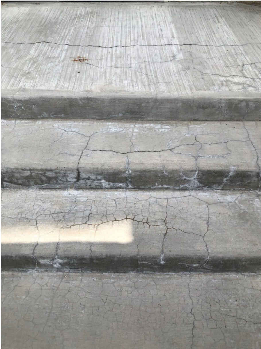
Figure 3.9: Typical Map Cracking with Efflorescence
