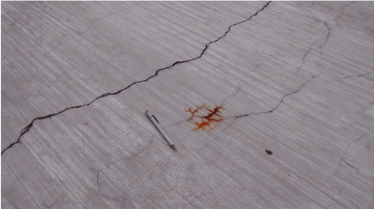
Figure 3.11: Rust Staining Coming Up Through Map Cracks
