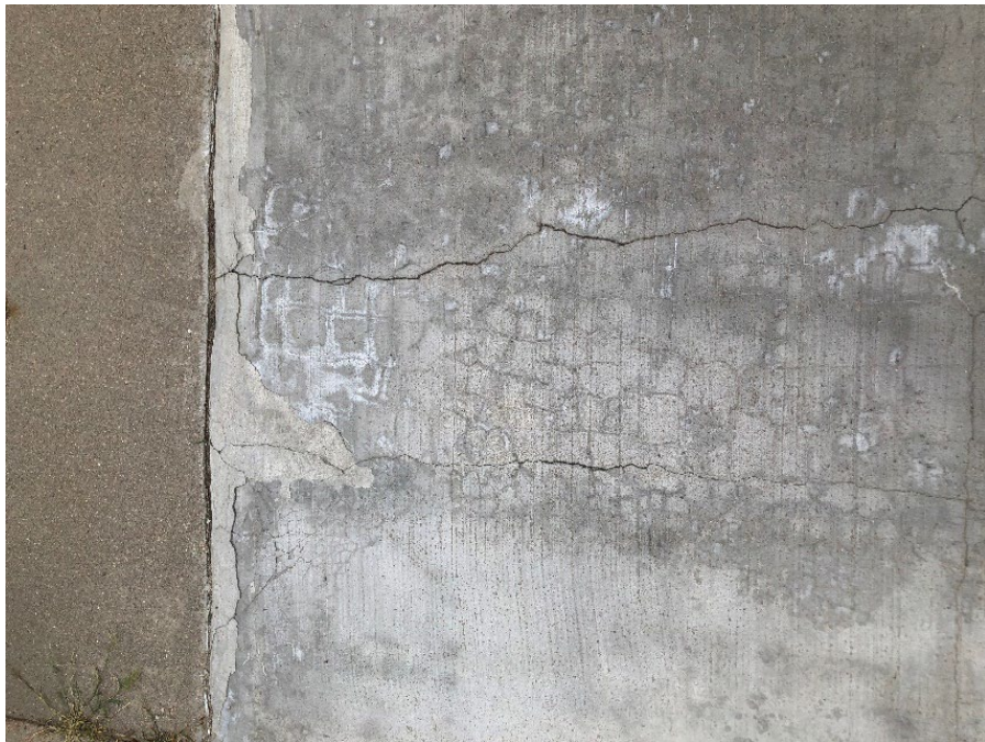
Figure 3.7: Map Cracking, Longitudinal Cracking, and Isolated Spalling Near Joint of Sidewalk
