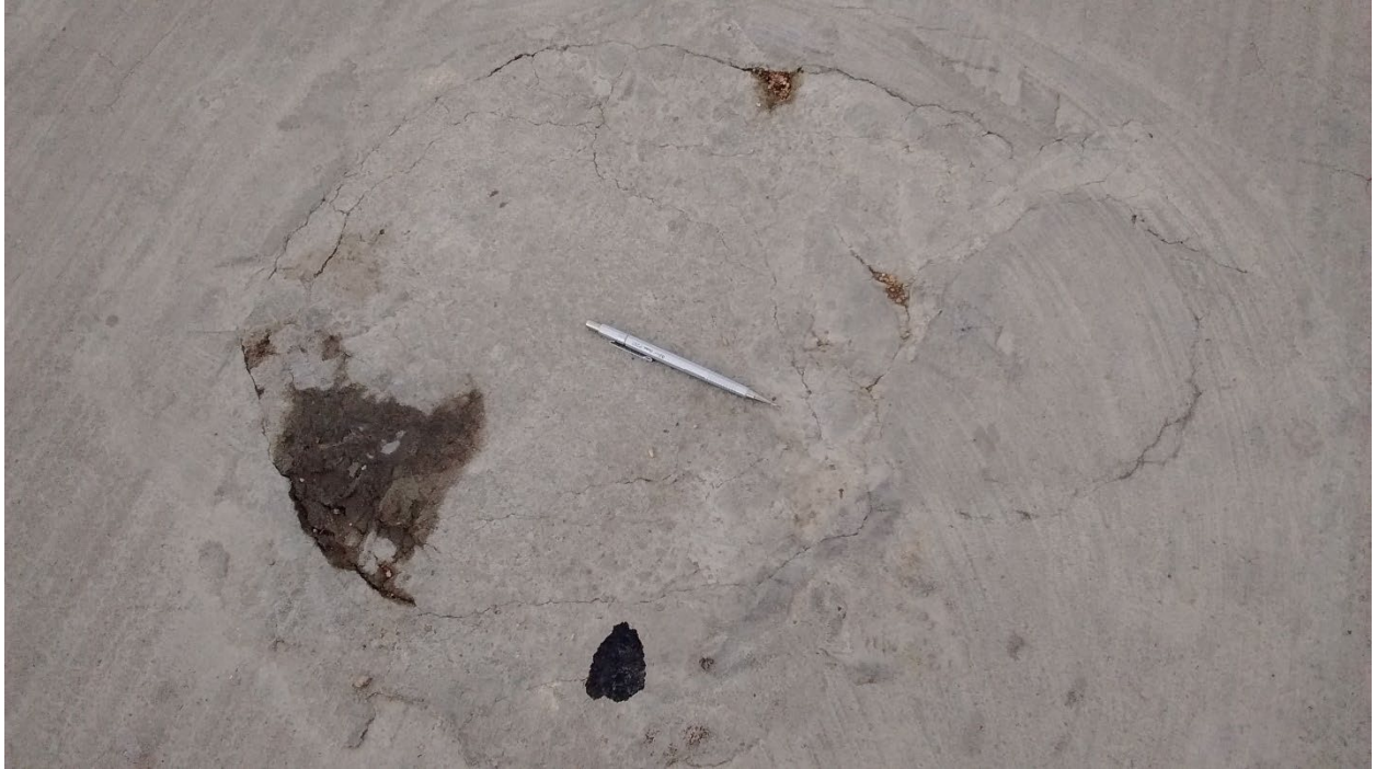
Figure 3.15: Typical Preliminary Medium Delamination with Pending Spall
