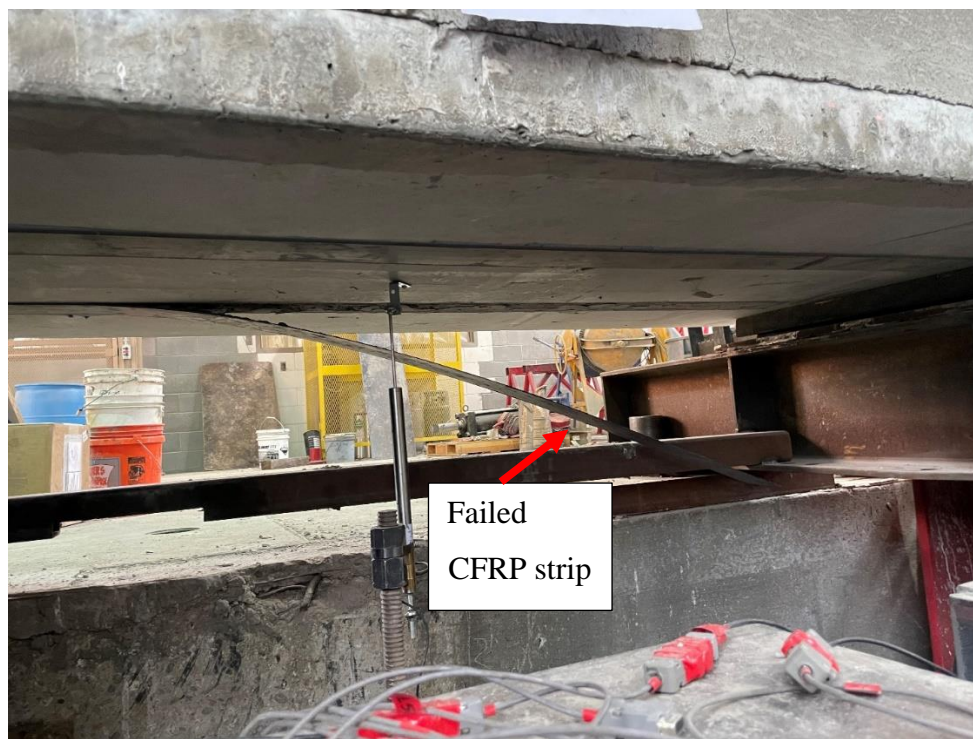
Figure 5.20 East CFRP bond failure at applied displacement of 2.4 in.
