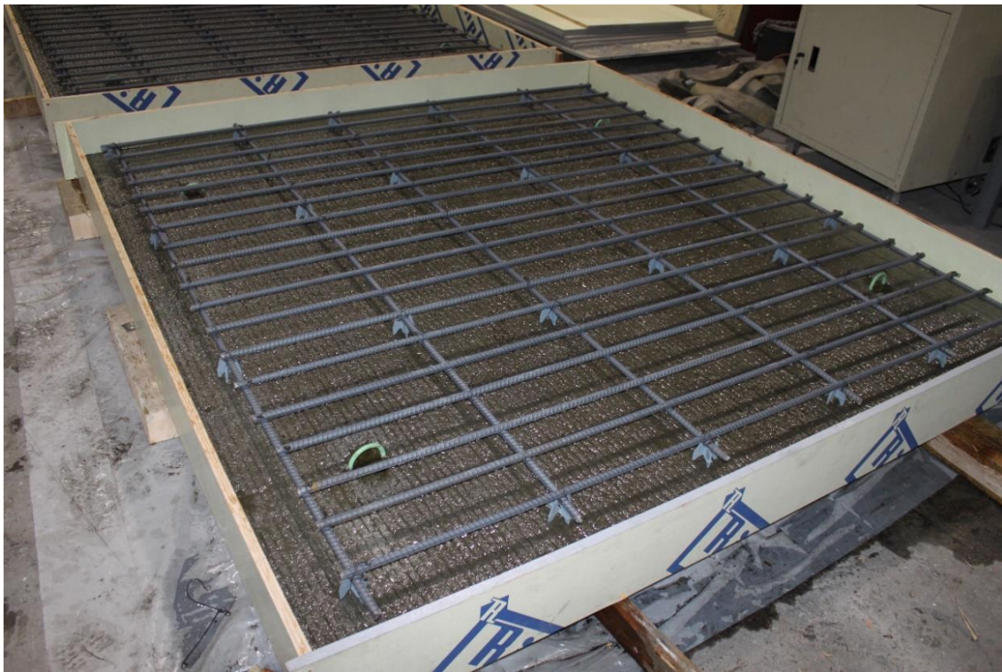
Figure 2.2 CIP section ready for casting with vegetable oil applied to the precast surface.
