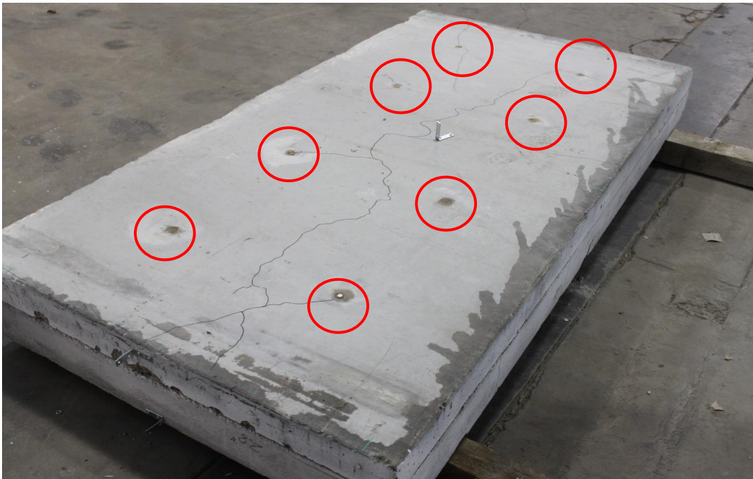
Figure 5.26 Test panel with nonproprietary anchor retrofit. The test panel is inverted, the red circles indicate the locations of the anchors.
