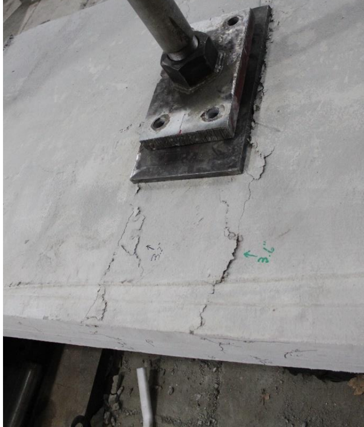
Figure 5.14 Shear anchor retrofit deck panel compressive failure after applied displacement of 3.6 in. (Location: top, mid-span)
