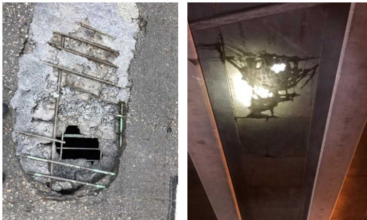
Figure 1.1 Blow-through of deck panel at I-15 and 800 South bridge (credit: UDOT)
