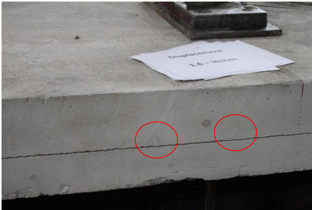
Figure 5.24 Flexural cracks at 1.6 in. of displacement.
