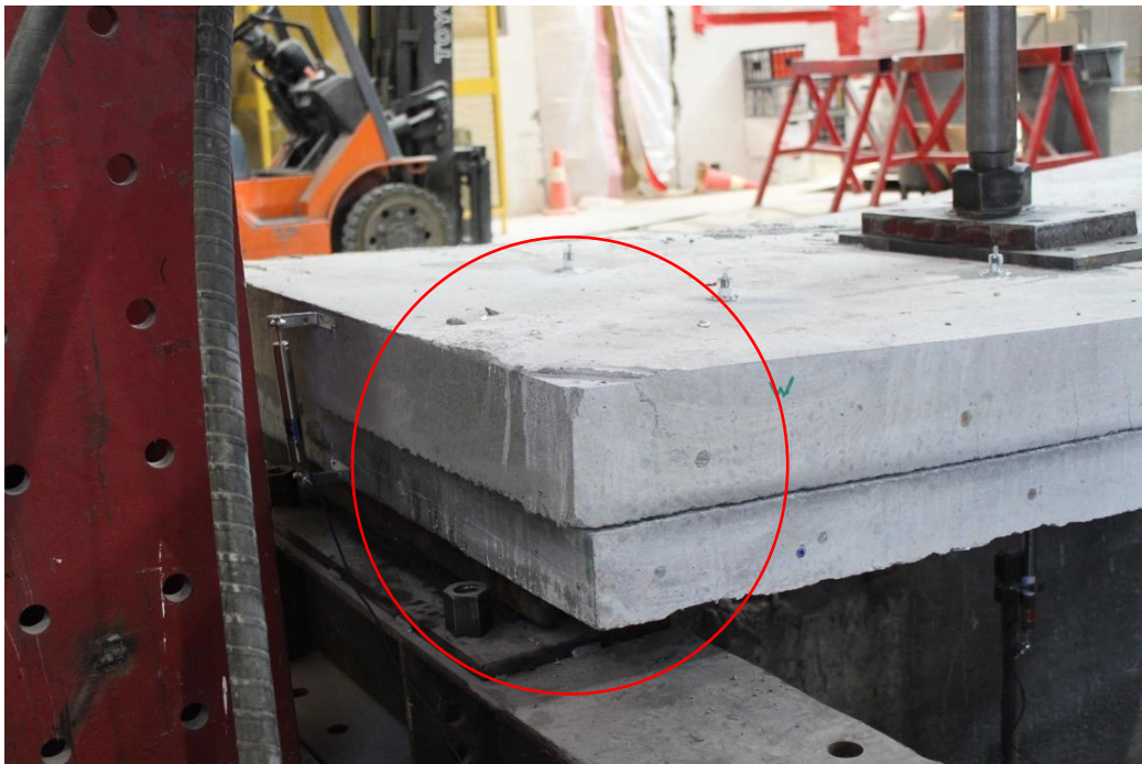
Figure 5.10 Lateral movement of epoxy retrofit deck panel at applied displacement of 4.0 in. (Location: northwest)
