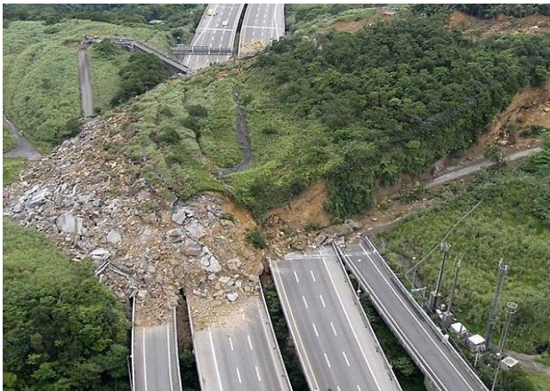
(c) Sudden, natural. Landslide damage of Freeway 3, 2010, Keelung City, Taiwan . (Source: D. Petley, blogs.agu.org/landslideblog )
