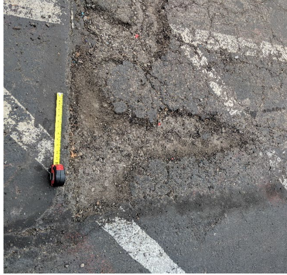
Figure 2.8 Scanned pothole with a tape measure providing one foot as a reference
