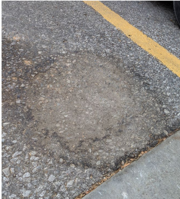
Figure 2.10 The second scanned pothole
