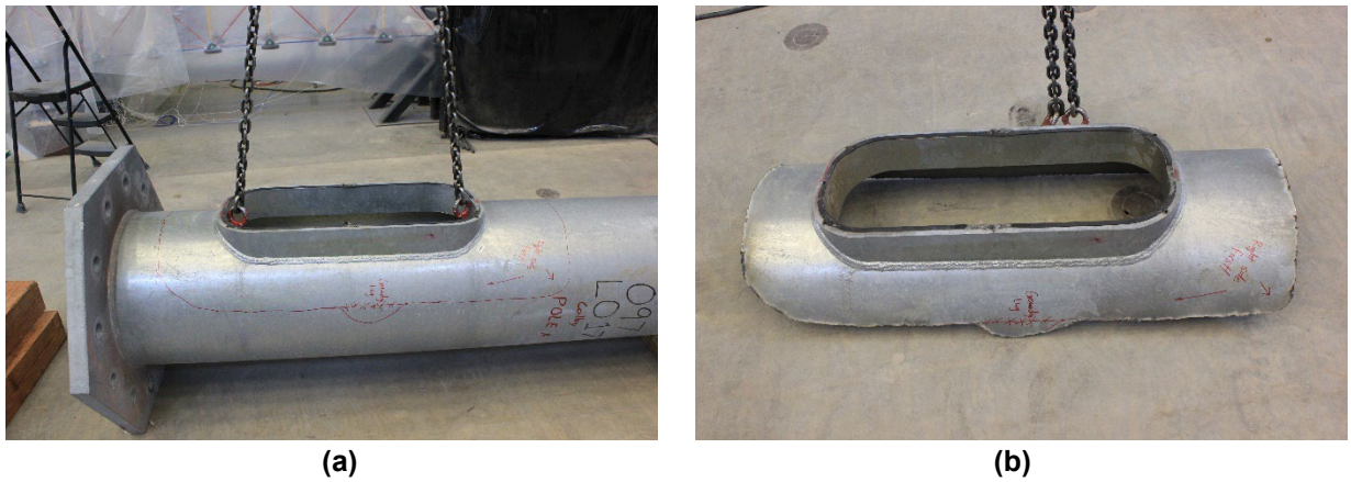
Figure 2.5: The Supports Used for (a) Plasma Cutting Poles A and C and (b) the Handhole Removed from Pole A
