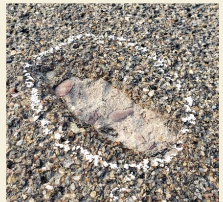
Figure 4: Close-up photograph of a small pop-out spall in the HFST on Bridge 1367 in 2020.
