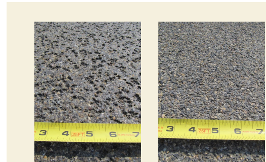
Figure 3: Close-up photographs of (a) the wheel path and (b) the shoulder of the HFST on Bridge 1367 in the Missoula District in 2022.
