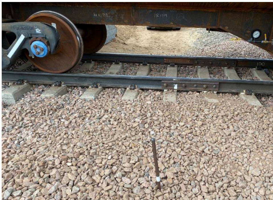
Figure 23. Fixed Measurement Point used to Assess Track Shift After the Impact
