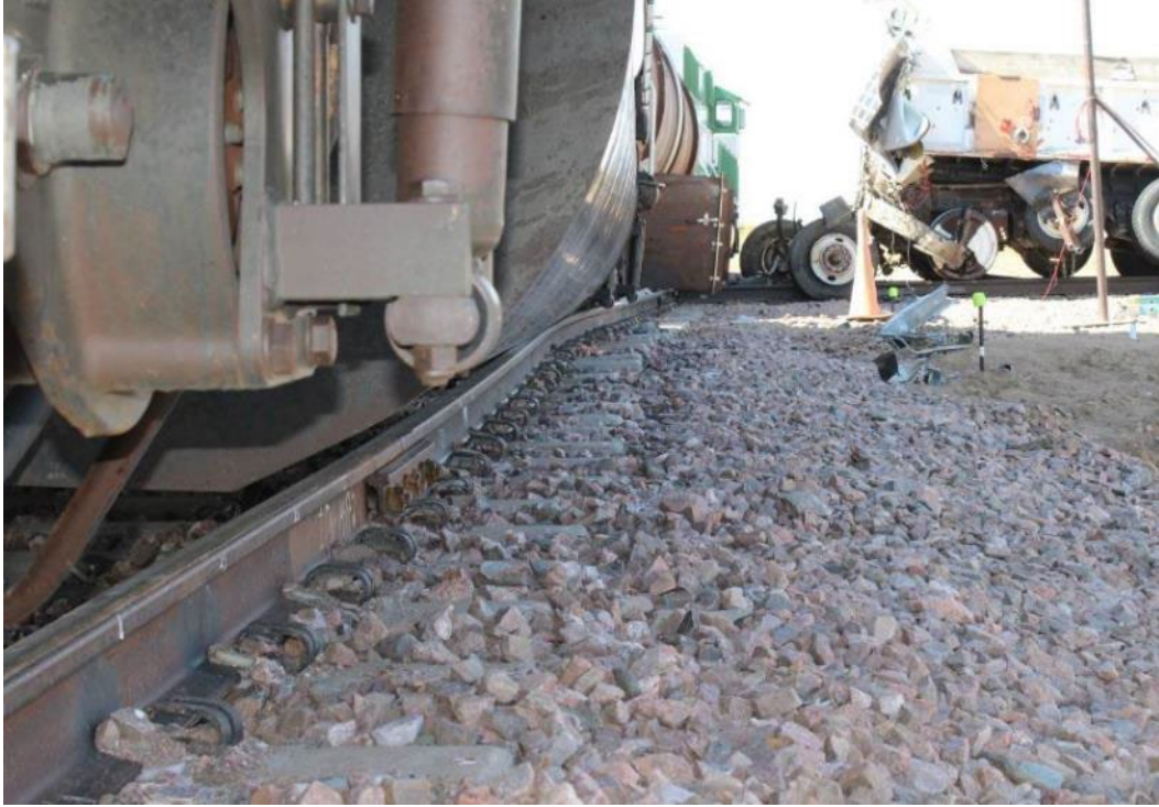
Figure 28. Track Shift on Ballast Bed
