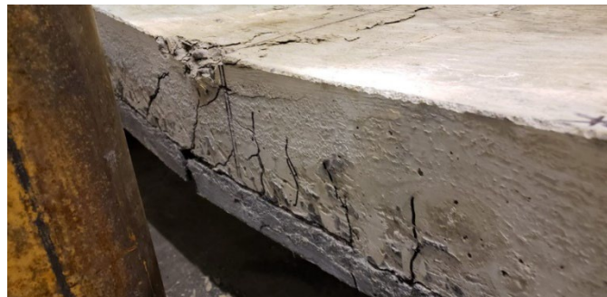
d) Midspan after failure, showing crushed concrete
