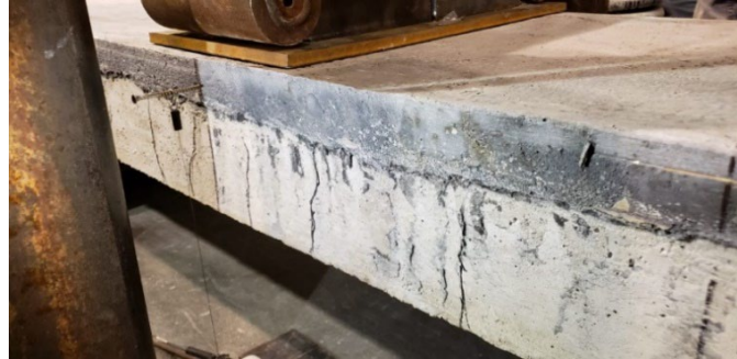
a) Flexural cracks initially forming
