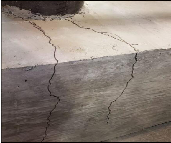
Figure 33: VT2/3-4 first cracks (69 k-ft)
