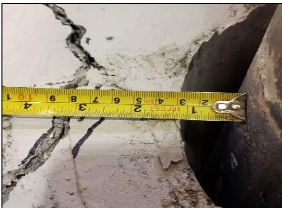
Figure 37: VT2/3-4 gap on back side of pile at failure from initial loading direction
