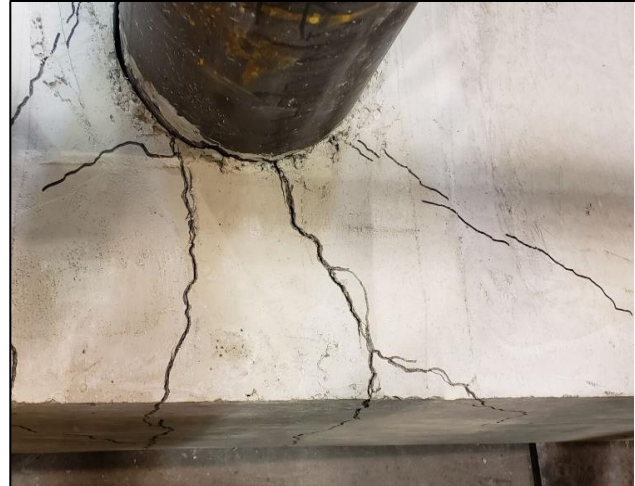
Figure 34: VT2/3-4 45-degree cracks (115 k-ft)
