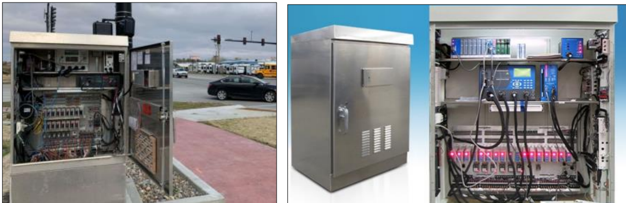
Figure 2.3: Typical TSC Cabinet (anon)
