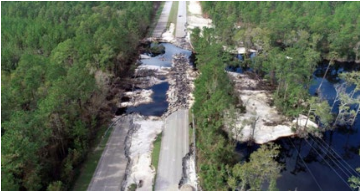
Figure 8. UAS Assessment of Flooding Across Road. (Image NCDOT)
