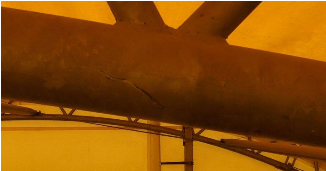
Figure 3. UAS Inspection of Damaged Beam within Wyoming Material Shed (Source: WYDOT)
