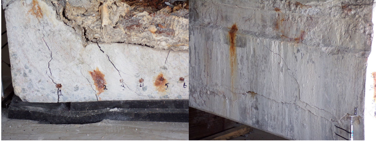
Figure 5.21: Cracking of Specimen E4 at south end triggering strand slip
