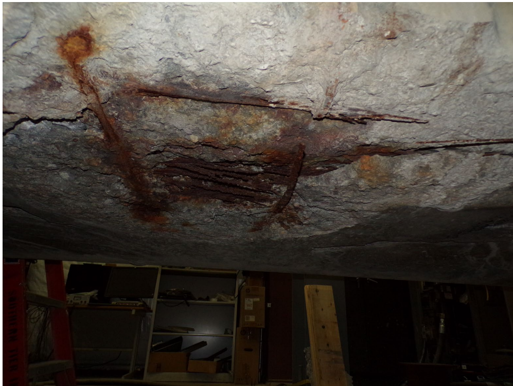
Figure 4.19: Exposed and corroded strand in the bottom of Specimen E3
