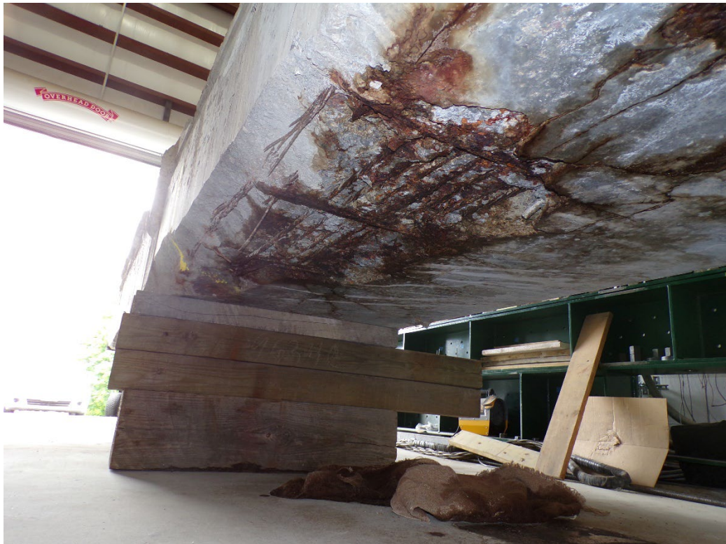
Figure 6.12: Specimen E3: visible deterioration of strands after spalling of concrete cover
