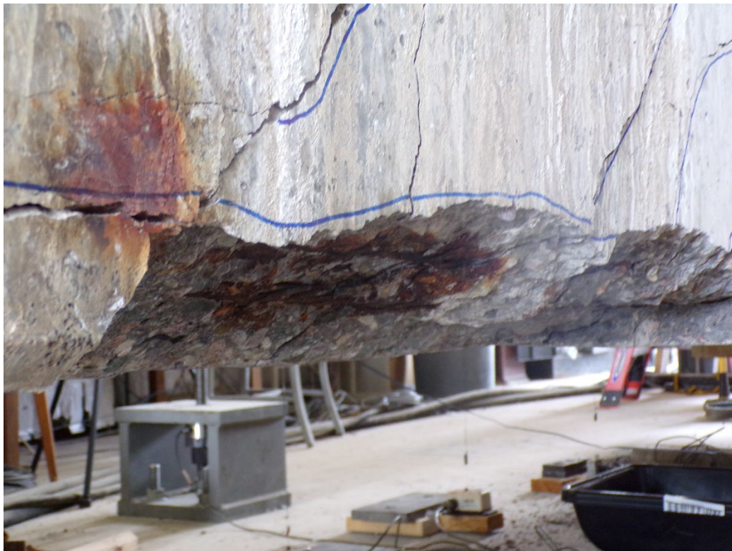
Figure 6.15: Visible strand corrosion and section loss in Specimen E9 after spalling
