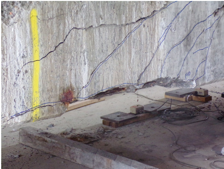
Figure 5.29: Flexure-shear cracking of Specimen E9 near peak load
