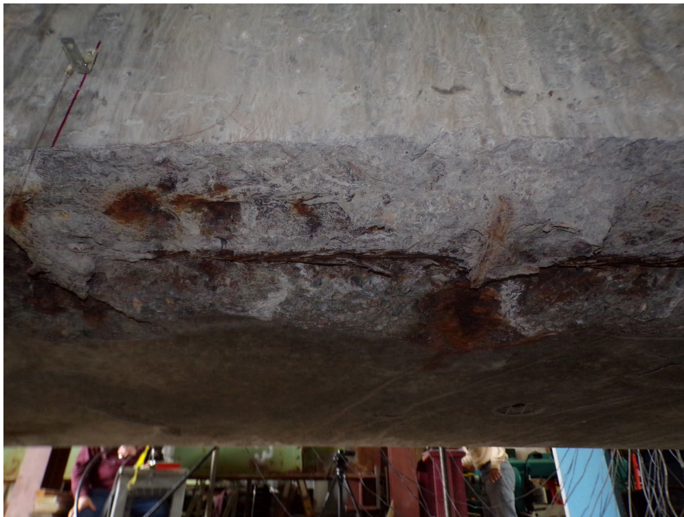
Figure 4.23: Spalled concrete corner in Specimen E9 exposing fractured strand
