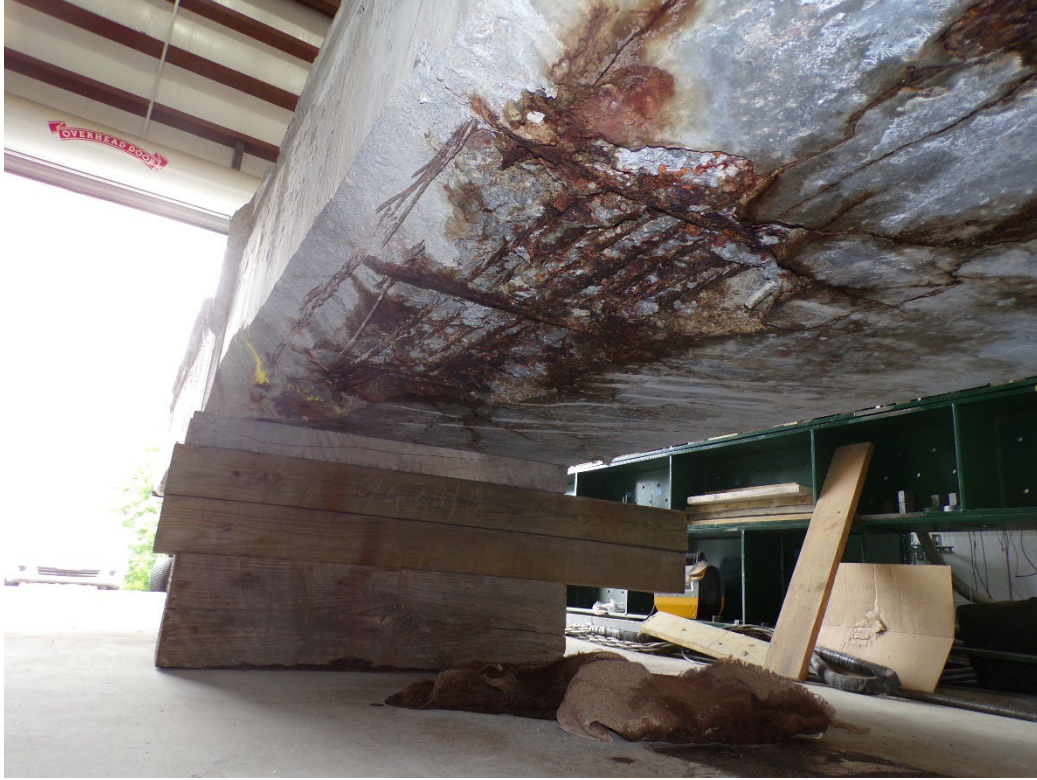
Figure 5.26: Severely corroded strand exposed in Specimen E3 after concrete spalling
