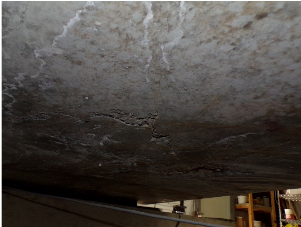
Figure 4.15: Bottom surface deterioration (Specimen E4)
