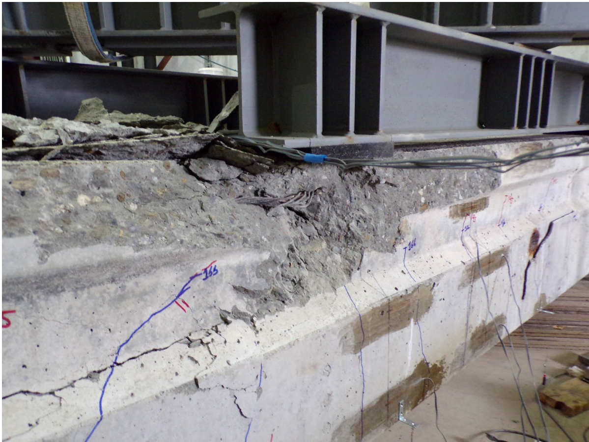
Figure 5.13: Concrete crushing at failure of Specimen R3
