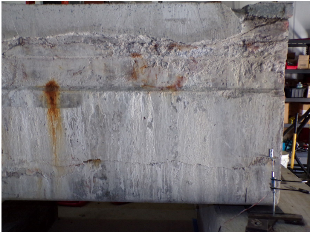
Figure 4.17: Longitudinal cracking at south end of Specimen E4
