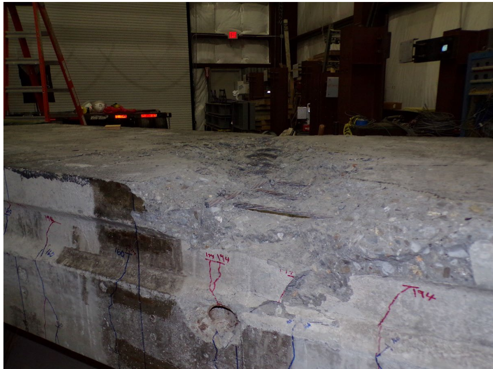
Figure 5.17: Concrete crushing after failure of Specimen R4
