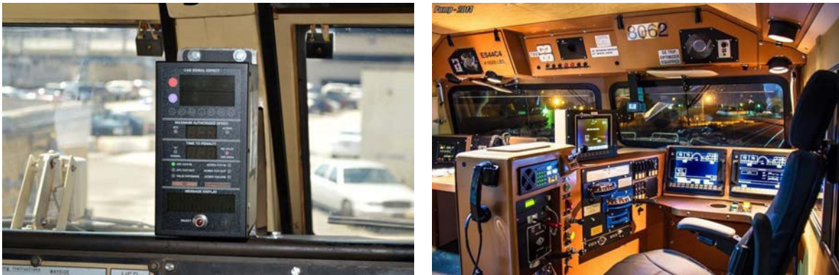
Figure 36. Left: A display for the ACSES positive train control system is mounted between the two windscreens; Right: Cab layout for a GE Evolution locomotive: Note the display atop the AAR control stand in the middle of the cabin
