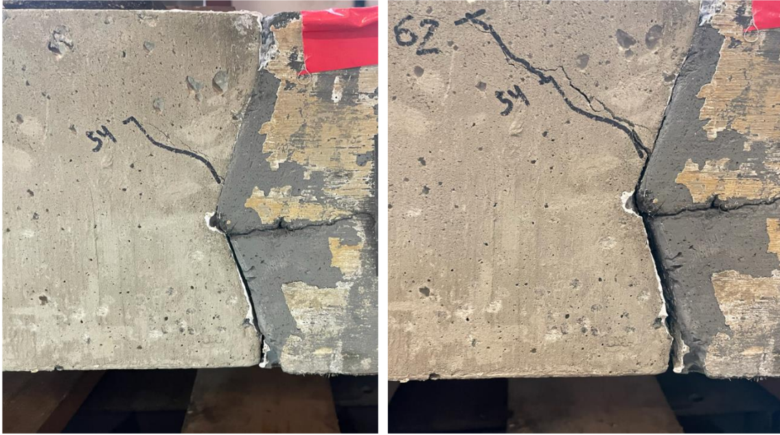
Left: 54 kips, Right: 62 kips Figure 7.12: Joint separation of specimen 2
