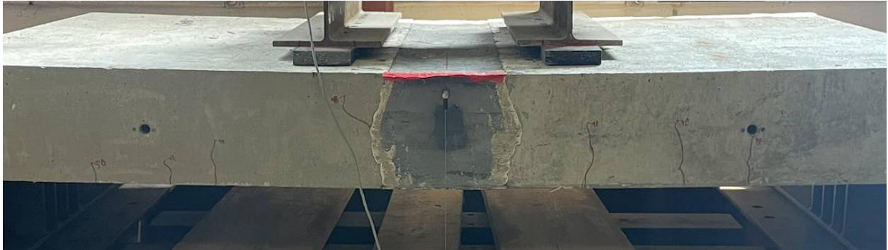
Figure 7.6: Initial cracking behavior of specimen 1
