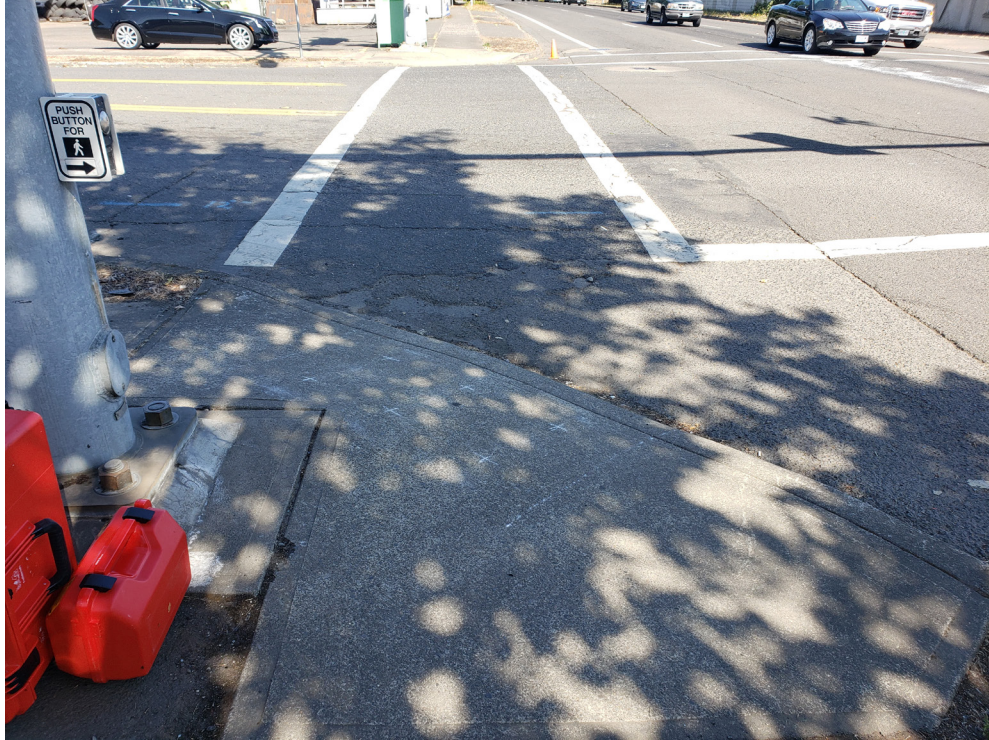
Figure 7.2: Example of a non-compliant curb ramp at the site of Salem, OR.
