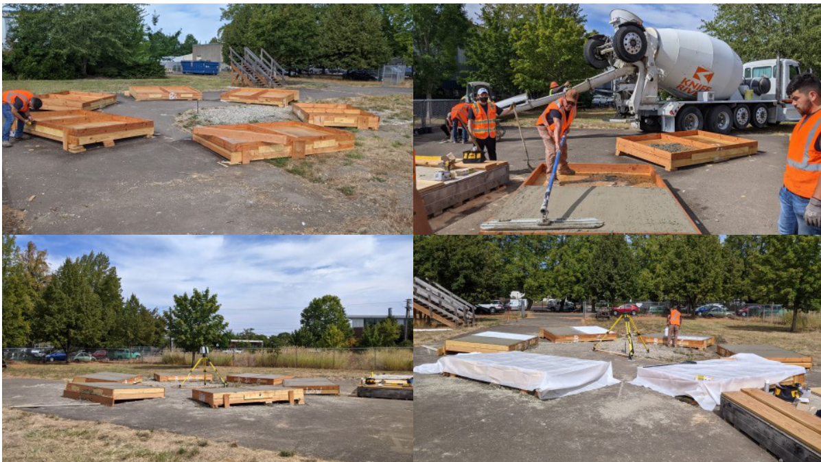
Figure 6.2: Ramp construction and survey configuration of the lab test for the concrete evaluation.
