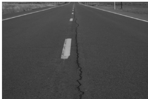
Figure 1. Photo. Example of longitudinal cracks (Ahmad & Khawaja, 2018).
