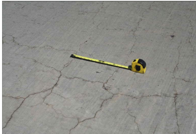
Figure 4. Photo. Example of map/pattern cracks in bridge decks (Wan et al., 2010).
