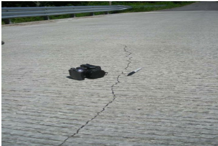
Figure 3. Photo. Example of diagonal cracks in bridge decks (Weiss et al., 2013).
