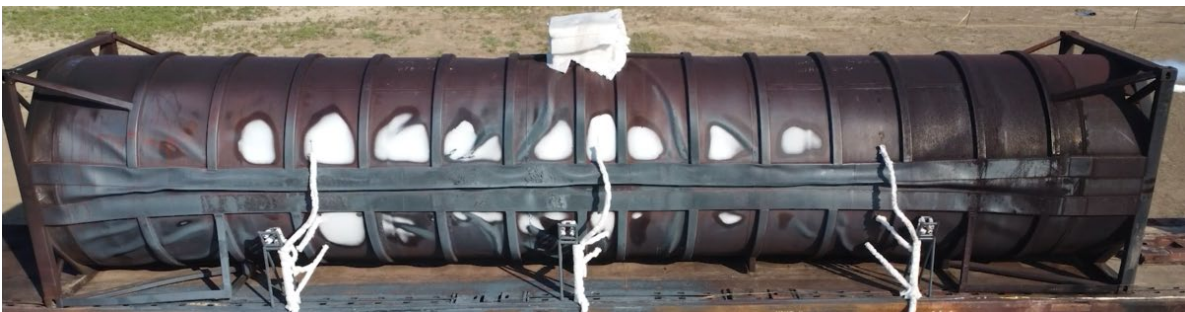
Figure 70. Frost on Deformed External Tank Jacket [1:07:24]
