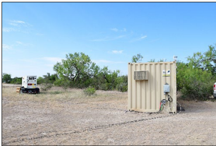
Container Control Room
