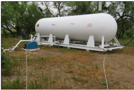
LPG Supply Tank, Pump and Bypass
