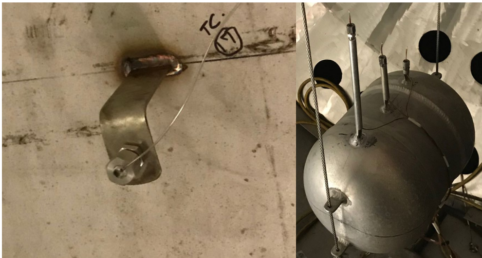
Figure 38. Vapor-space TCs; Tank-mounted (left), Float-mounted (right)
