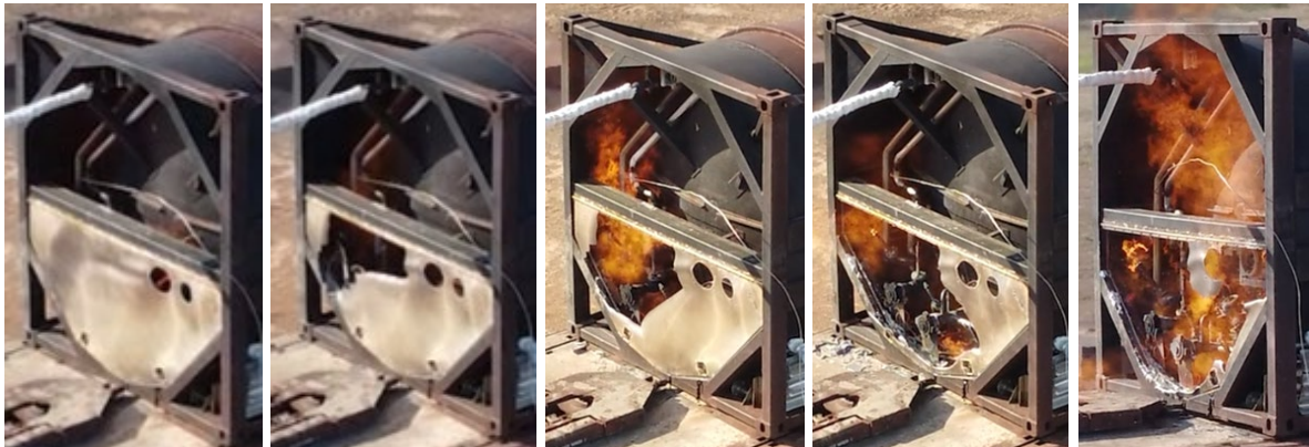
Figure 52. Progression of Piping Cabinet Door Failure over ~3 Min 50 s; Note the Increase in Fire Size as More of the Door is Melted [1:21:47 – 1:25:37]
