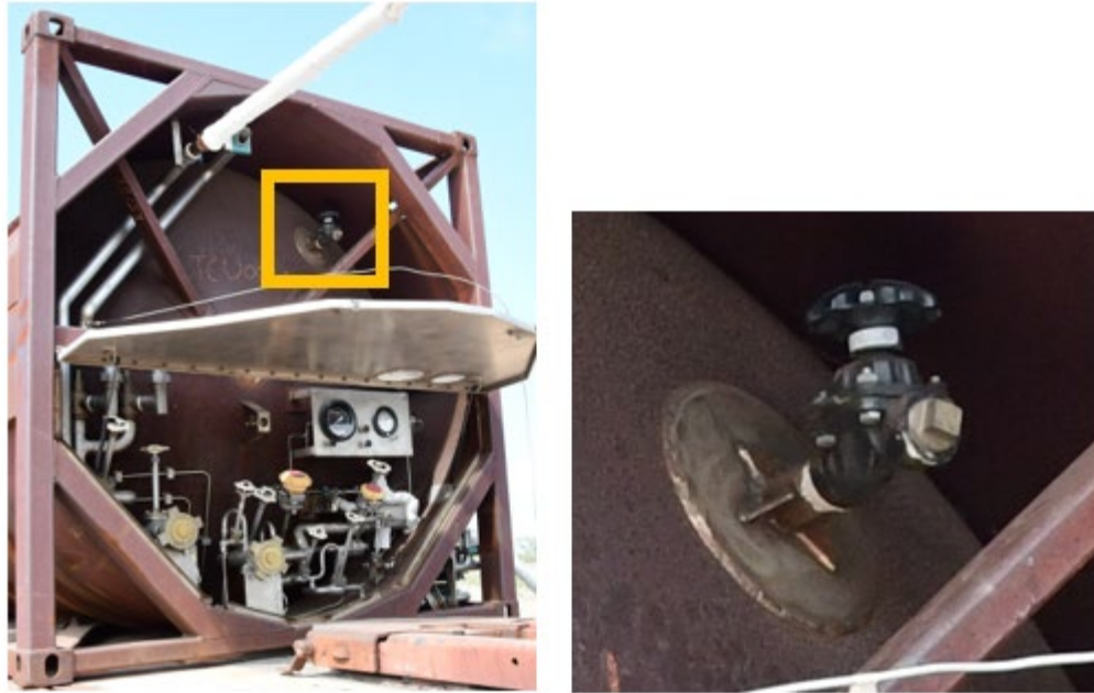
Figure 71. Trycock Valve Prior to Test
