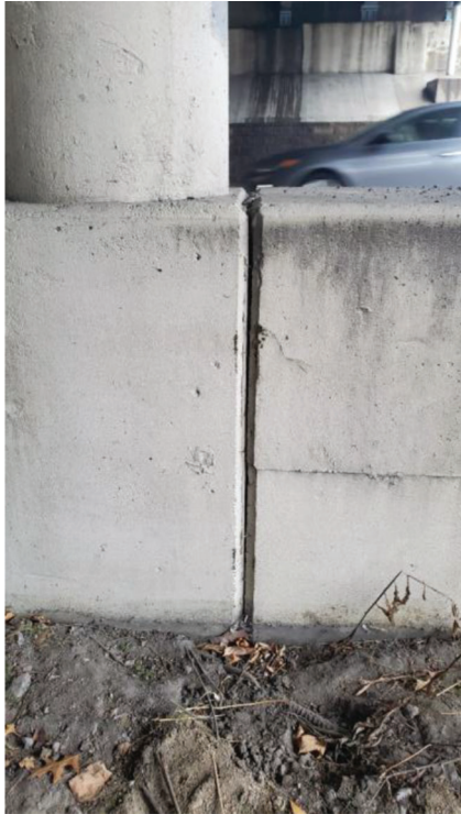
Figure 7.5 Photo of the crack in the joint connecting the original and widened portions of the interior pier (photo from United Consulting, personal communication, April 28, 2022).
