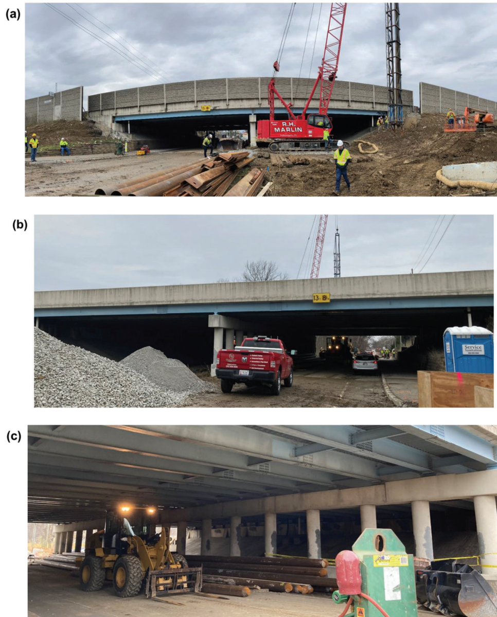
Figure 7.2 Bridge construction site: (a) I-465 Southbound side, (b) I-465 Northbound side, and (c) interior piers.
