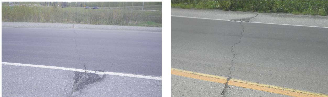
Photo 11 - Ramp 7 – General Transverse Cracking Conditions 2021 (left) and 2022 (right)
