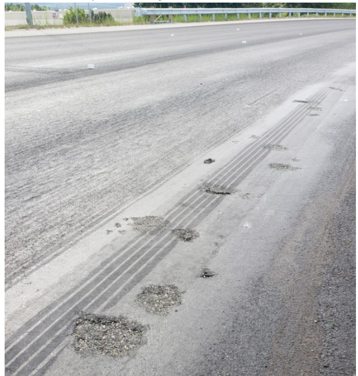
Photo 7 - Ramp 2 Flushing Distress
