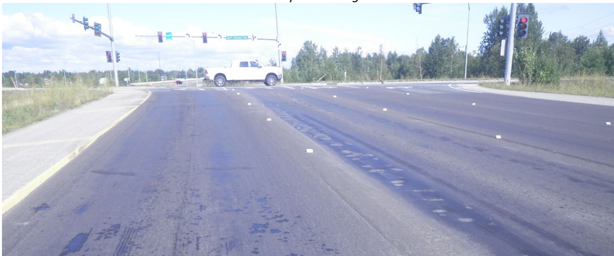
Photo 8 - Ramp 2 Flushing Distress
