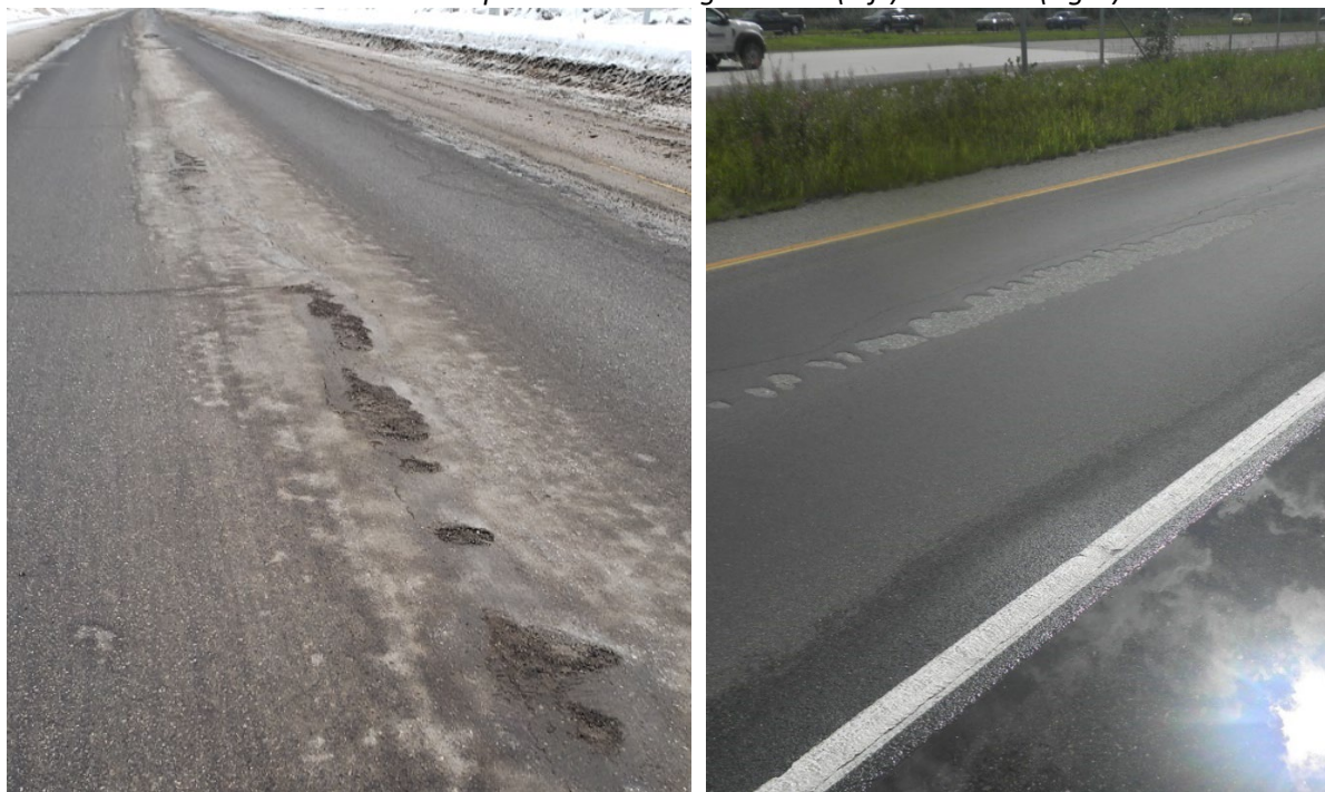
Photo 10 - Ramp 12 Plow Damage – 2021 (left) and 2022 (right)
