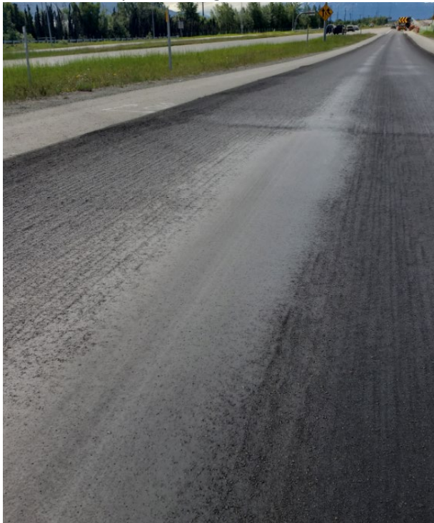
Photo 6 - Ramp 1 Flushing Distress
