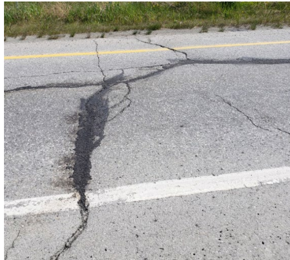
Photo 4 - Ramp 12 - Cracks after Surface Preparation
