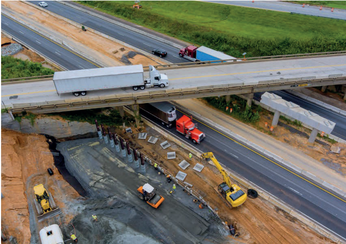
Highway construction projects, and others, benefit from AID Demonstration funding. © ungvart / AdobeStock.com.
