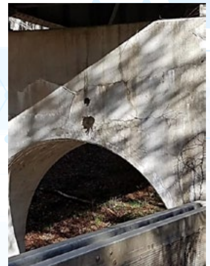
An example of concrete cracking caused by alkali-silica reaction gels.
