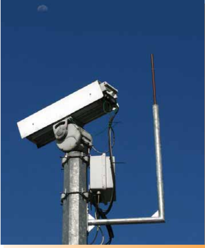
TYPICAL CCTV CAMERA ON POLE
