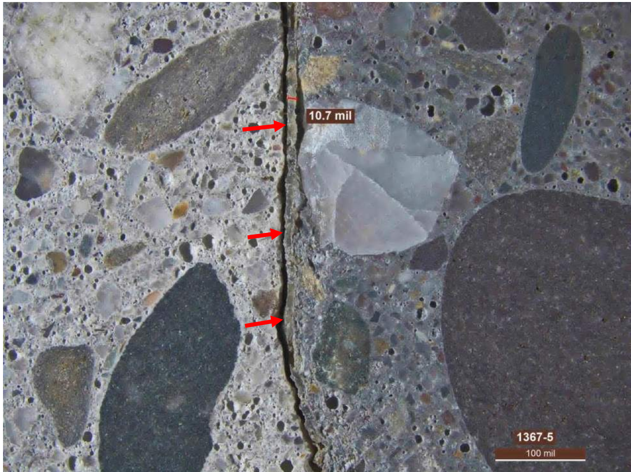
Figure C.6. Core 1367-5. Closeup view shows the crack sealer or PPC resin lining the crack.
