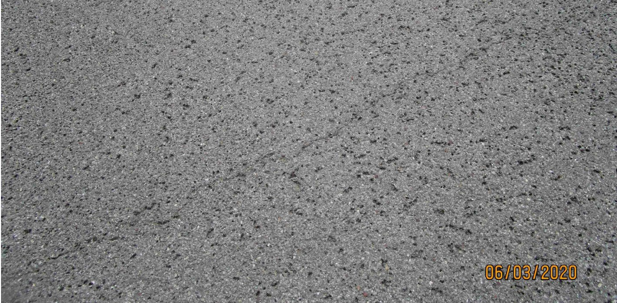
Figure 7. A transverse crack and aggregate pop-out in the HFST applied to MDT Bridge 1374, which is in the Missoula District. Image provided by MDT.
