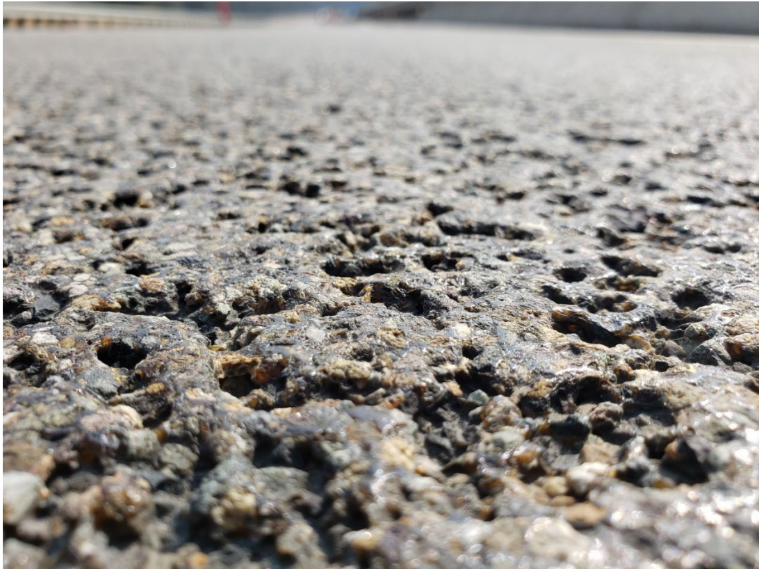
Figure 49. Close-up of HFST surface in right wheel path of driving lane on Bridge 1367 in 2022. Note polished surface and pockets of local loss of overlay.
