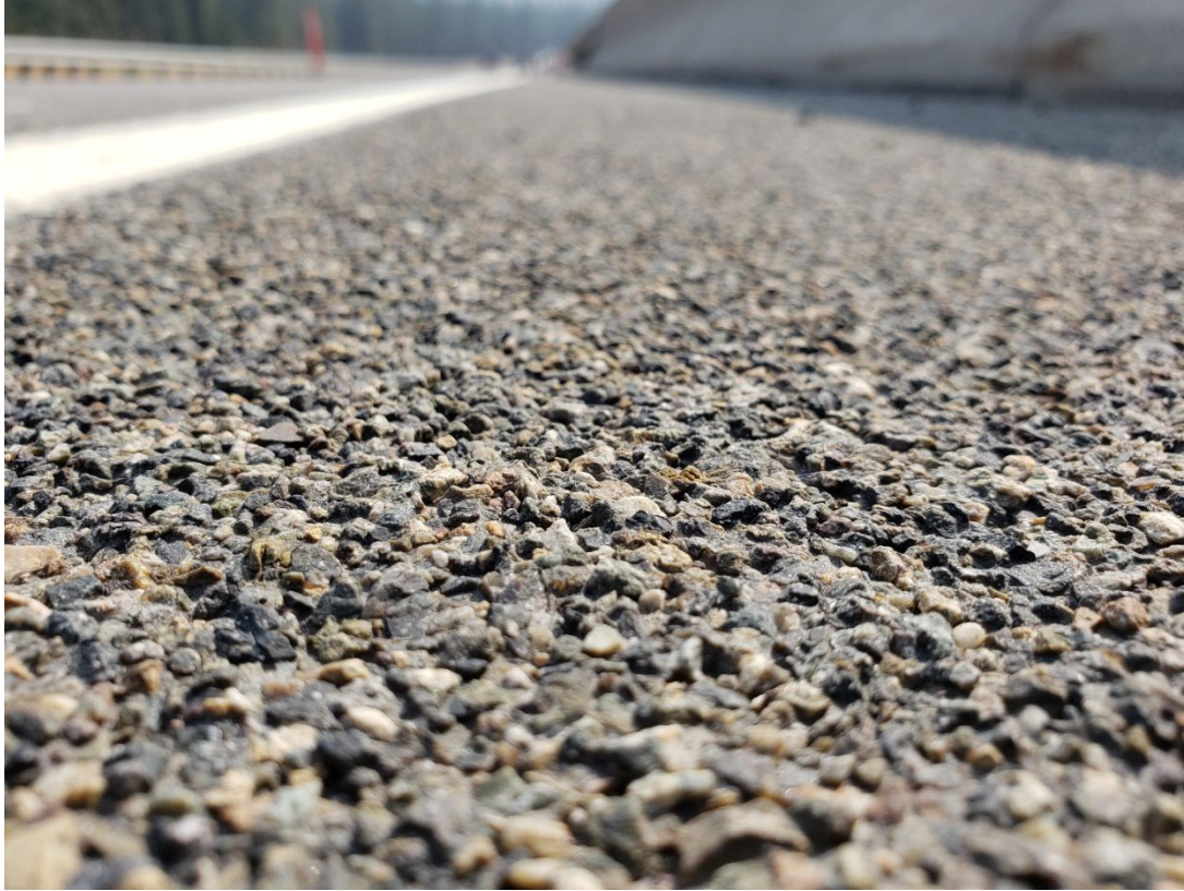
Figure 50. Close-up of HFST surface in shoulder on Bridge 1367 in 2022. Note aggregate remains proud and intact.
