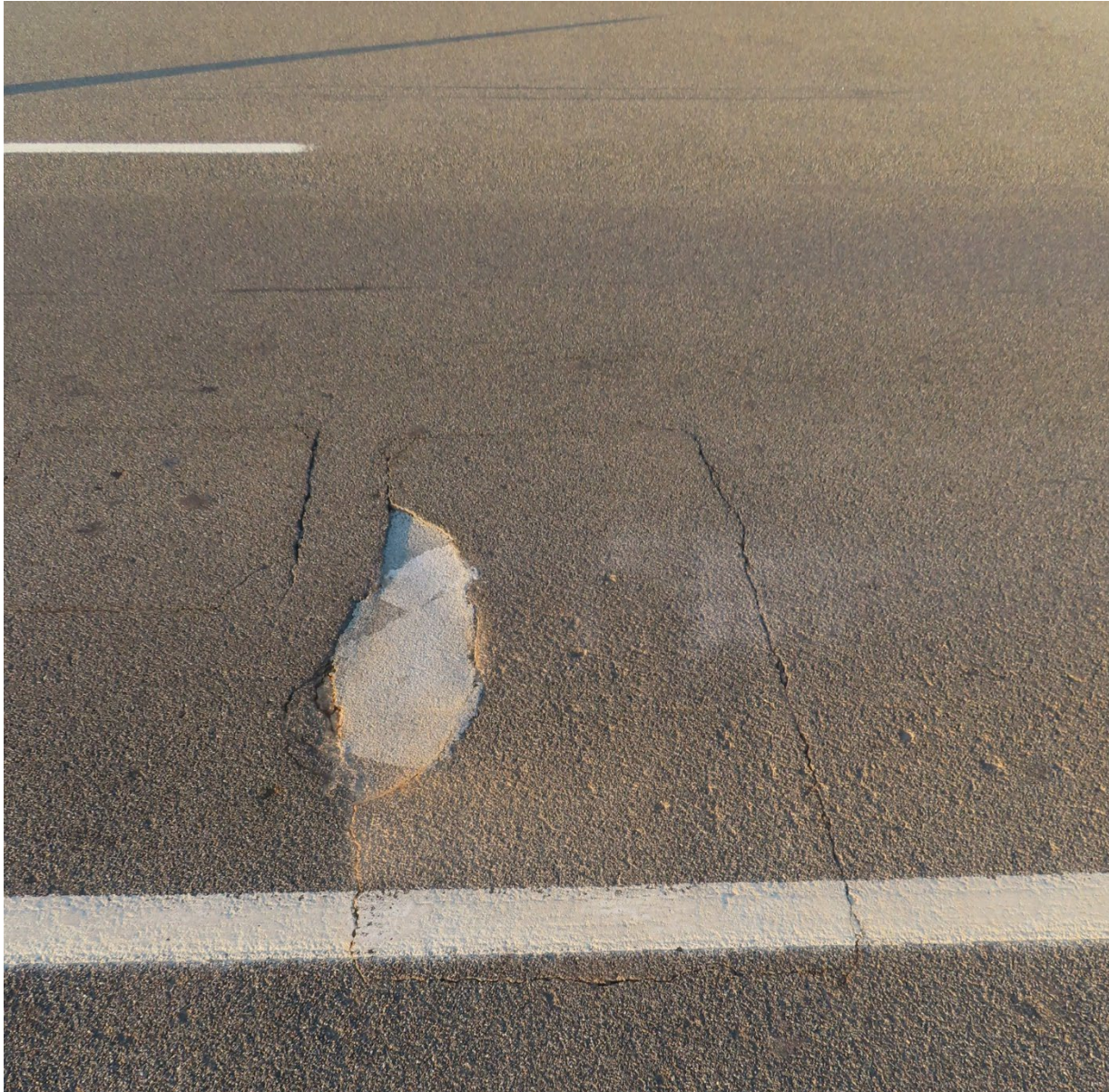
Figure 22. Photograph of reflective cracking and spalling of deck repairs and HFST on Bridge 1682 in 2020.
