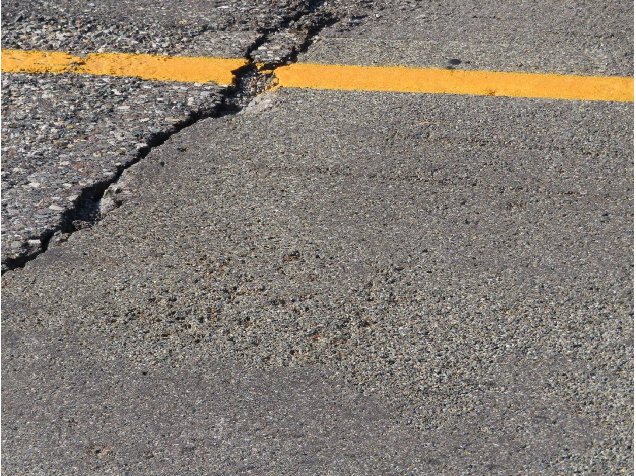
Figure 24. Area of overlay raveling and pockmarking in the HFST at Bridge 1682 in 2020.
