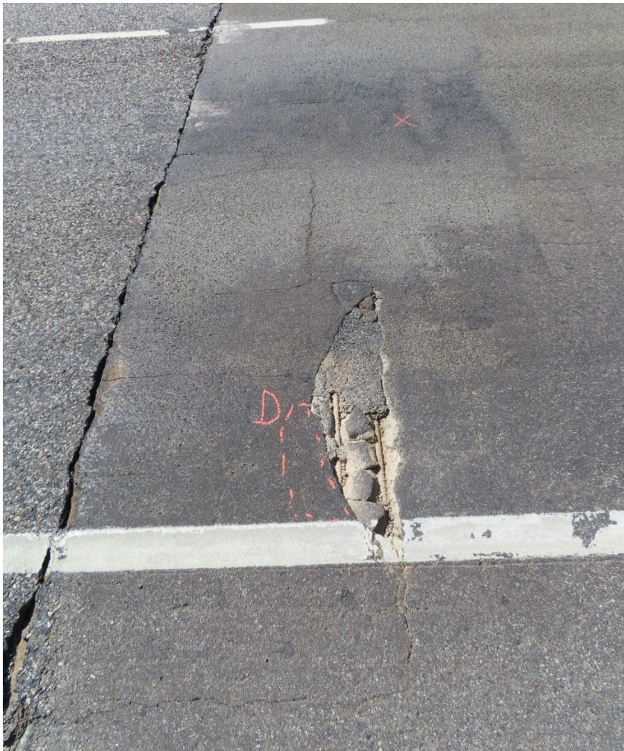
Figure 15. Spall exposing rebar and delamination on Bridge 1670, as seen in 2020 inspection. Loss of HFST at the bridge edge due to snow plow damage is visible in the upper left.
