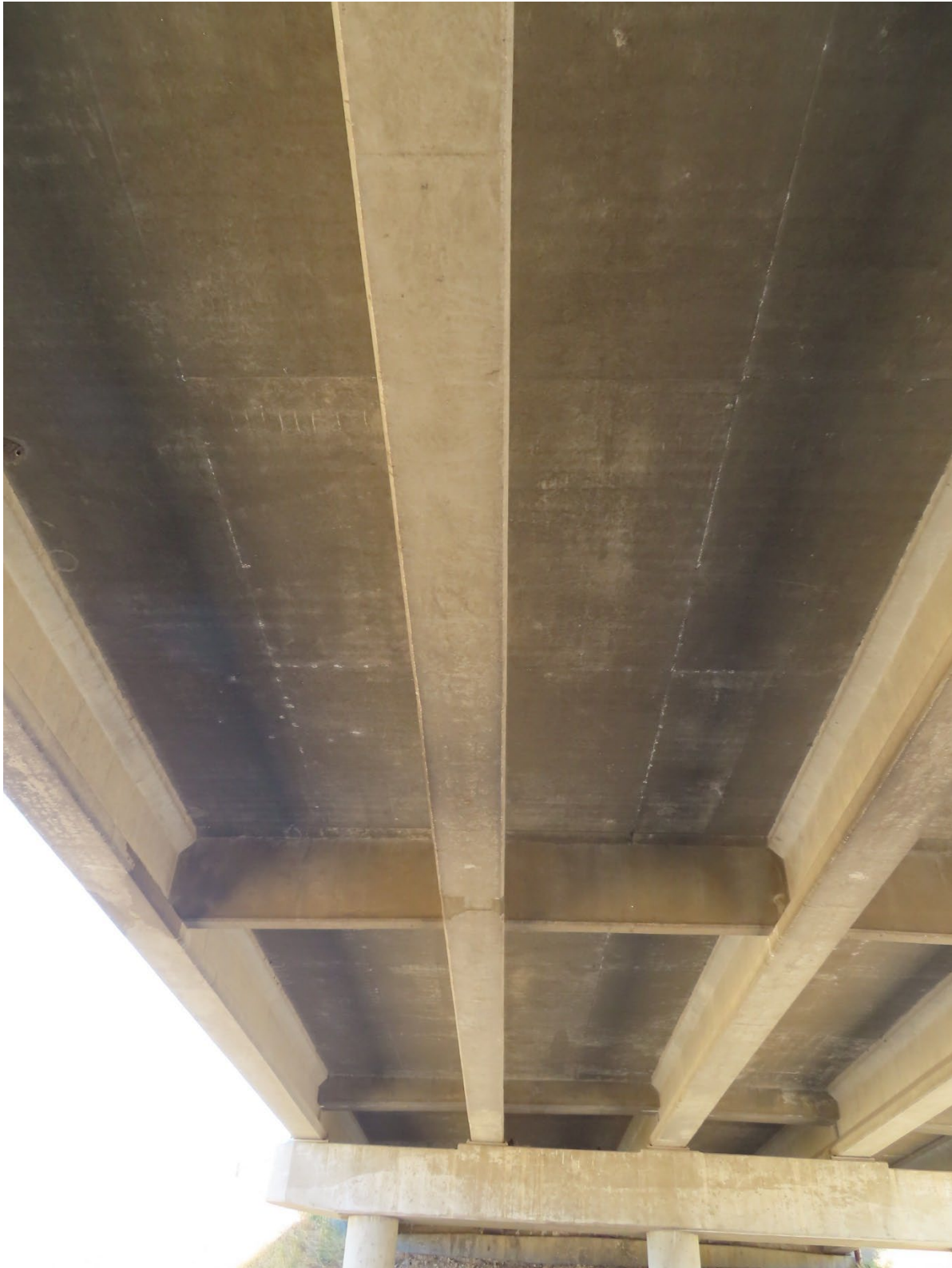
Figure 16. Image showing the typical conditions of the soffit of Bridge 1670 in 2020. Small amounts of efflorescence were present.
