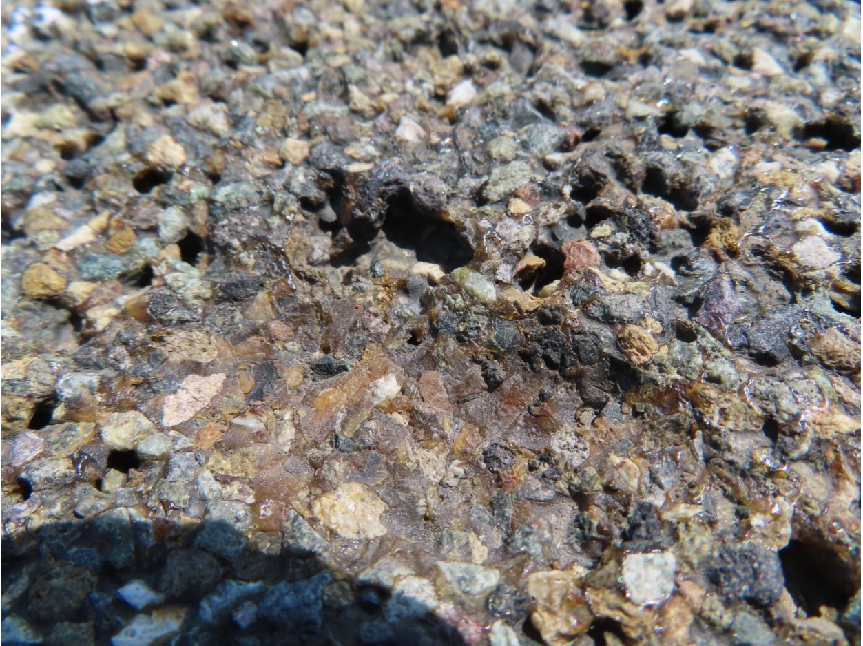
Figure 34. Close-up of the gouged area (likely plow damage) in the HFST of Bridge 1459 in 2020.
