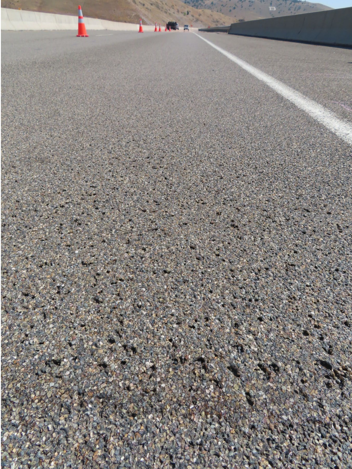
Figure 32. Photograph showing aggregate loss in the driving lane of Bridge 1459 in 2020.
