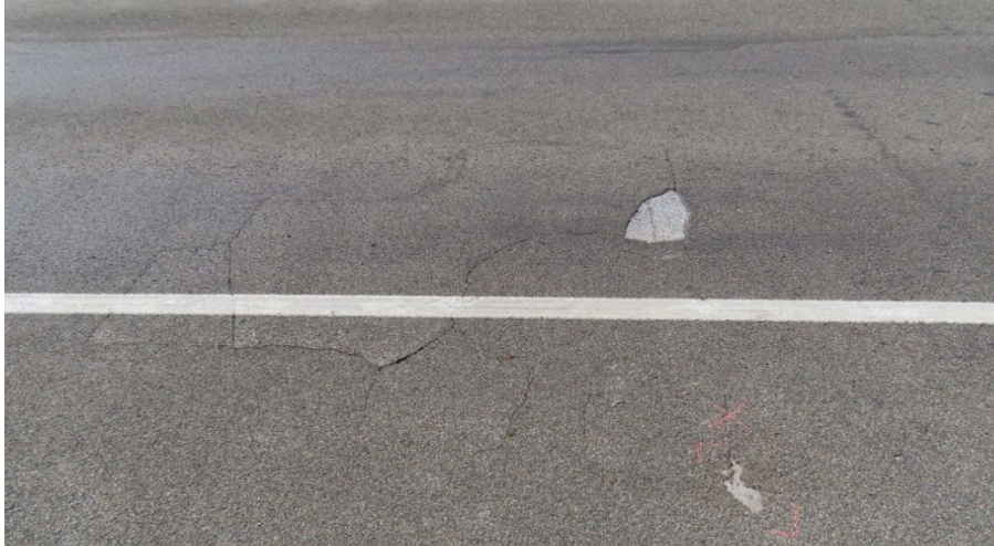
Figure 14. Reflective cracking in the driving lane of the HFST on Bridge 1670 and several spalls of the HFST, as of 2020.
