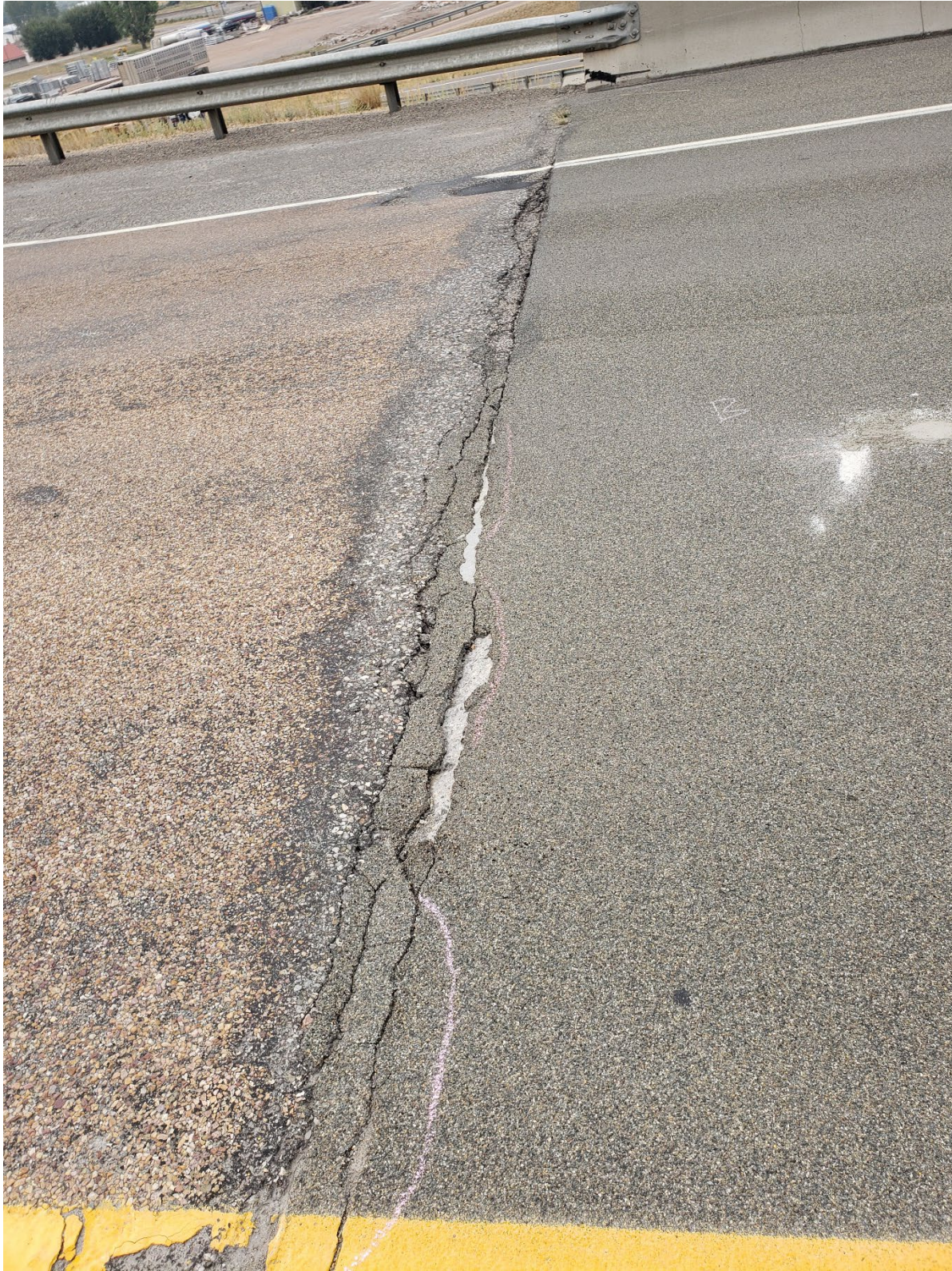
Figure 38. Cracking, spalling, and delamination of the HFST along the end of Bridge 1459 in 2022. Note this is the same joint as that shown in Figure 33 from 2020.
