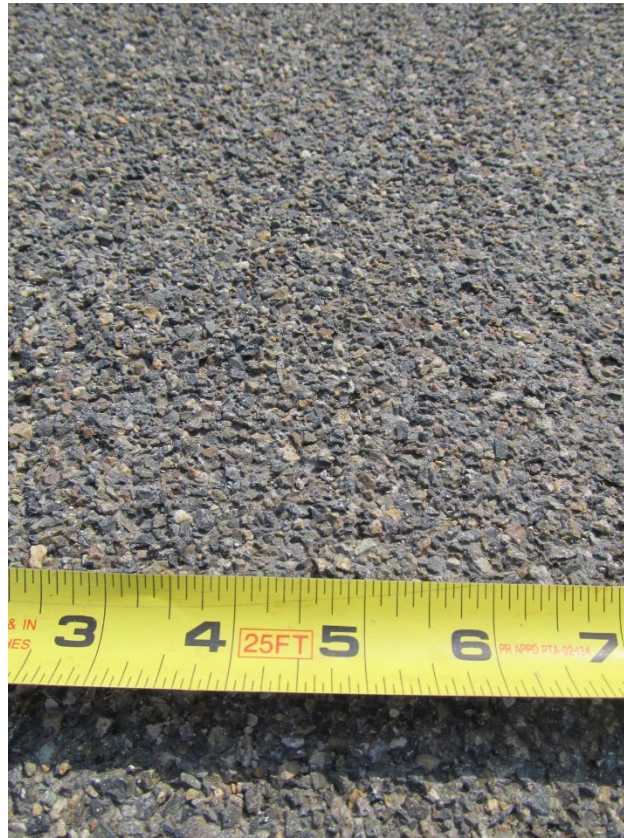
Figure 47. Close-up of shoulder surface on Bridge 1367 in 2022.
