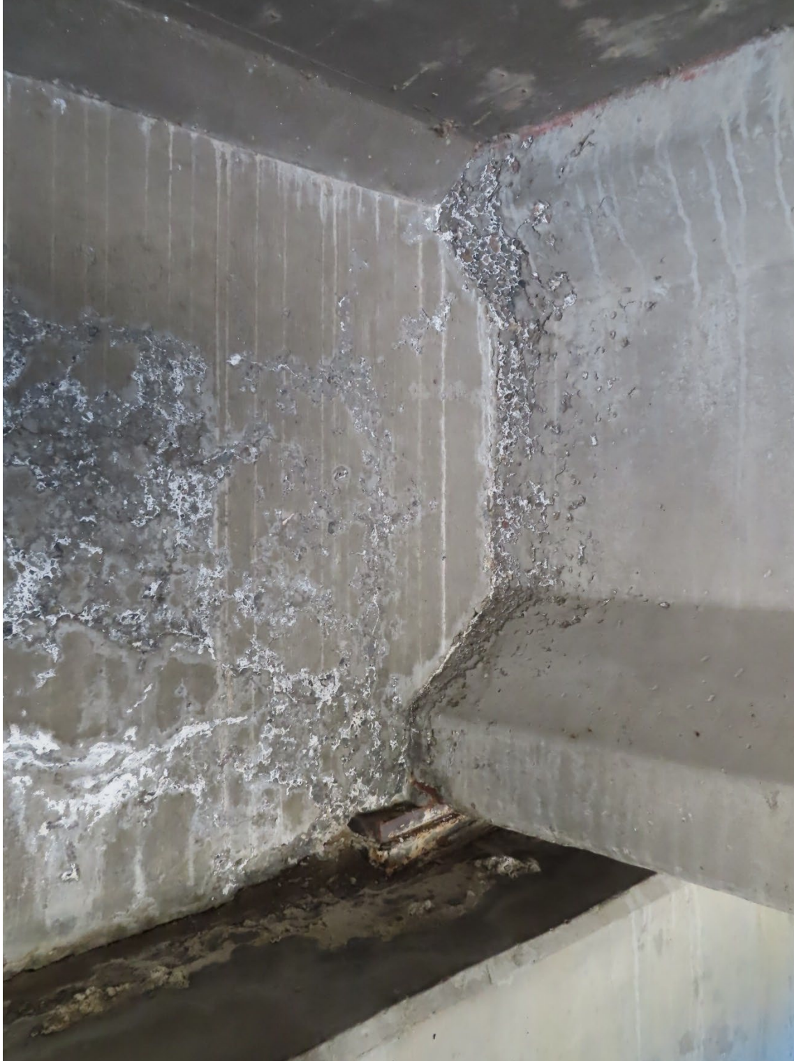
Figure 25. Close-up of distress on abutment and girder end at Bridge 1682 in 2020 suggesting significant moisture and deicer exposure.
