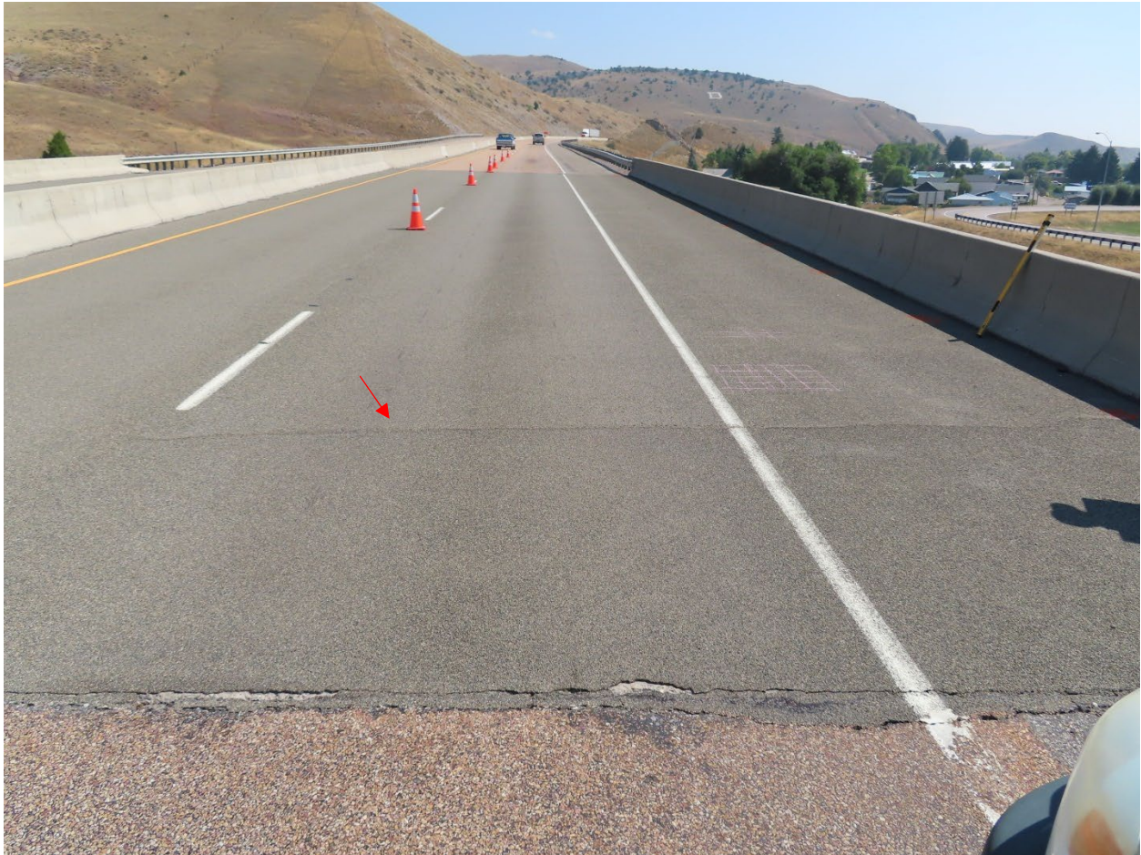
Figure 30. Overview of HFST on Bridge 1459 in 2020. The lap in the overlay is identified by the red arrow.
