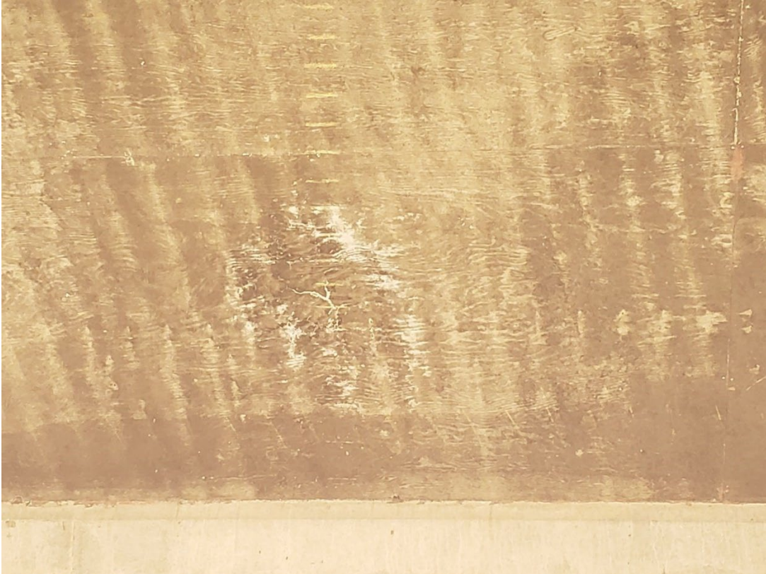
Figure 29. Area with a short, efflorescing crack on the soffit of Bridge 1682 in 2022.
