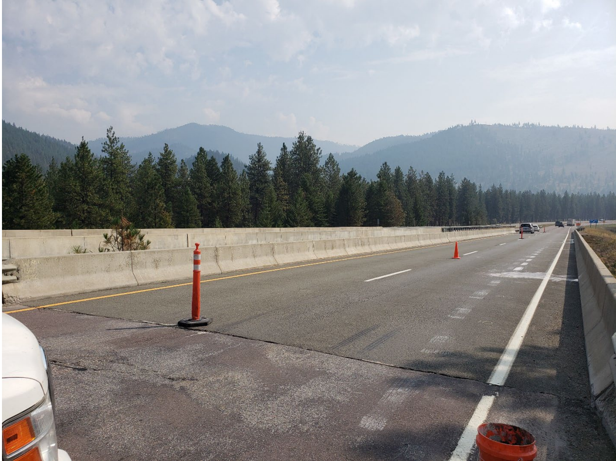
Figure 40. Overview of HFST approach on Bridge 1367 in 2022. Note photographer is facing in the direction of traffic.
