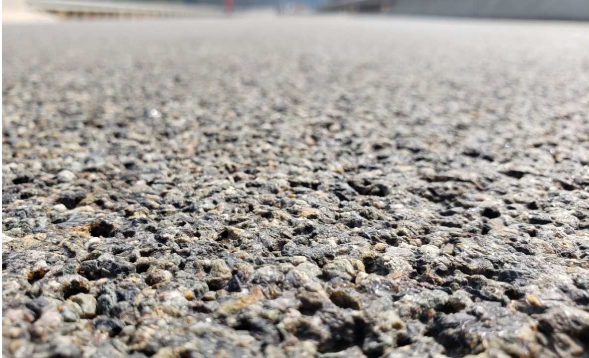
Figure 48. Close-up of HFST surface between wheel paths in driving lane on Bridge 1367 in 2022.
