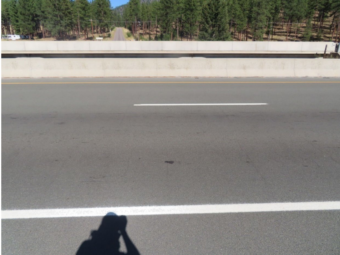
Figure 57. Photograph of a location on Bridge 1374 showing transverse cracking in 2020.
