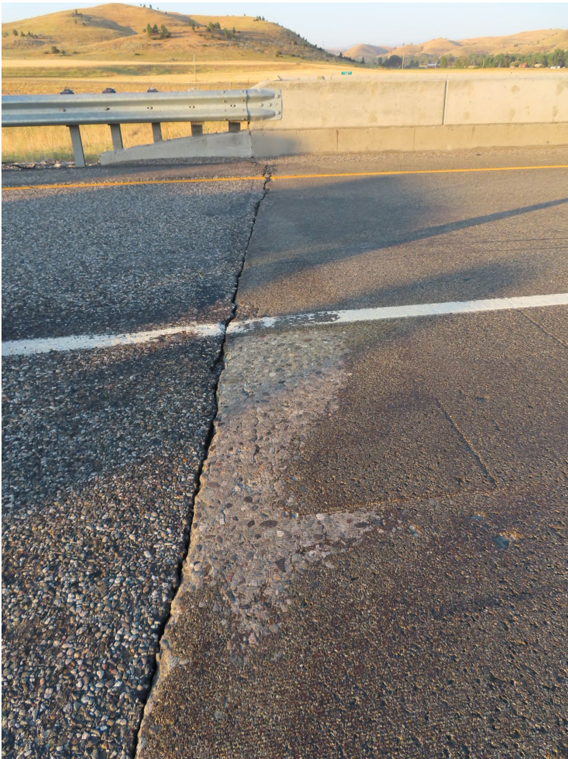
Figure 23. Abrasion/impact damage of the HFST at the leading approach edge of the HFST on Bridge 1682 in 2020.
