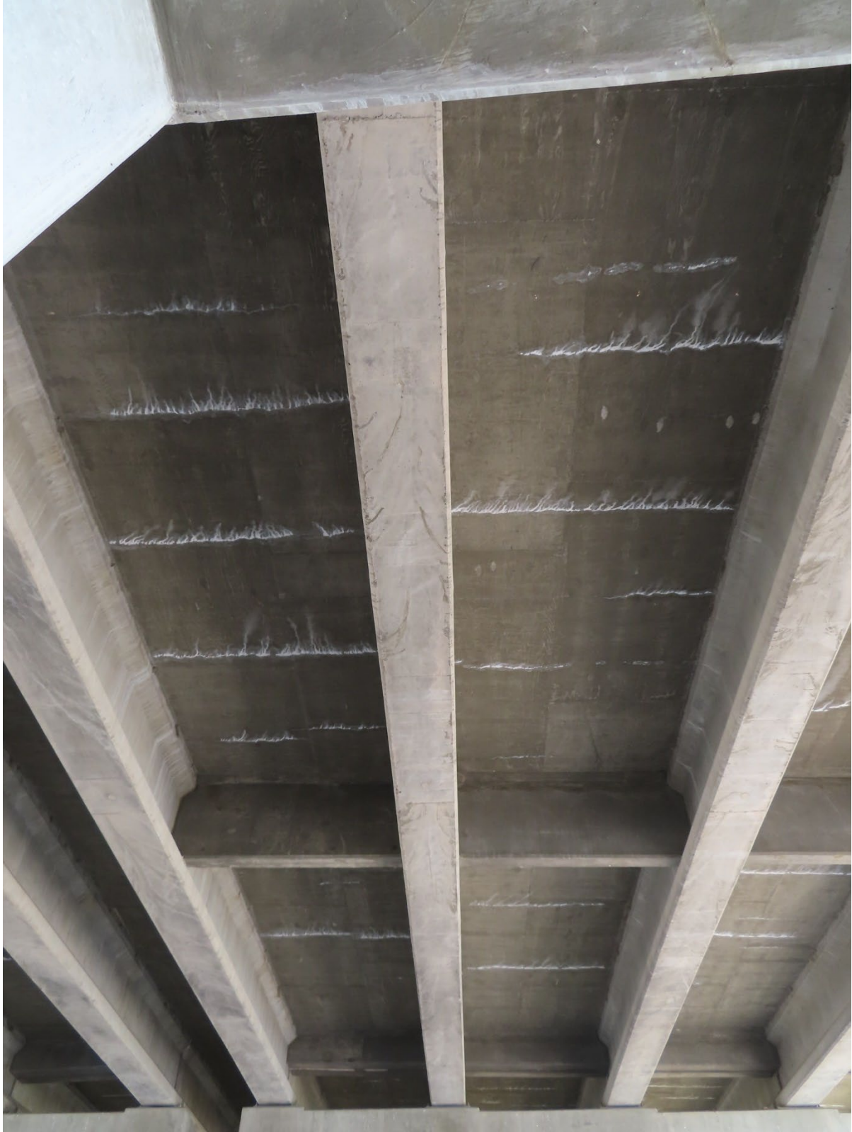
Figure 36. Photograph showing transverse cracking and efflorescence on the deck soffit of Bridge 1459 in 2020.
