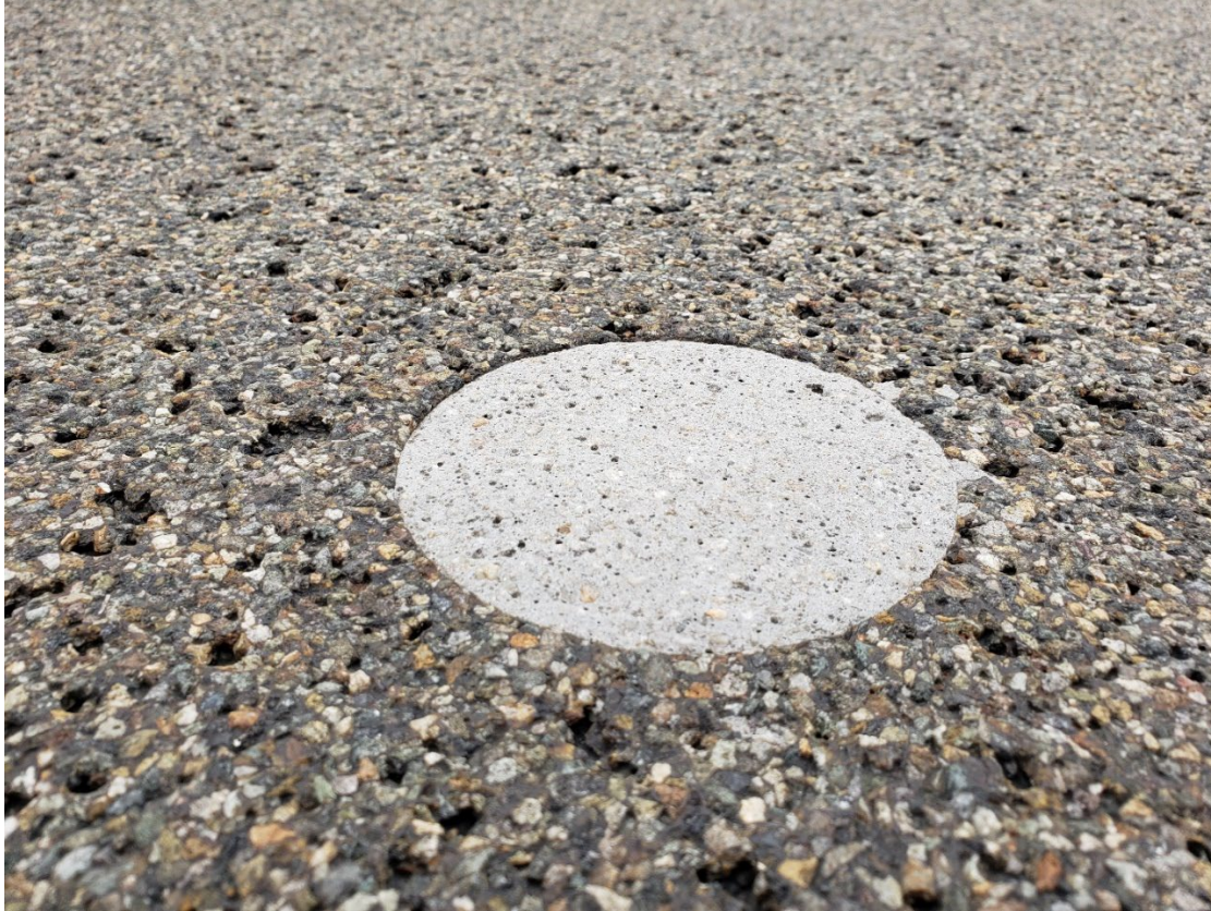
Figure 37. Close-up of the wearing surface in one of the wheel paths of the driving lane of Bridge 1459 in 2022 at prior core hole location. Polymer concrete is holding up well.
