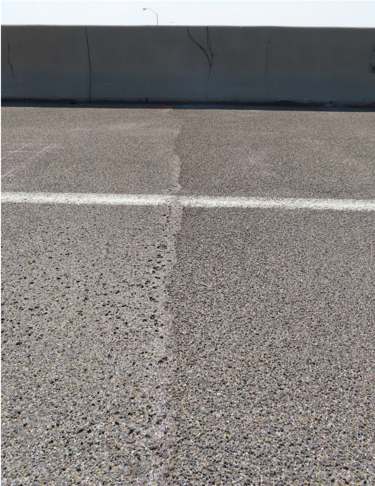
Figure 35. Close-up of the construction lap in the overlay of Bridge 1459 showing a clear difference in wear and texture in 2020.
