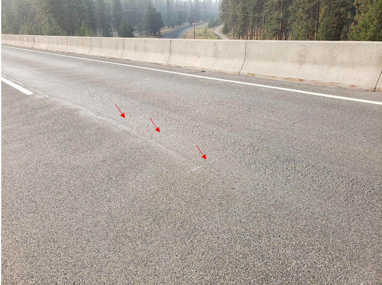
Figure 51. Photograph showing transverse cracking in the driving lane of Bridge 1367 in 2022. Some transverse cracks are identified with red arrows.
