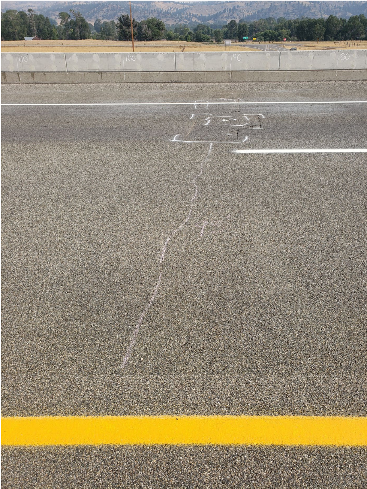
Figure 27. Transverse crack near bent in Bridge 1682 in 2022.
