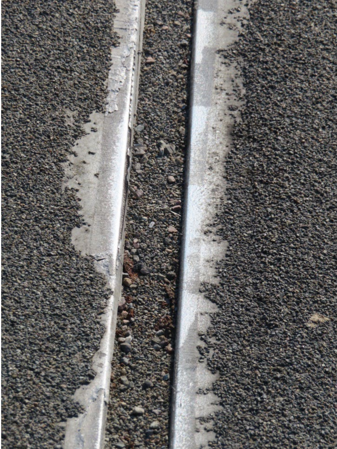
Figure 53. Photograph showing aggregate debris in an armored joint on Bridge 25 and encroachment of the polymer overlay onto the joint armor.
