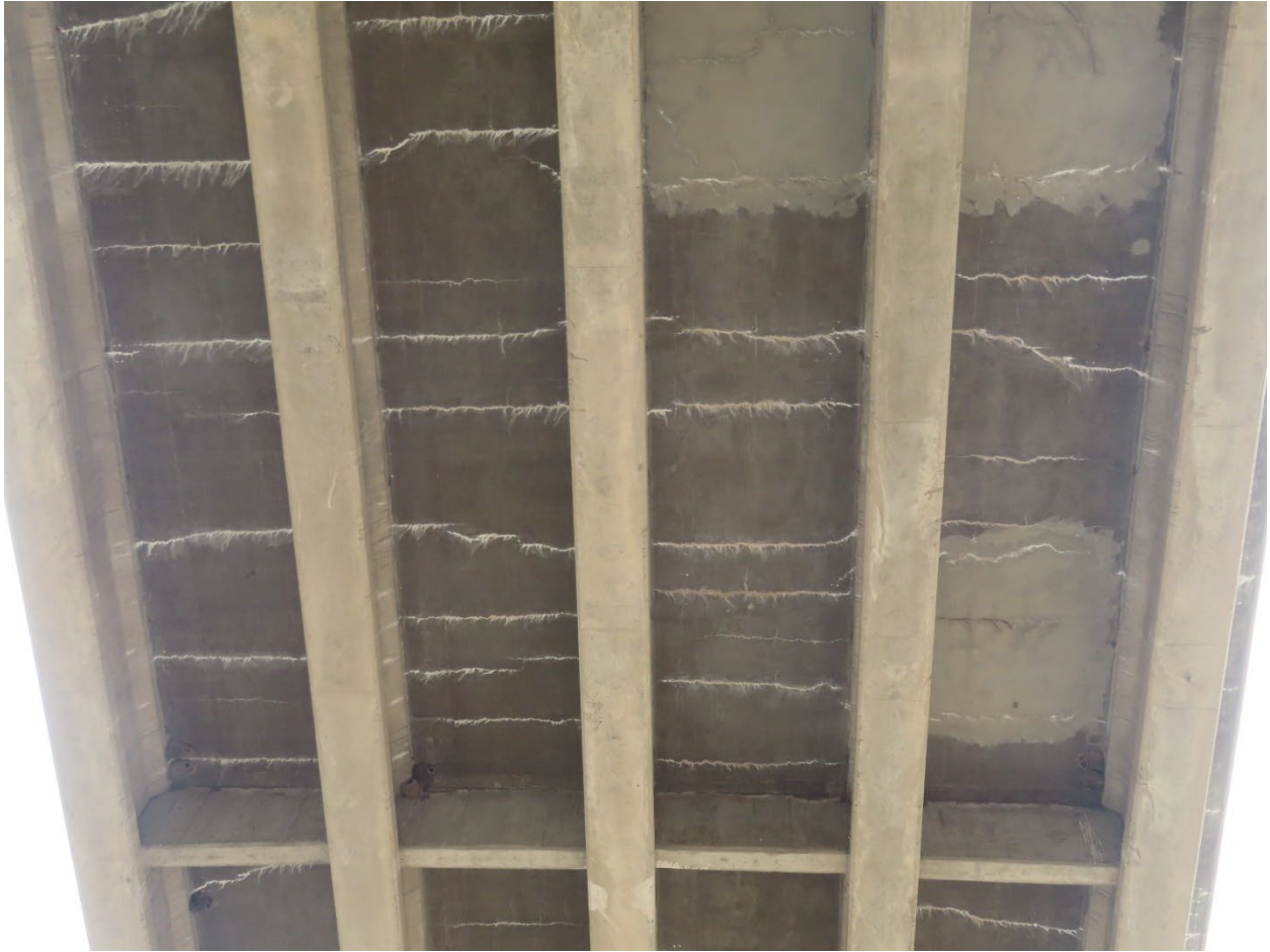
Figure 45. Photograph of soffit of Bridge 1367 in 2020 showing transverse cracks with efflorescence and full-depth repairs.
