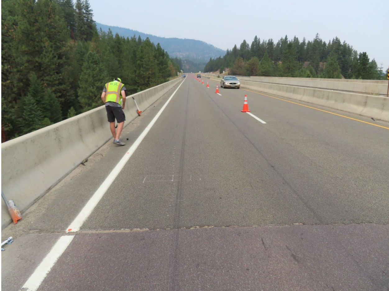
Figure 39. Overview of HFST on Bridge 1367 in 2020. Note photographer is facing into oncoming traffic.
