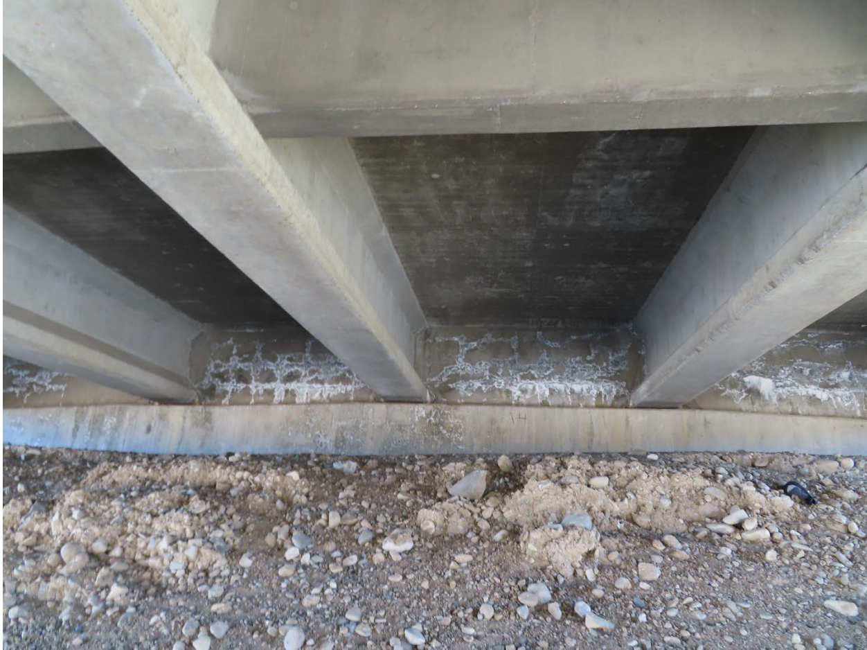
Figure 17. Photograph showing moisture efflorescence, cracking, and distress on the abutments of Bridge 1670 as of 2020.
