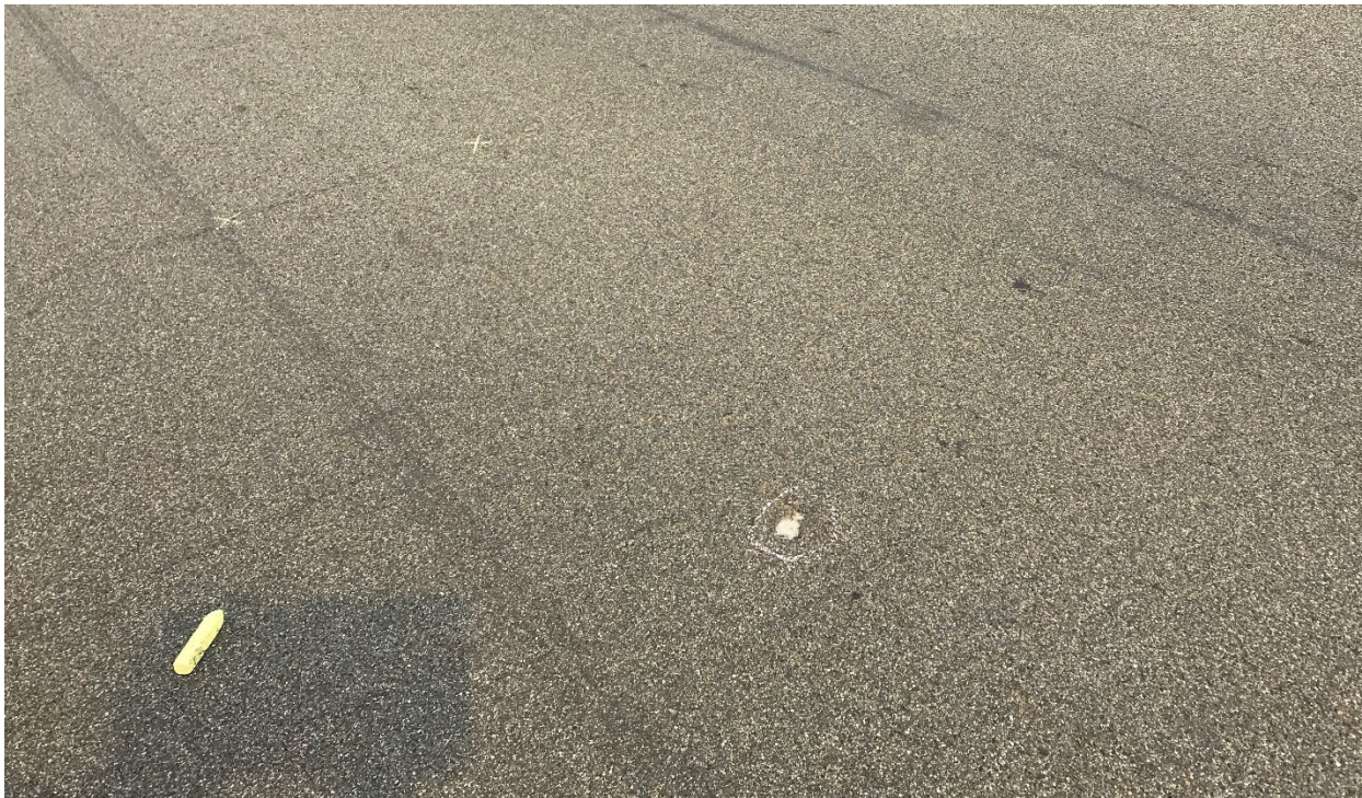
Figure 44. Small spall and transverse cracks in HFST on Bridge 1367 in 2020.
