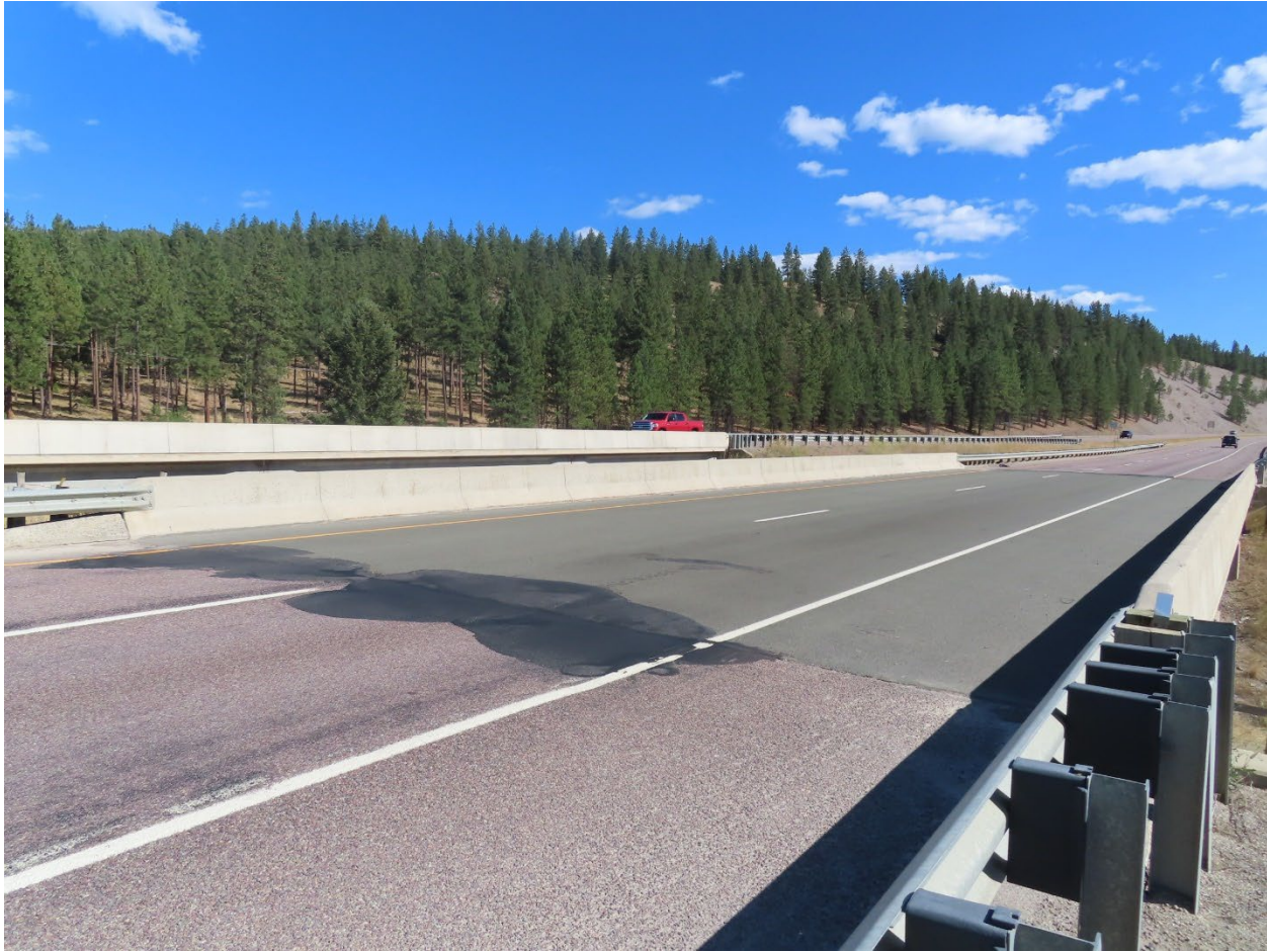
Figure 54. Large bituminous patch present at the entrance onto Bridge 1374.
