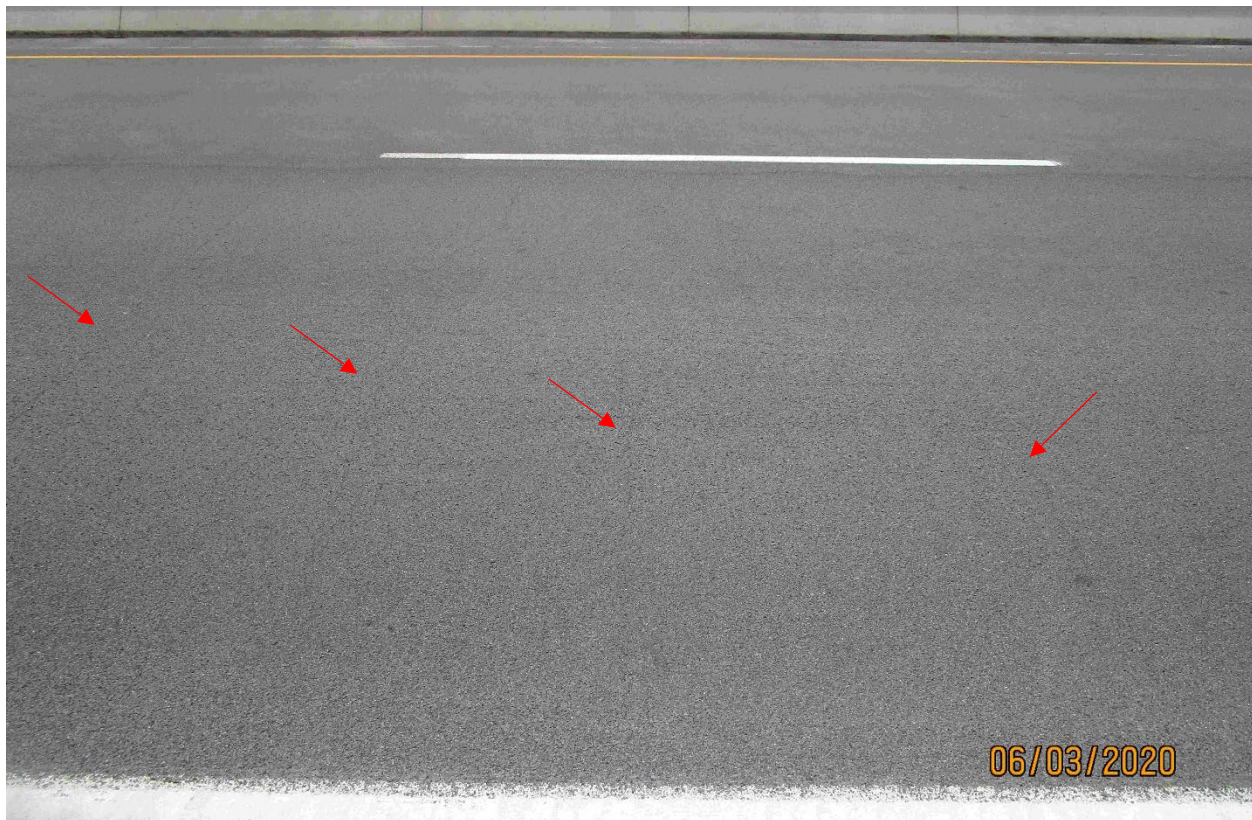
Figure 6. Transverse cracks in a HFST applied to MDT Bridge 1374, which is in the Missoula District. Image provided by MDT. Red arrows added by WJE to point out the transverse cracks.
