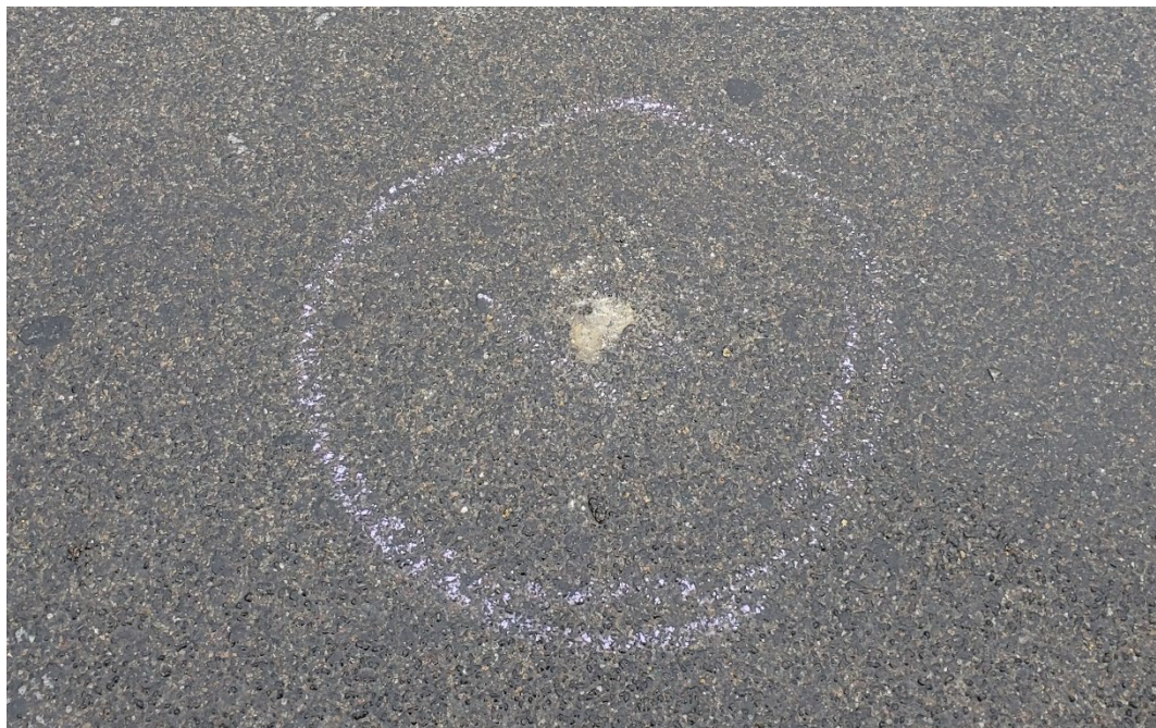
Figure 55. Area identified as delaminated on Bridge 3734 in 2022. The “spall” at the center is due to chipping the HFST away to determine if the delamination was at the HFST-deck interface or due to reinforcement corrosion.
