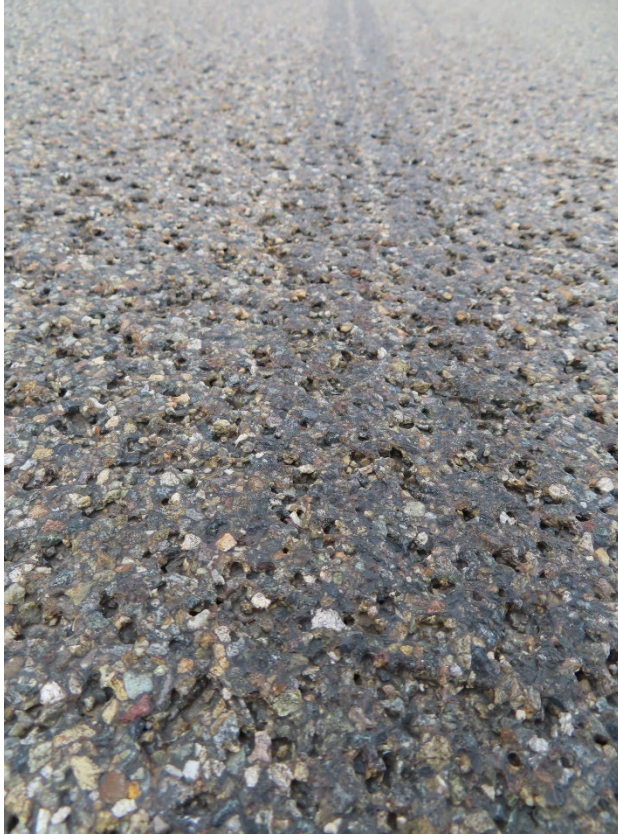
Figure 42. Close-up of overlay pop-out and wear in the driving lane of Bridge 1367 in 2020.
