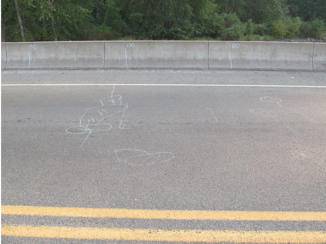
Figure 59. Photograph of largest delaminated area identified on Bridge 1333 in 2022.
