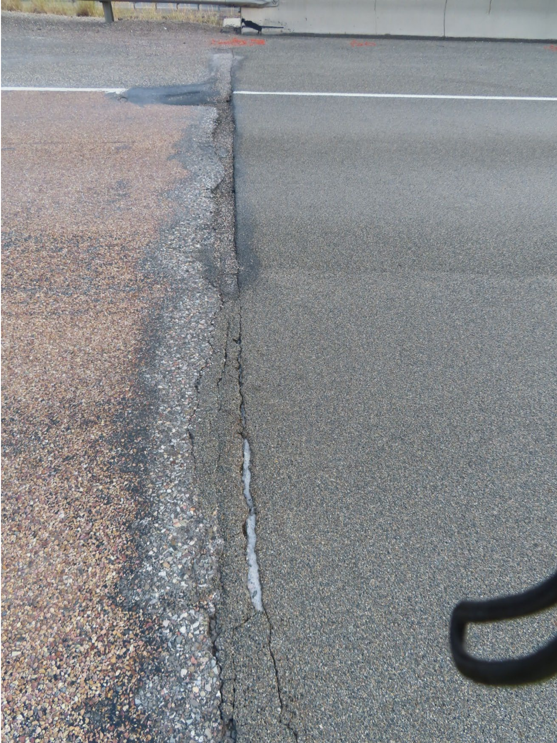
Figure 33. Cracking and spalling of the HFST at the end of Bridge 1459 in 2020.
