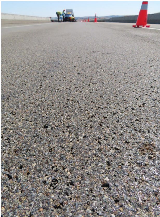
Figure 12. Photograph of wear and aggregate pop-out in driving lane of Bridge 1670 in 2020.
