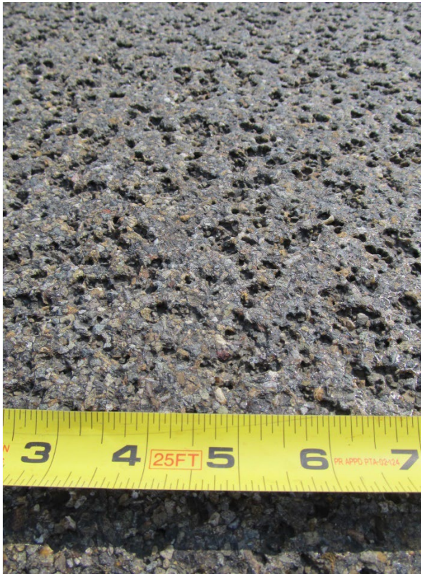
Figure 46. Close-up of wheel path surface on Bridge 1367 in 2022.
