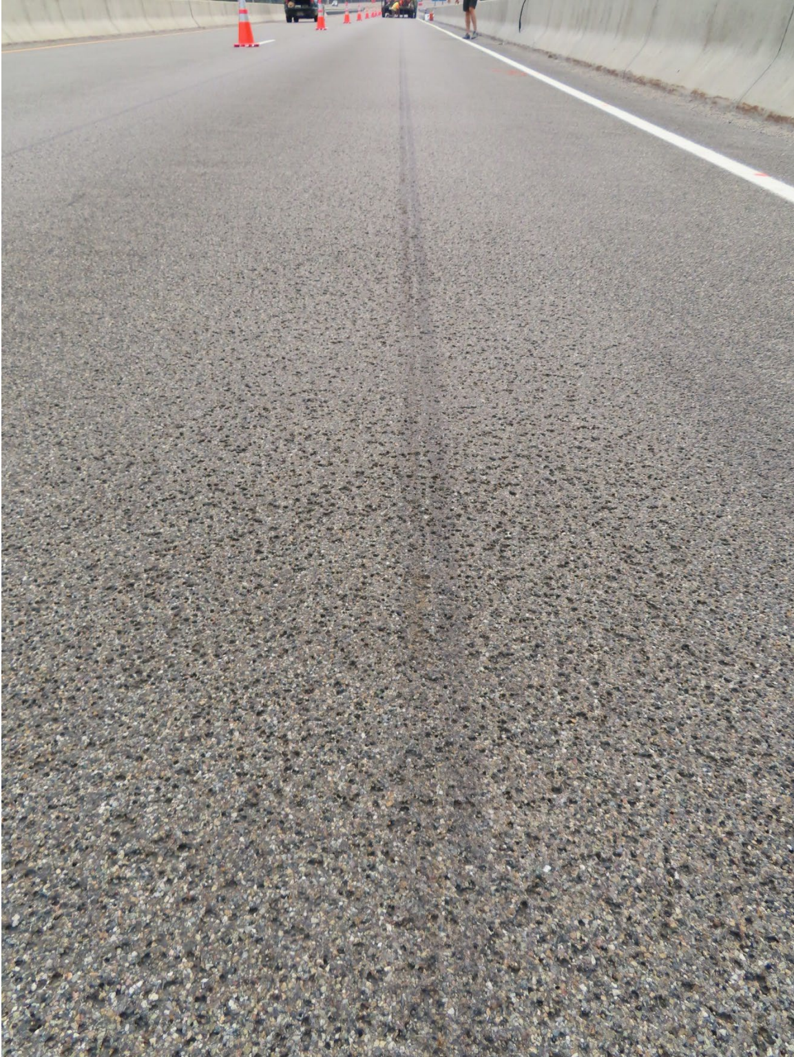
Figure 41. Photograph showing aggregate loss and polishing of the HFST in the driving lane of Bridge 1367 in 2020.
