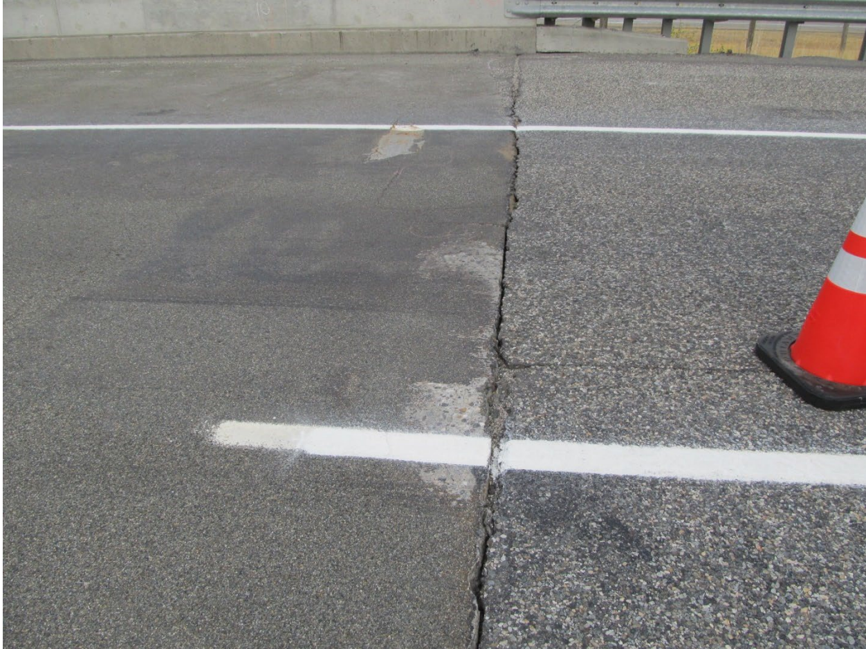
Figure 19. Photograph of snow plow damage and gouging at the entrance joint onto Bridge 1670 in the 2022 inspection.
