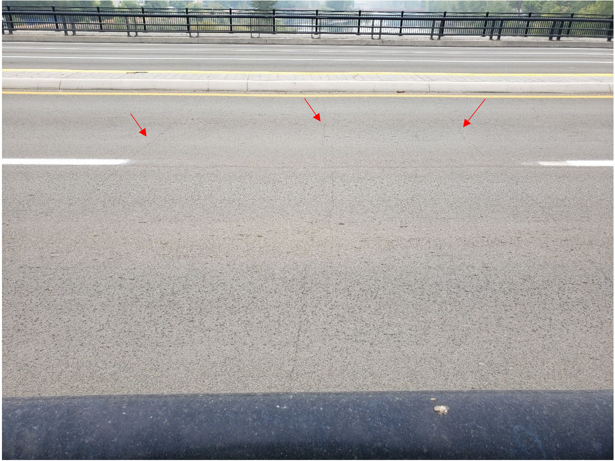
Figure 56. Photograph showing transverse cracking and wear of the SB lanes (foreground) on Bridge 25 in 2022. The NB lanes (Bridge 14) are in the background. Transverse cracks are identified with red arrows.
