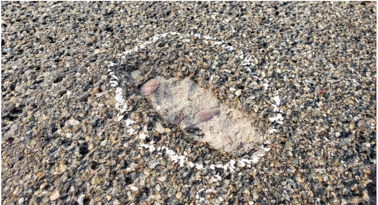
Figure 52. Close-up of small spall (gouge) in HFST of Bridge 1367 in 2022.
