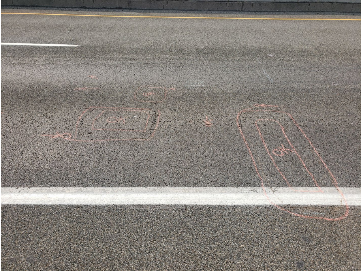
Figure 18. Photograph from 2022 inspection of Bridge 1670 showing delaminations around repair patches' edges that had reflective cracking previously. The centers of the patches remained sound.
