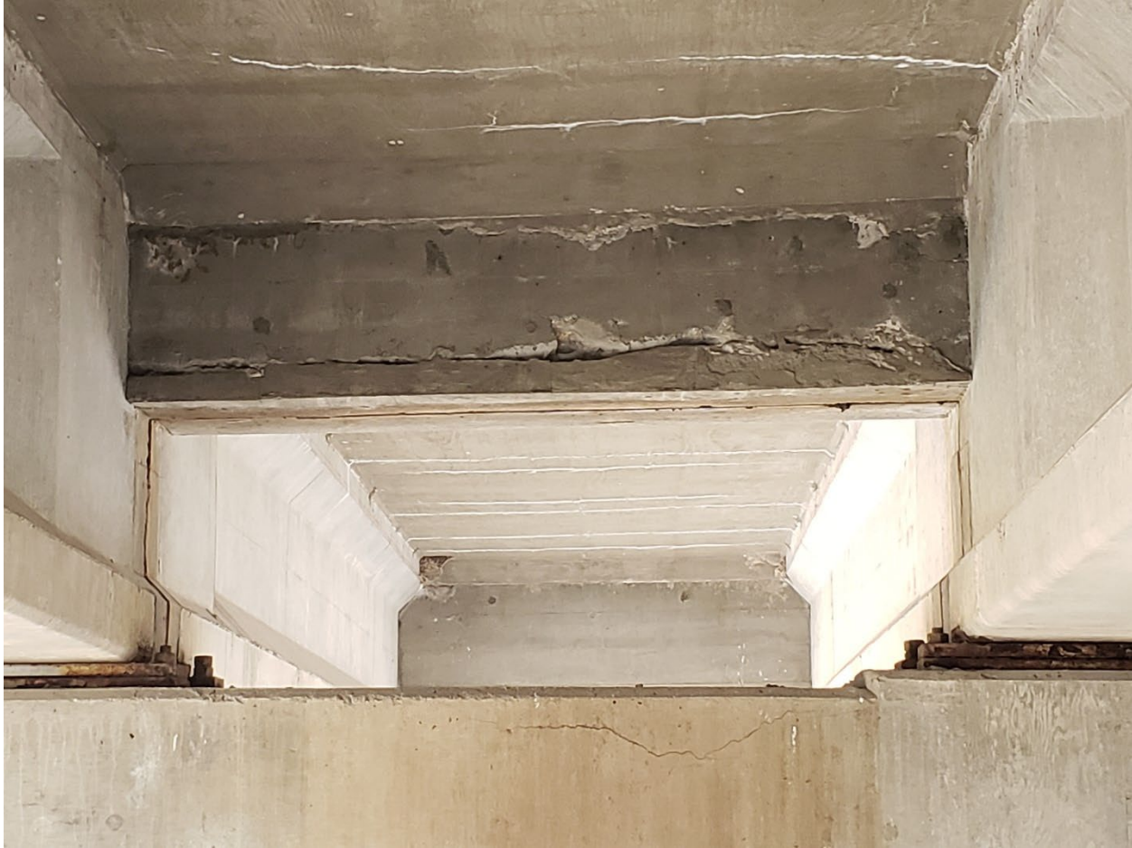
Figure 60. Cracks and spalls on the superstructure, deck beams, and pier cap of Bridge 1374 in 2022.
