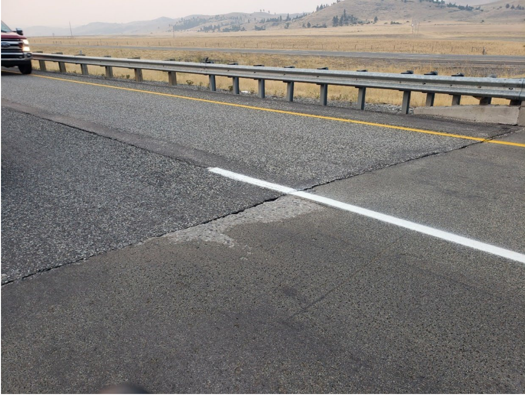
Figure 28. Area on leading edge of Bridge 1682 in 2022 where HFST was fully worn away.
