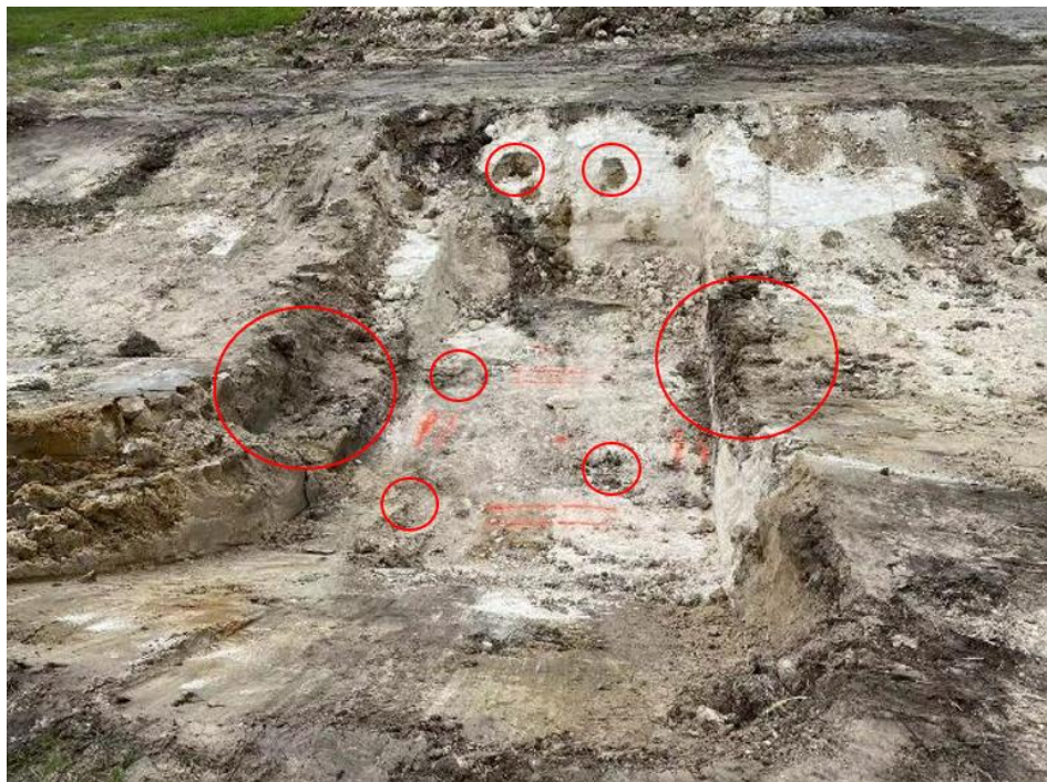
Figure 7-13. Footing location excavation (circles identify soil-filled voids)
