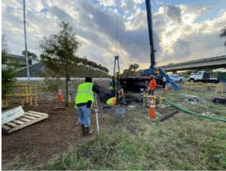
Figure 6-19 Measure the depth of the top of the threaded rods (2 ft from the ground surface) and align the drilled shafts
