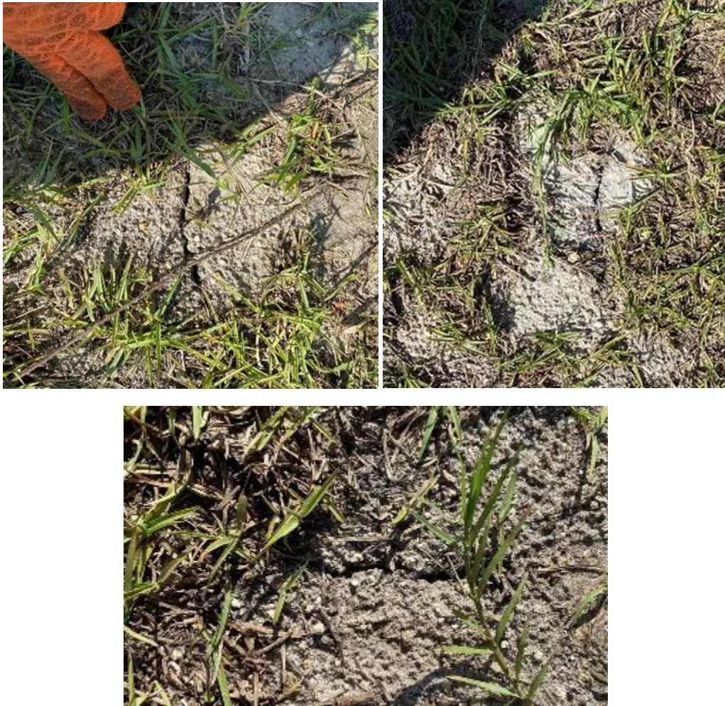
Figure 7-19 Tension cracks after load test
