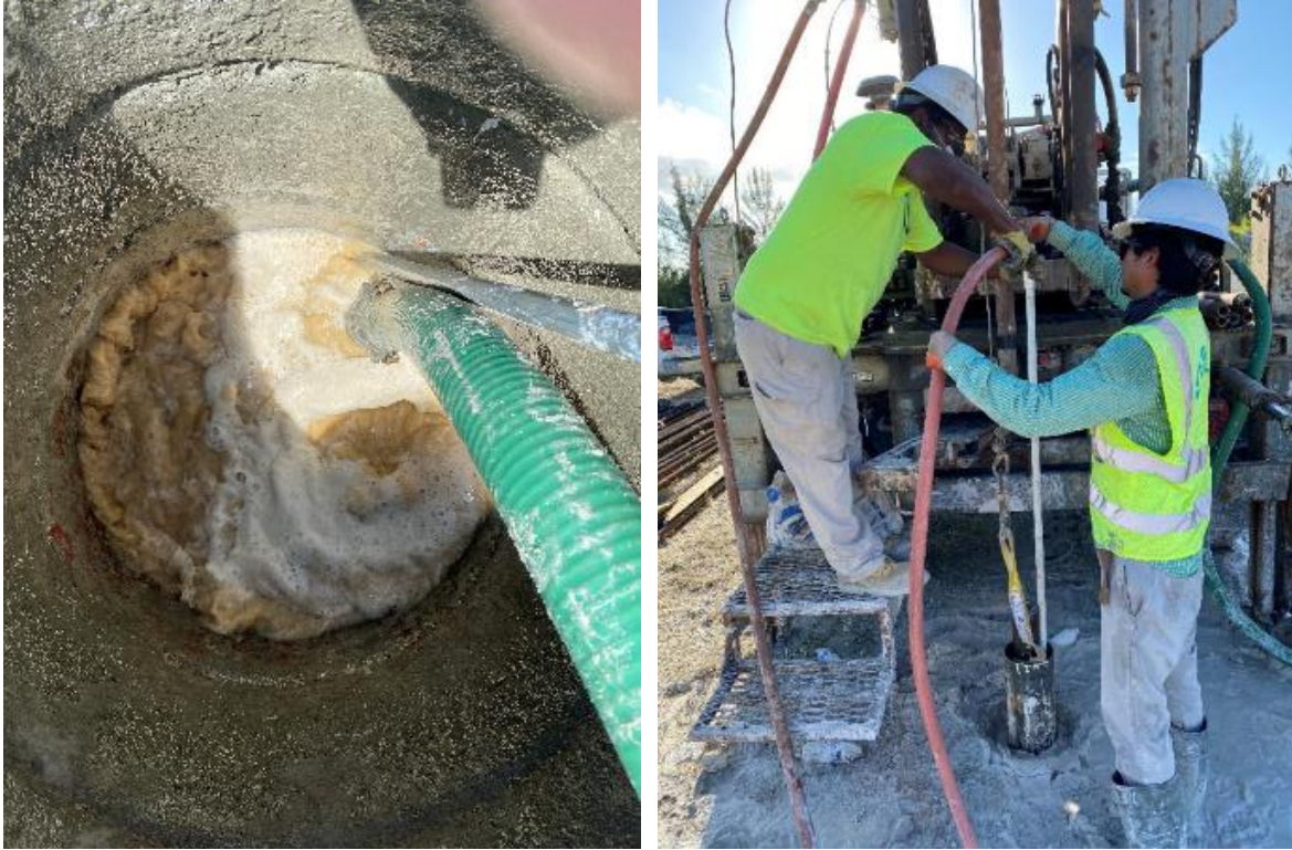
Figure 5-15 Grouting process (the grout mixed with ASTM C494 Type D retarder admixture and the ASTM C494 Type F superplasticizer admixture)
