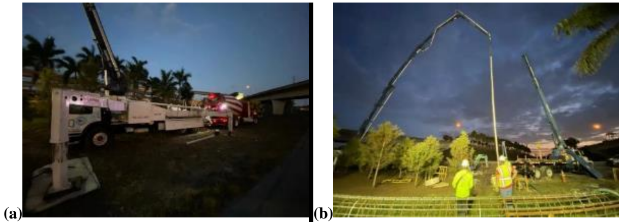
Figure 6-20 (a) mounted boom concrete pump truck and concrete truck; (b) delivery pipe and end hose
