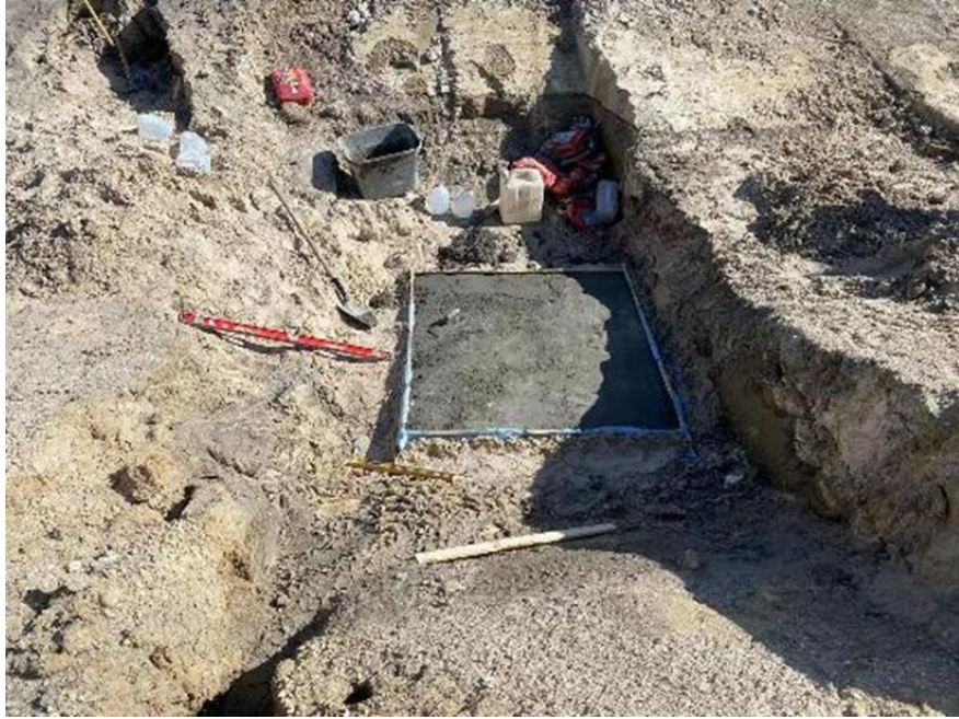
Figure 7-14. One in concrete leveling pad for placement of the steel foundation elements
