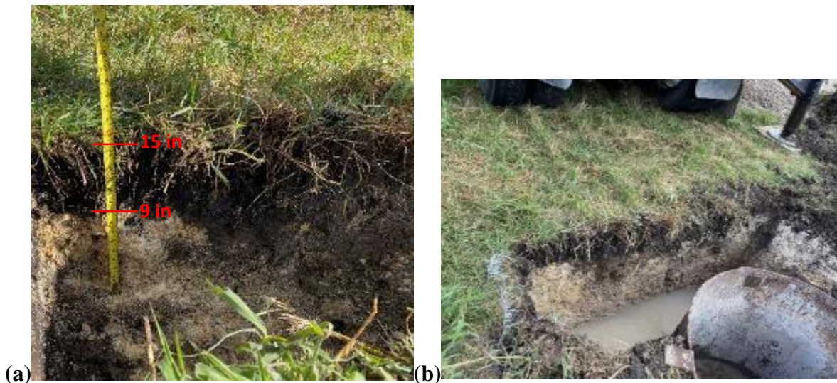
Figure 6-13 Miami limestone layer: (a) excavated down to 15 in; (b) excavated down to 3 ft.
