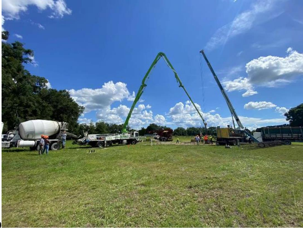
Figure 7-10. Construction of West shaft: (a) casing placement; (b) bailing bucket to clean the hole; (c) rebar cage installation; (d) installation of spacers for rebar cage and (e) concrete pumping
