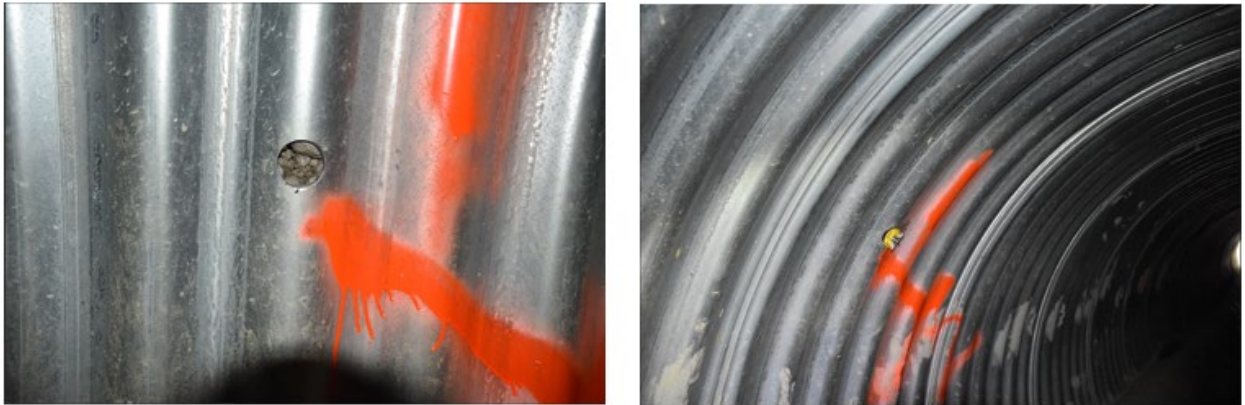
Loose limestone found at one culvert location.
