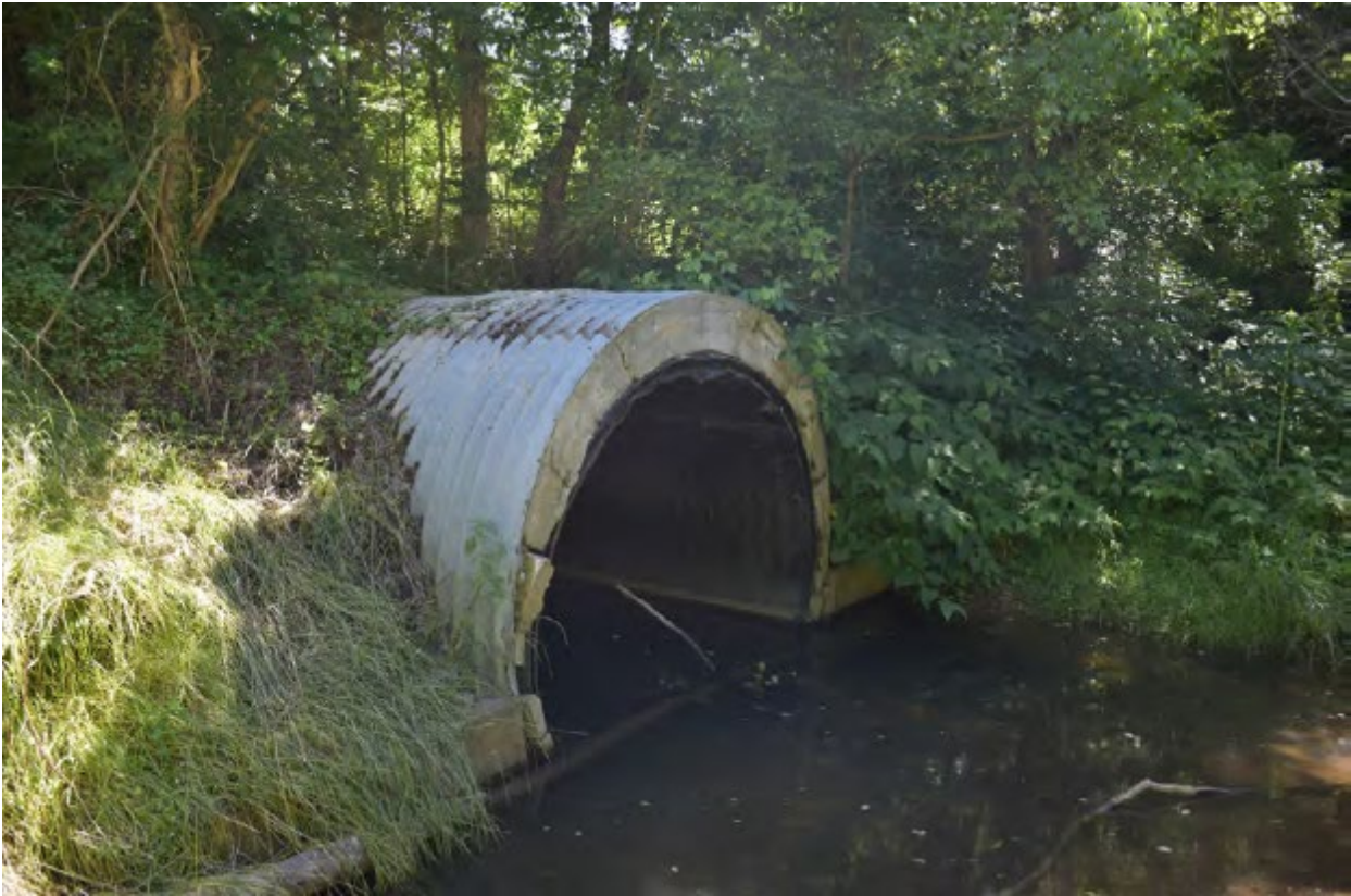
Culvert Access: High water level and unsafe access prevented inspection.
