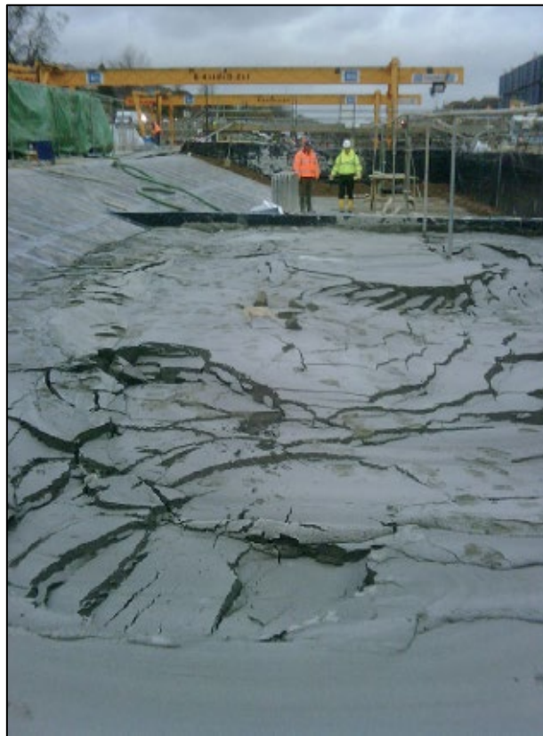
Figure E.10: Cellular Grout Instability on Site (Jones et al., 2016).
