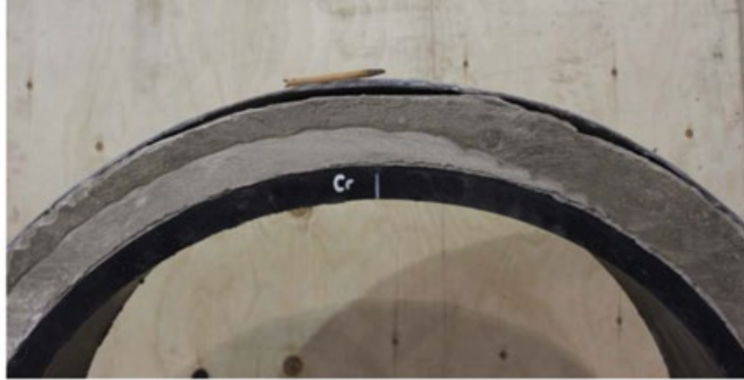
(a) Shrinkage of the high-strength grout in the rehabilitated specimen.
