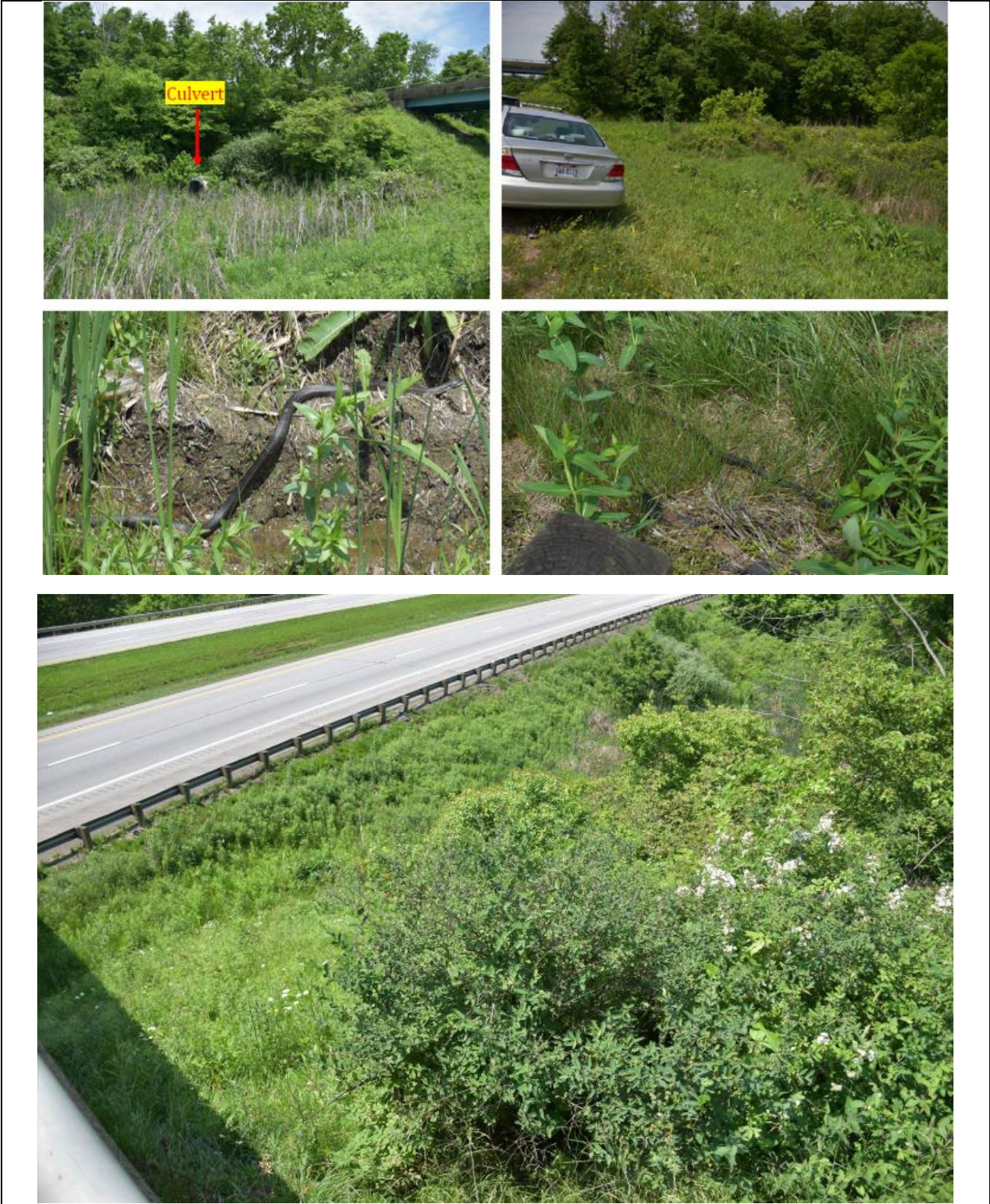
Marshy Land (Top), Snakes (Center). Inspection was Aborted due to safety concerns.
