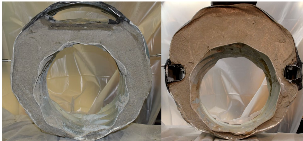
Figure F.24: Sliplined Culvert Specimens: One with a Void at Crown ( left ) and One with Two Voids at the Springline ( right ).
