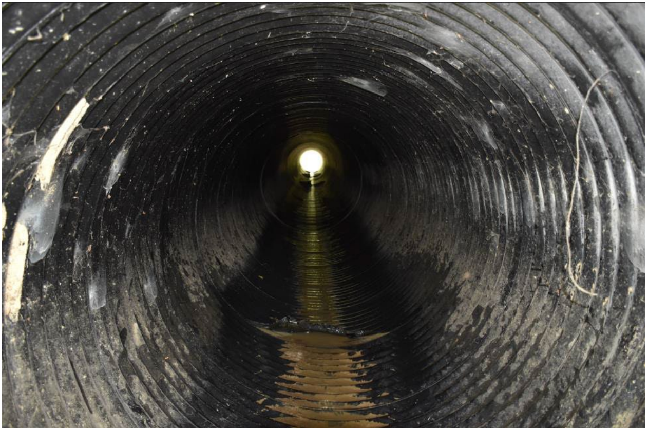
Culvert was made from corrugated steel pipe coated with bitumen (not sliplined) and exhibited tearing of the coatings at the joints.
