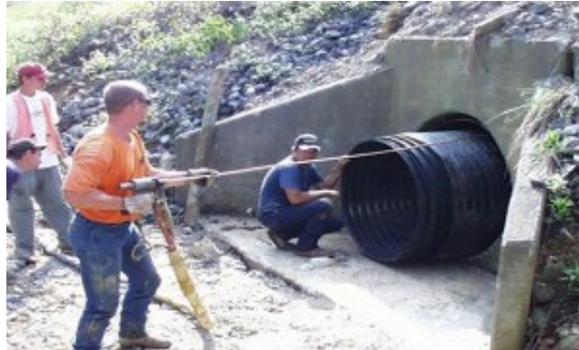
Figure A.12: URETEK team works to inject grout in between the pipes (Armstead 2015).
