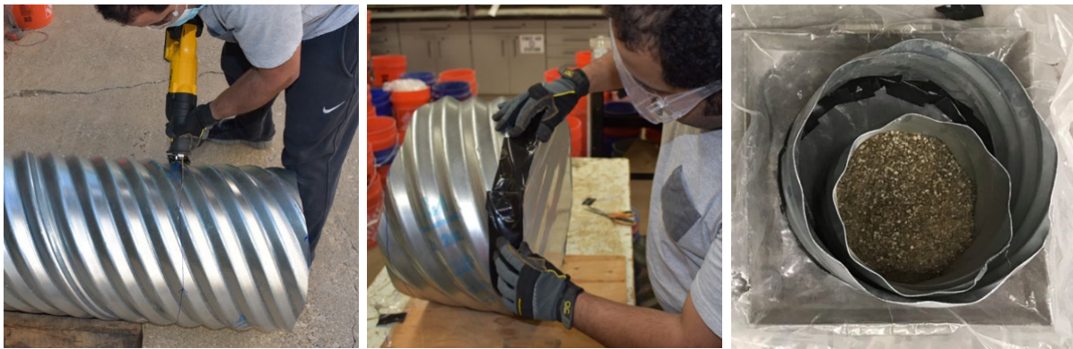
Figure F.20: Preparation of Host Pipe and Liner: Cutting the Liner Pipe ( left ), Wrapping the Bottom of Host Pipe with Plastic ( center ). Liner Pipe Packed with Sand ( right ).
