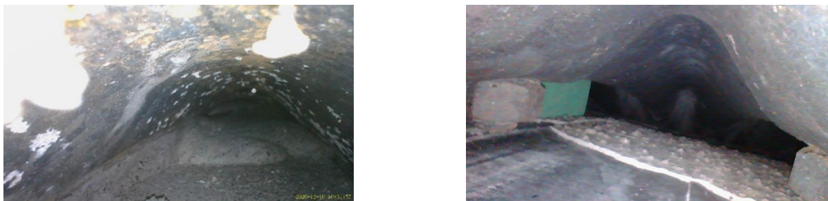
Figure 4: Images Showing Examples of Partially Filled Annulus Voids.
