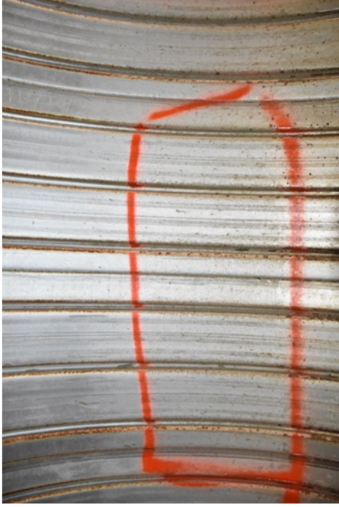
(b) Marking the Location of a Suspected Void with Orange Paint
