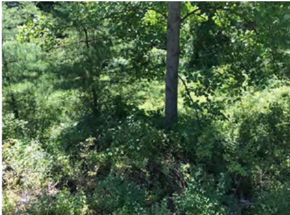
Culvert Access: Vegetation made it difficult and unsafe to access either side of the culvert.
