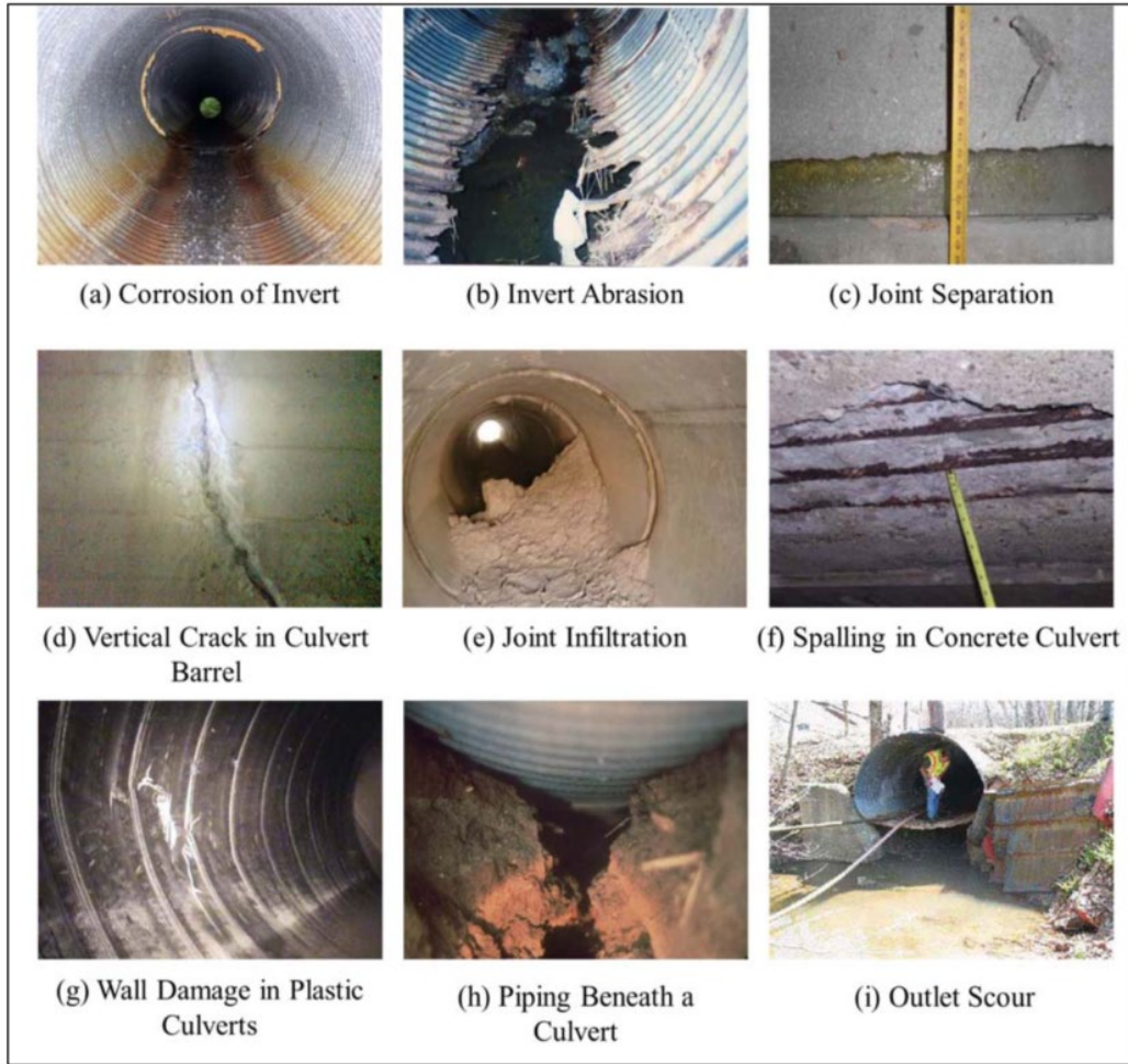
Figure A.68: Common defects observed in culverts (Piratla et al. 2017).
