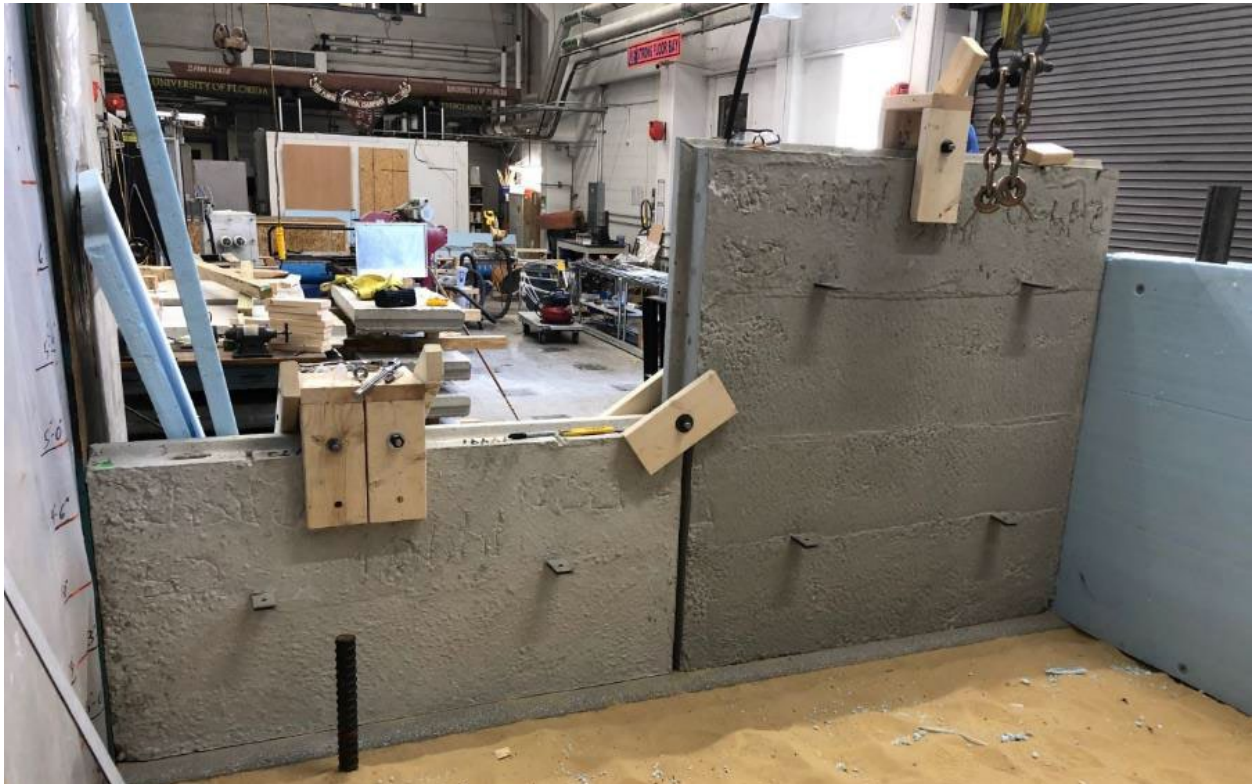
Figure 4-20. Front MSE wall prior to the first lift above the base layer.
