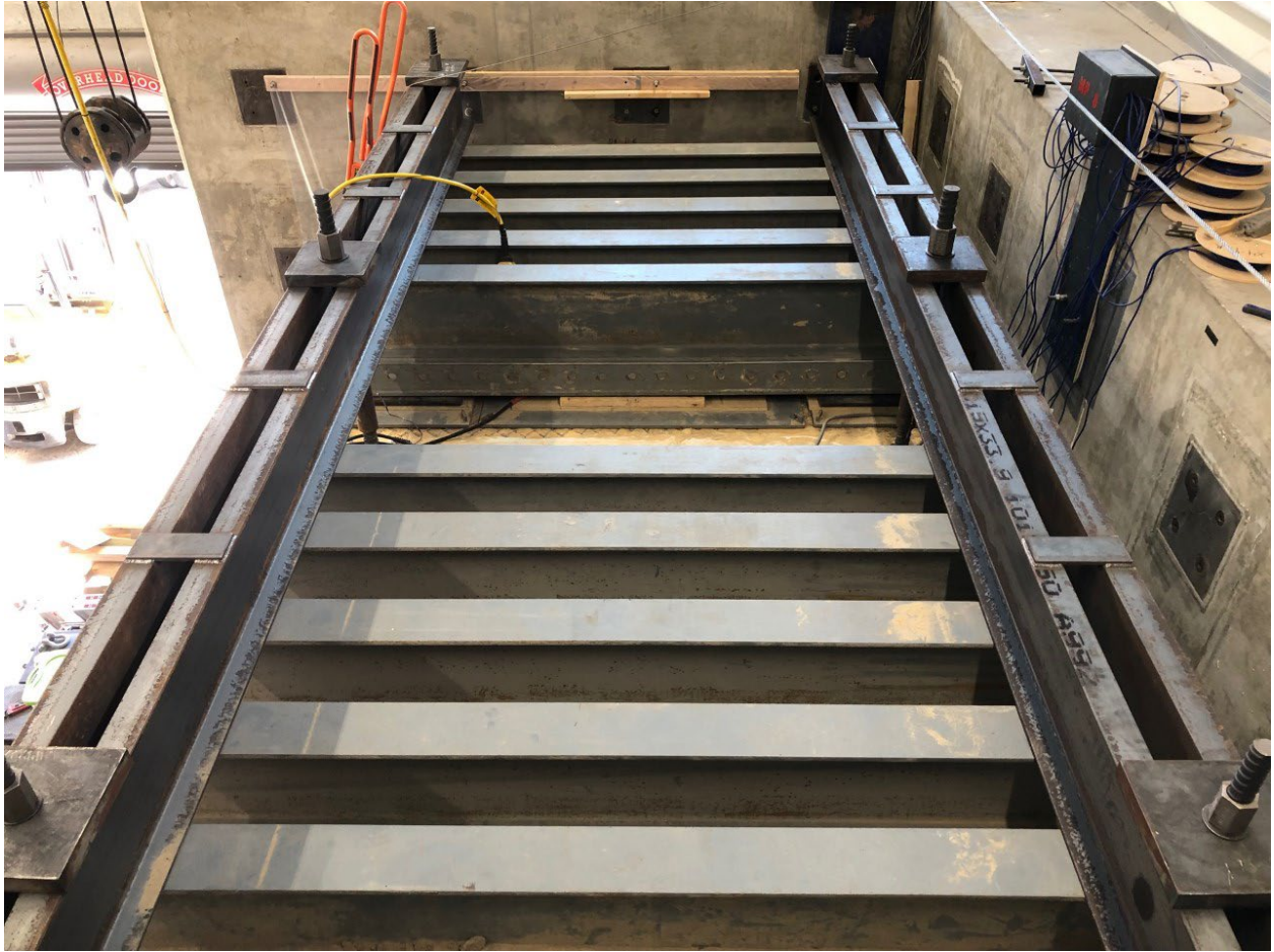
Figure 4-38. C-channels added and secured in place to complete the matjack reaction frame.
