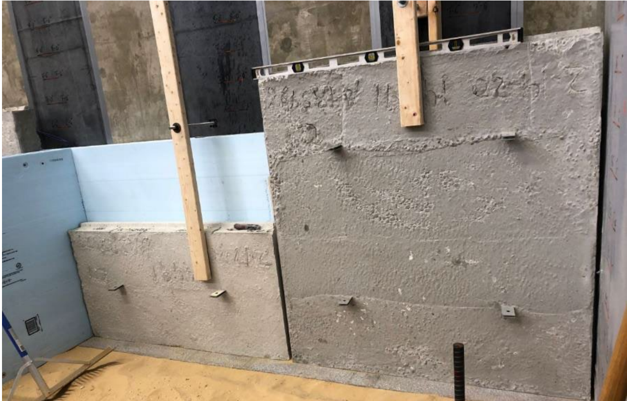
Figure 4-19. Back MSE wall prior to the first lift above the base layer.
