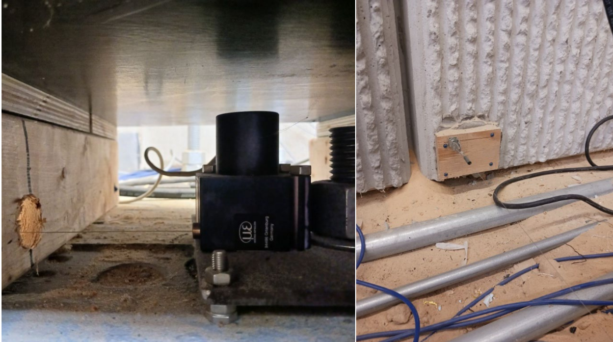
Figure 4-53. Draw wire sensor attached to base MSE wall panel to measure wall movement.
