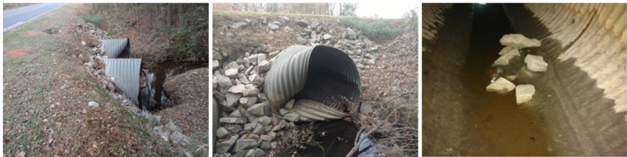
Figure 30. Photos of damage after Hurricane Matthew in Site 95-3-M.
