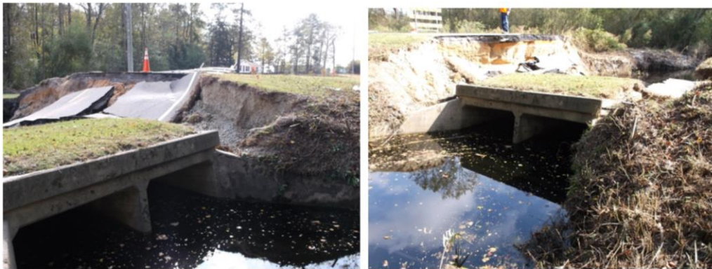
Figure 19. Photos of damage after Hurricane Matthew in Site 95-4-MF.
