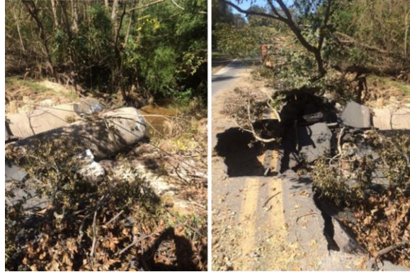
Figure 27. Photos of damage after Hurricane Matthew in Site 53-4-MF.
