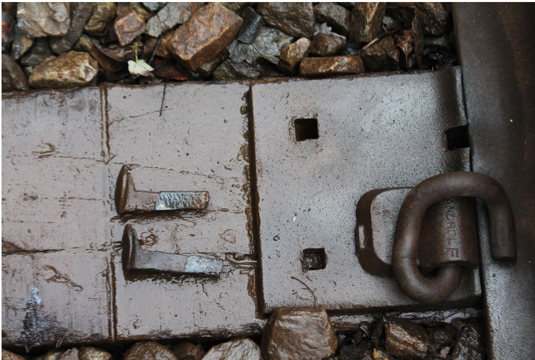
Figure 46. Two broken spikes in a Victor plate on a new crosstie
