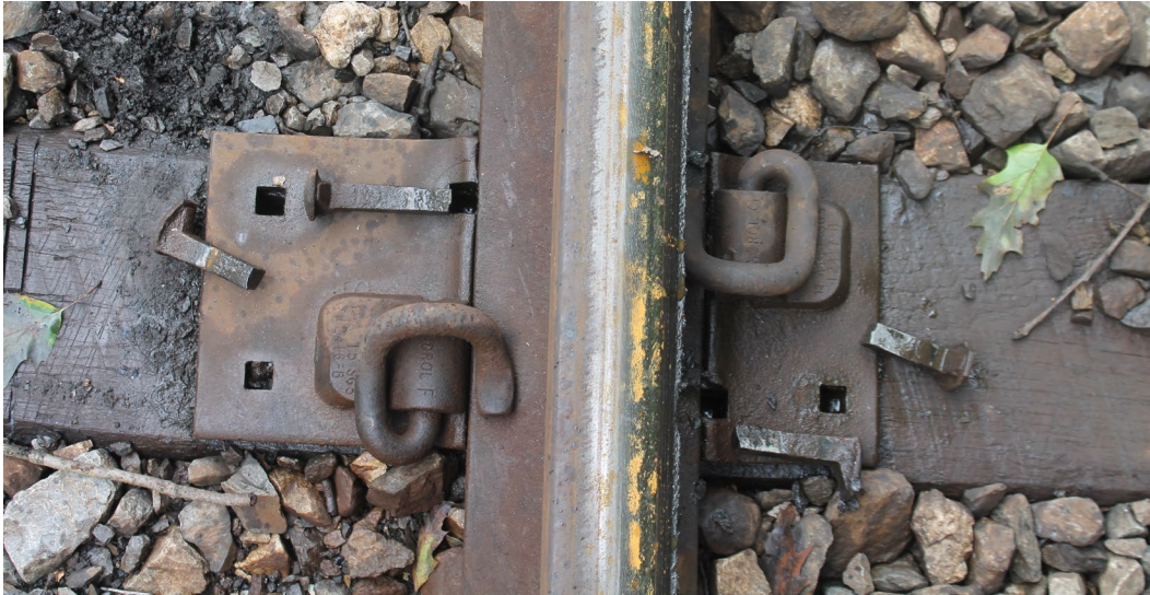
Figure 44. Four broken spikes removed from a Victor plate in the low rail
