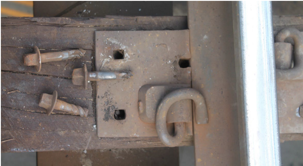
Figure 39. Three broken spikes removed from a bridge timber. The fact that these are drive spikes signifies that all three spike holes previously had cut spikes that broke
