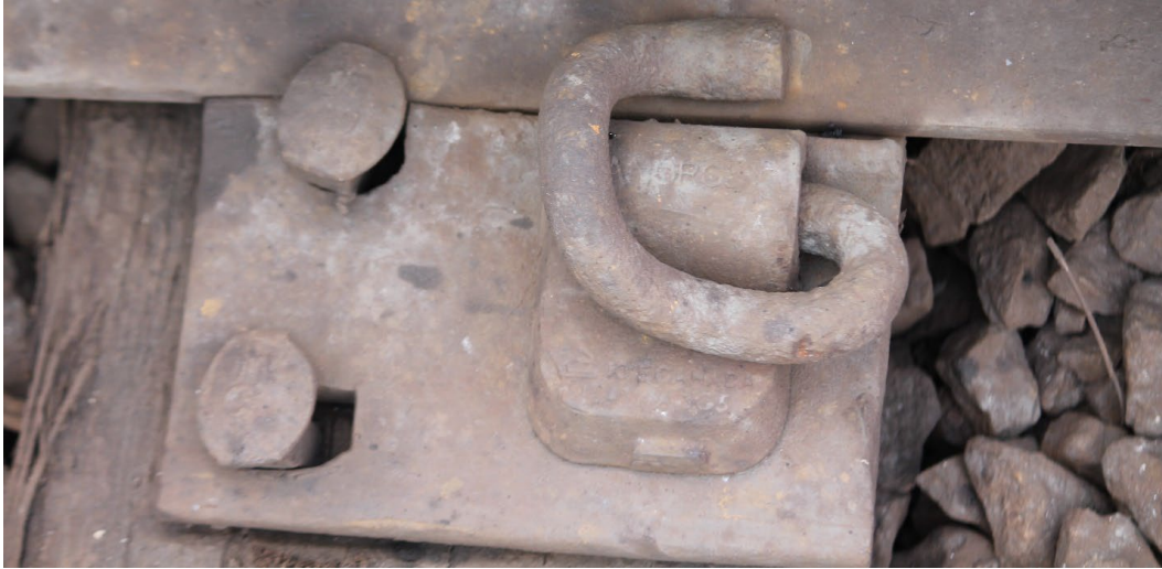
Figure 41. Spike hole and shoulder wear indicates plate rotation and severe contact between plate and spike
