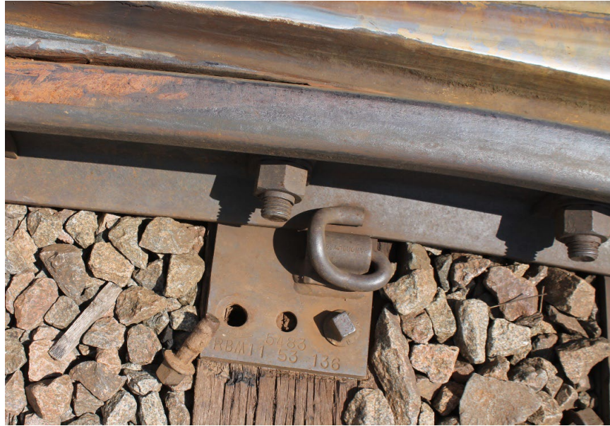
Figure 33. Broken spike around the frog of a turnout
