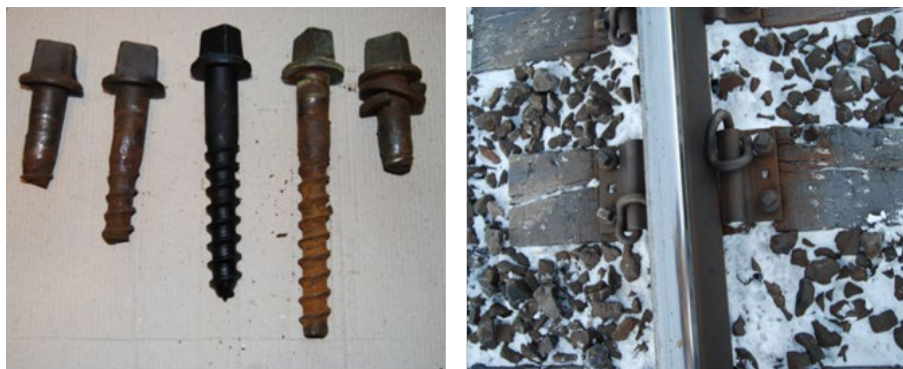
Figure 4. Broken screw spikes (left) and rolled plates (right) [3]
