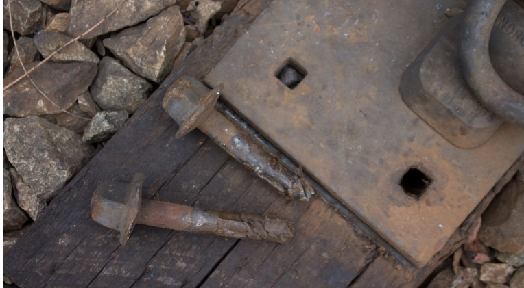
Figure 26. Broken drive spikes in repeat-breakage locations
