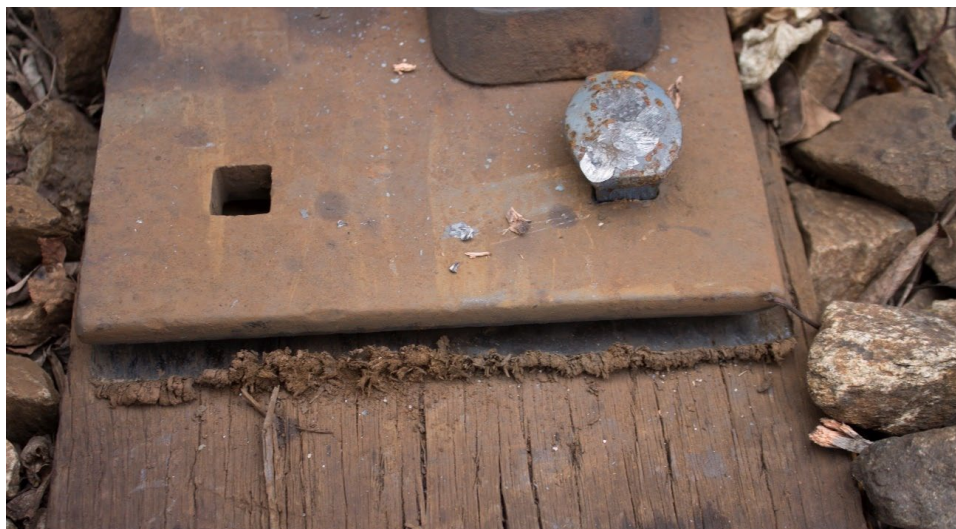
Figure 23. Plate cut/shove suggesting possible broken spikes
