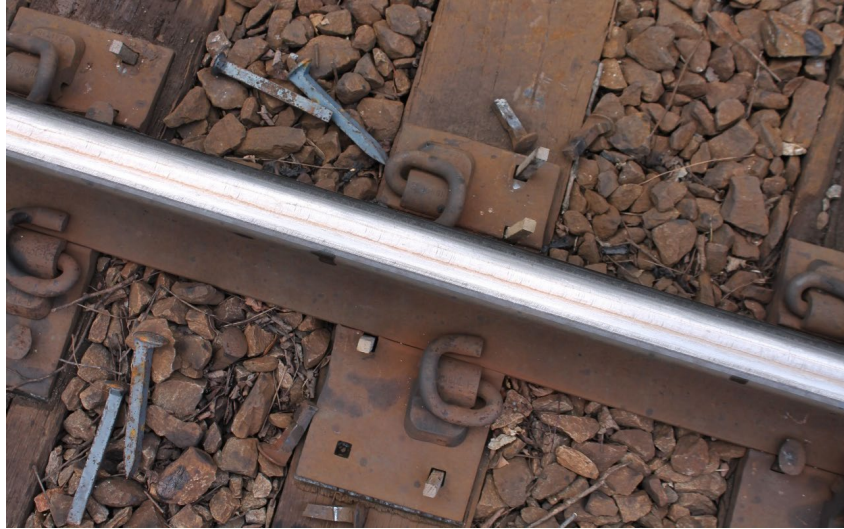
Figure 29. Plug wood and new spikes to be installed in a plate where all four spikes broke.
