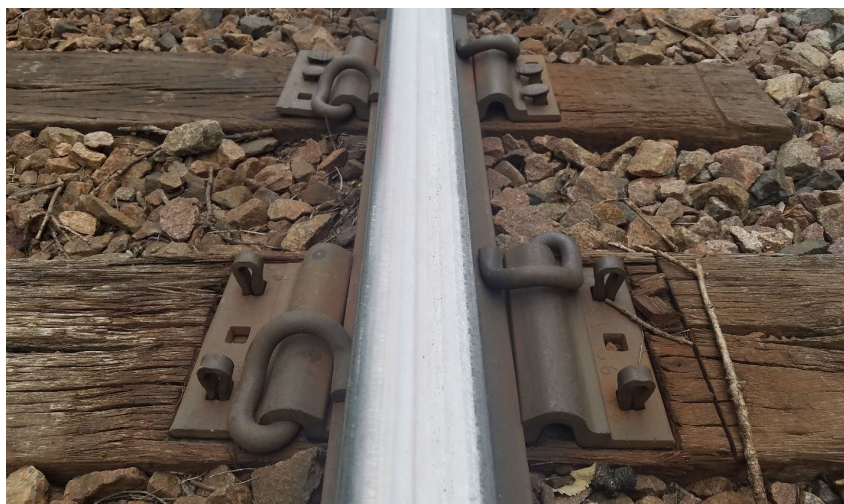
Figure 30. Pandrol plates using lock spikes (foreground) and cut spikes (background)
