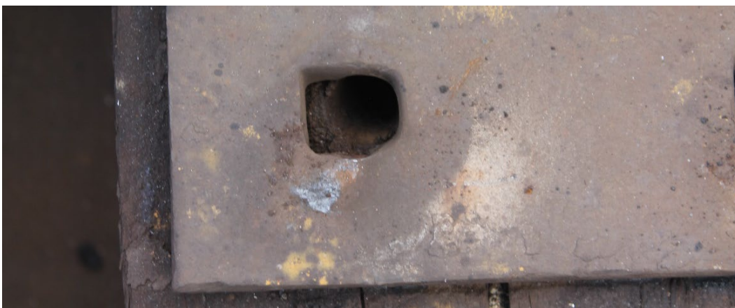
Figure 40. A spike hole with broken spike removed reveals that the spike was in a severe contact position with the plate. Spike hole wear is indicative of longitudinal plate movement to the left
