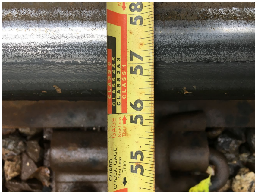
Figure 48. Slight tight gage found at one broken spike cluster
