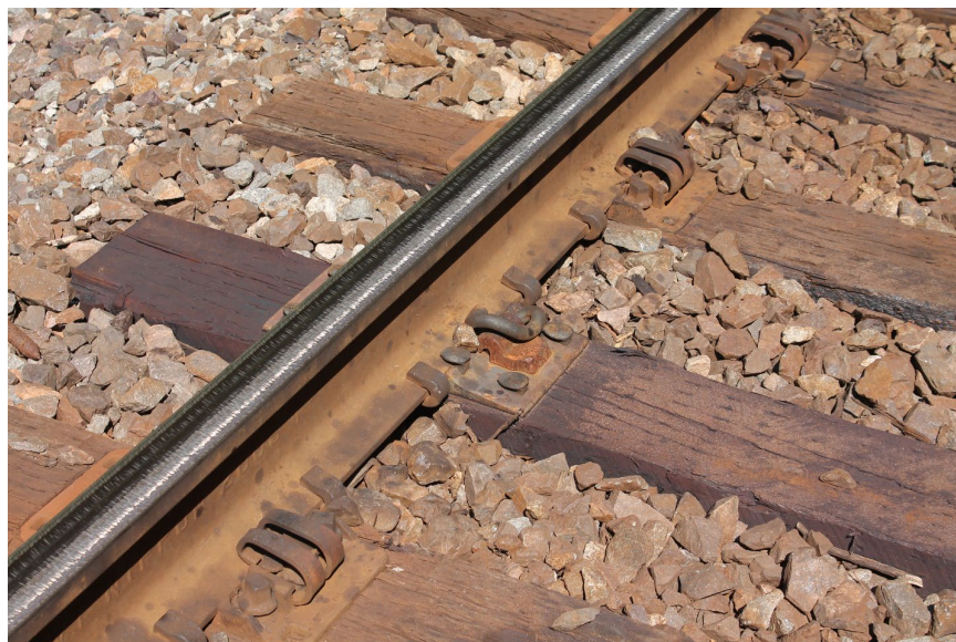
Figure 37. A new crosstie with Victor plate, spotted in where there was previously a crosstie with broken lags in the McKay system
