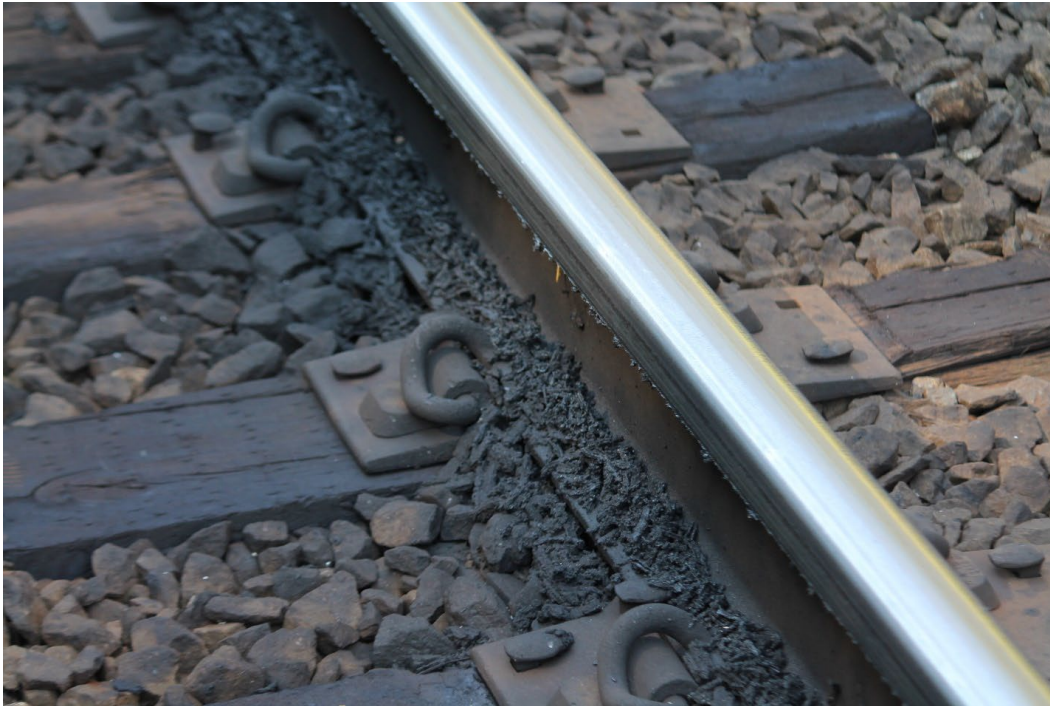
Figure 43. Curve grease build-up at Conemaugh, PA
