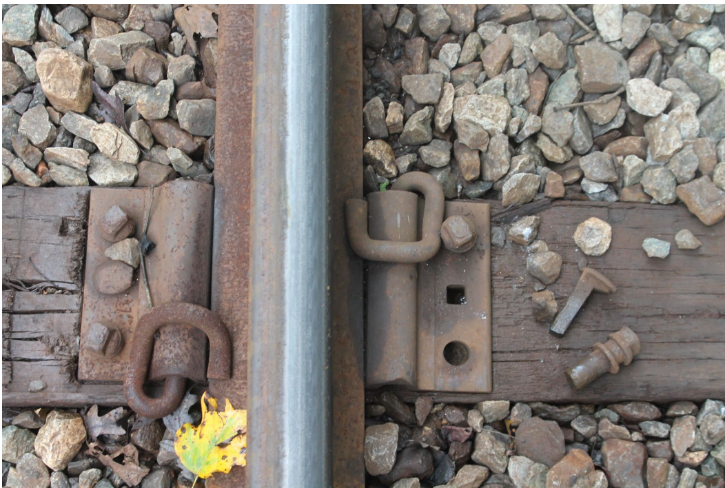
Figure 45. A broken Evergrip and a broken cut spike found in a Pandrol plate on the high rail at the second curve
