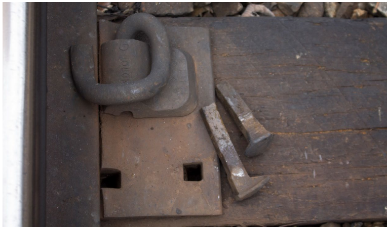
Figure 24. Typical broken spikes after removal
