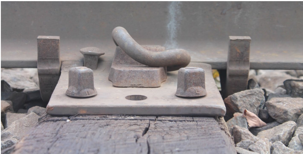
Figure 42. New crosstie with "bridge Victors" and rail anchors to help alleviate spike failures
