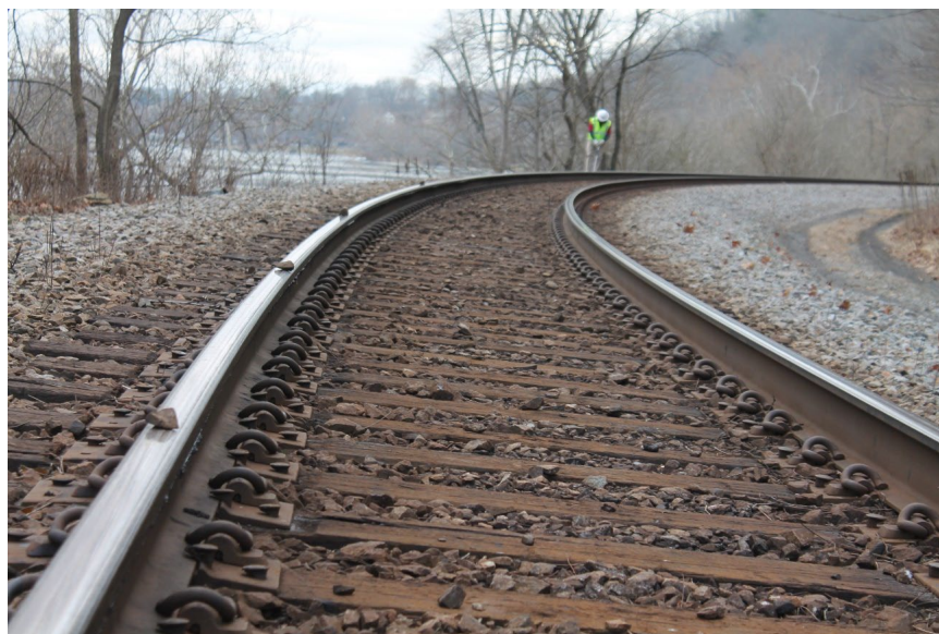
Figure 28. Broken spike clusters appearing at certain intervals, marked by ballast particles on the rail. Note the curve grease marks on the high rail gauge face.
