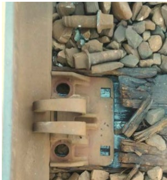
Figure 6. Broken lag bolts at the Mosier derailment site [6]
