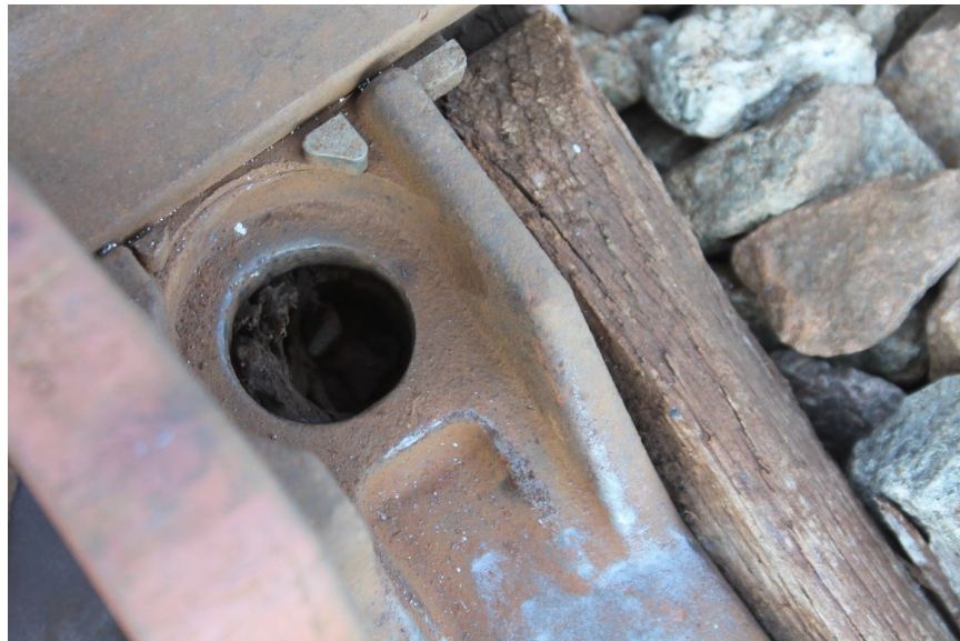
Figure 36. Timber visible in the spike hole, possibly suggesting plate movement and/or severe contact of the plate and spike
