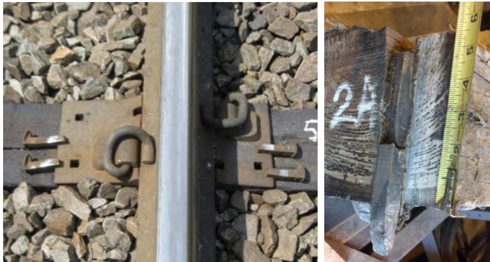
Figure 5. Broken spikes (left) and rail seat cross-section (right) [4]
