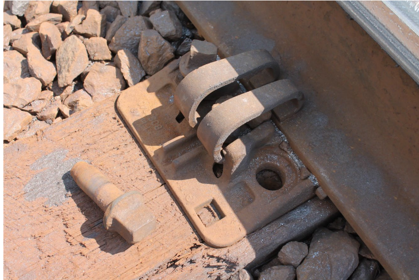
Figure 35. Broken lag screw removed from cast plate, typical of failures observed
