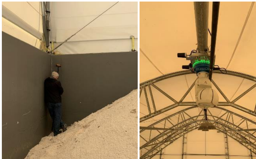
Figure 6.5. Measuring the Salt Shed with the Carlson BRx7 GPS receiver and RT4 Data collector.
