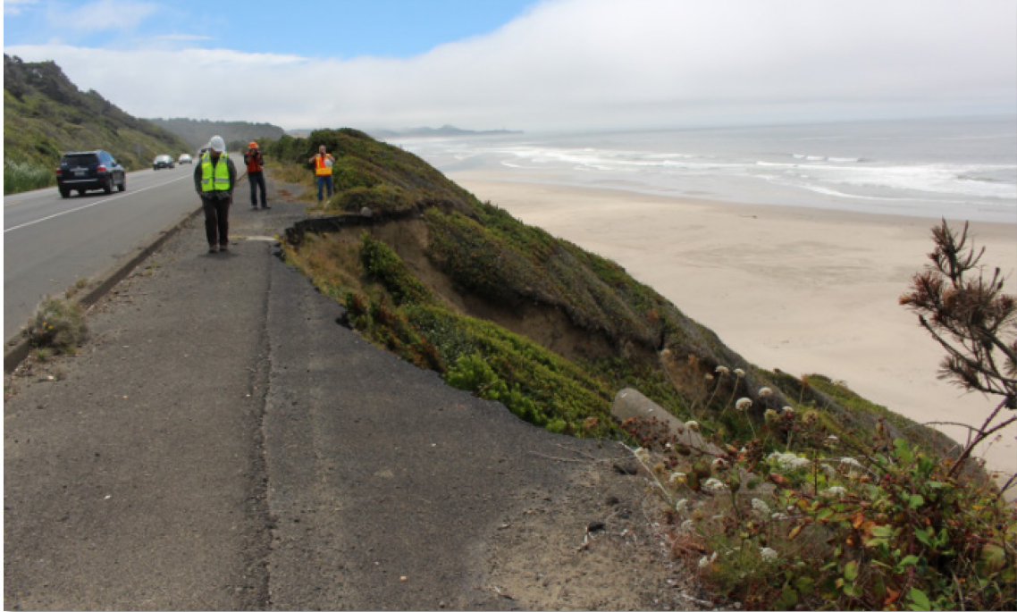
Figure 7.15: Mass movement and infrastructure damage along Hwy 101 at Spencer Creek, (facing south, near MP 134, August 2016).
