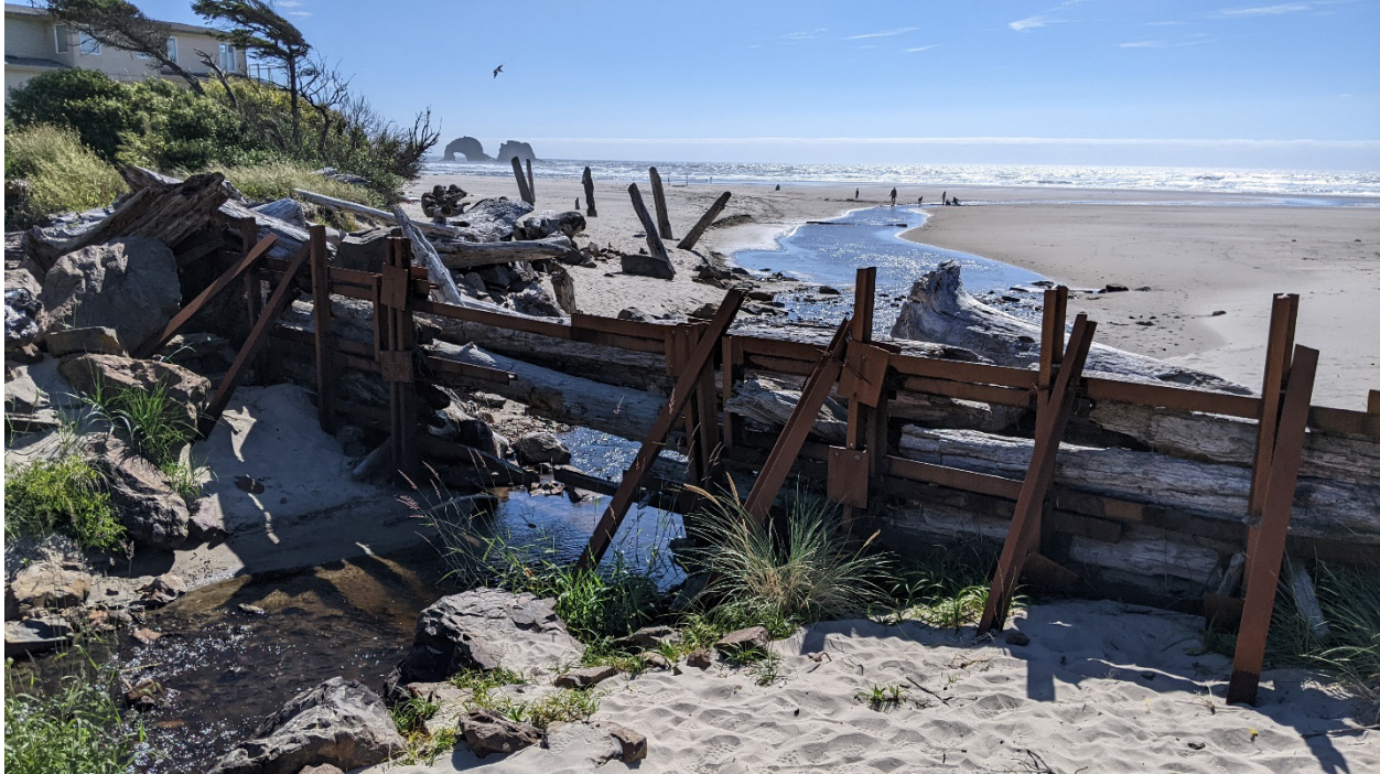
Figure 7.13: Photograph showing the driftwood protection wall with steel railroad track supports (July 2022).
