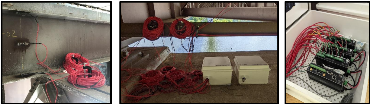
Figure 3-8. Cabling and DAQ Connection
