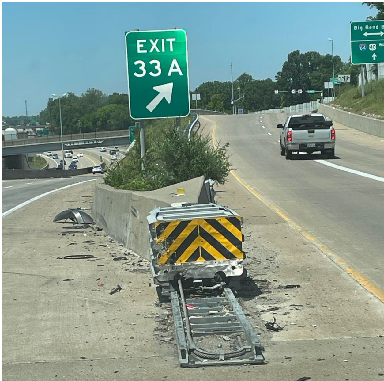
Figure 4. WB I-64 Exit to Big Bend Boulevard Crash Barrier Impact
