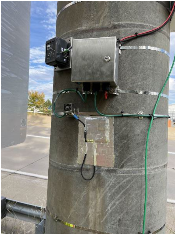
Figure 21. SB 141 at MO 100 – Strain Gauge and Node Installation
