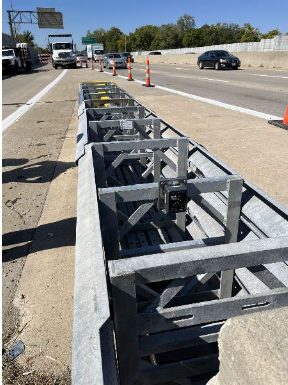
Figure 24. I-64 WB Exit Gore to Big Bend Boulevard – Accelerometer Installation
